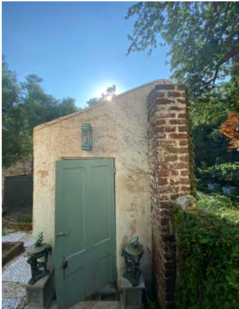
Tool Shed (door rotted)
