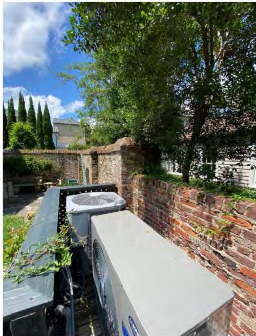
HVAC Platform (existing)
