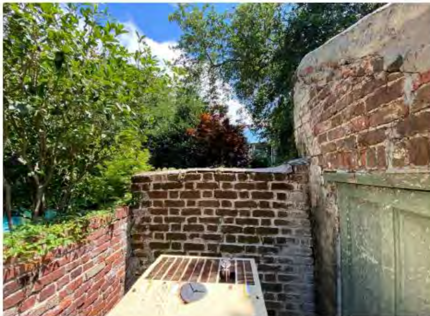
Generator Platform behind Tool Shed (existing)
