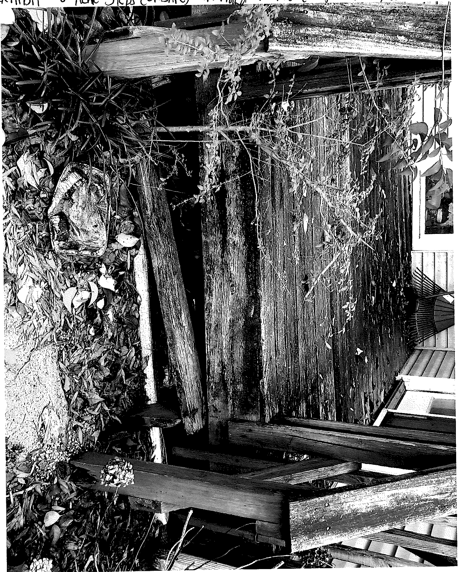
Exhibit #8 Rear Steps (UNSAFE) Provided To The Court JAN 6, 2022
