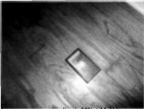
Moisture meter max reading is 32% + Mold begins growth at 17%
