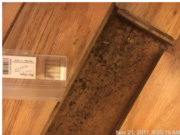
Under the flooring in the 1 st floor bathroom.
