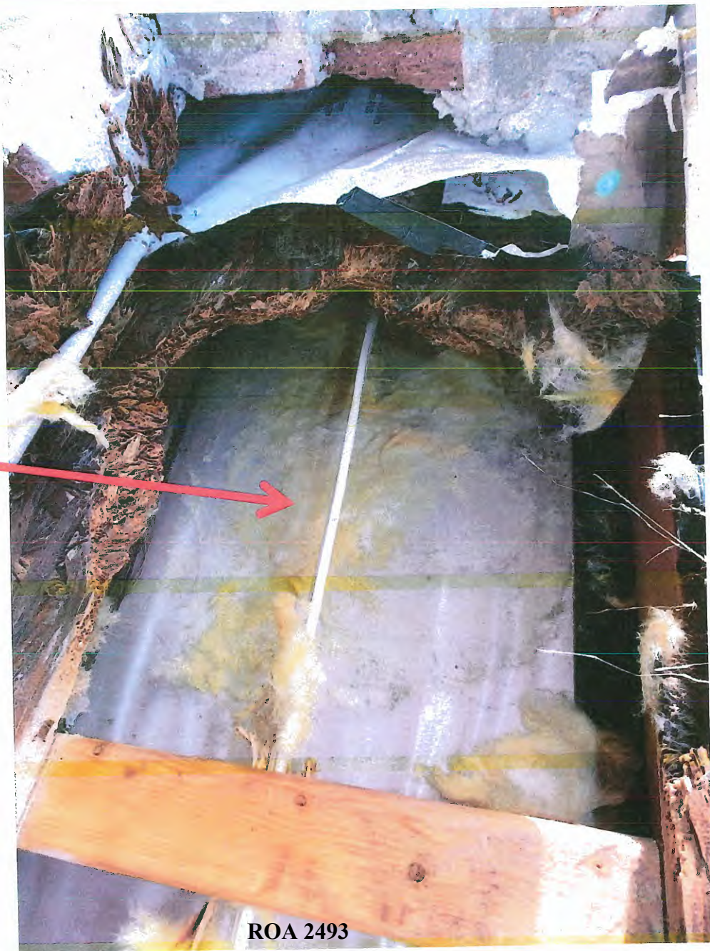
INSULATION ADHERED TO VAPOR BARRIER DUE TO MOISTURE ACCUMULATION
