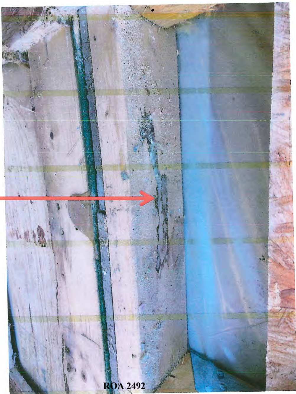
EVIDENCE OF MOISTURE ACCUMULATION WITHIN WALL CAVITY
