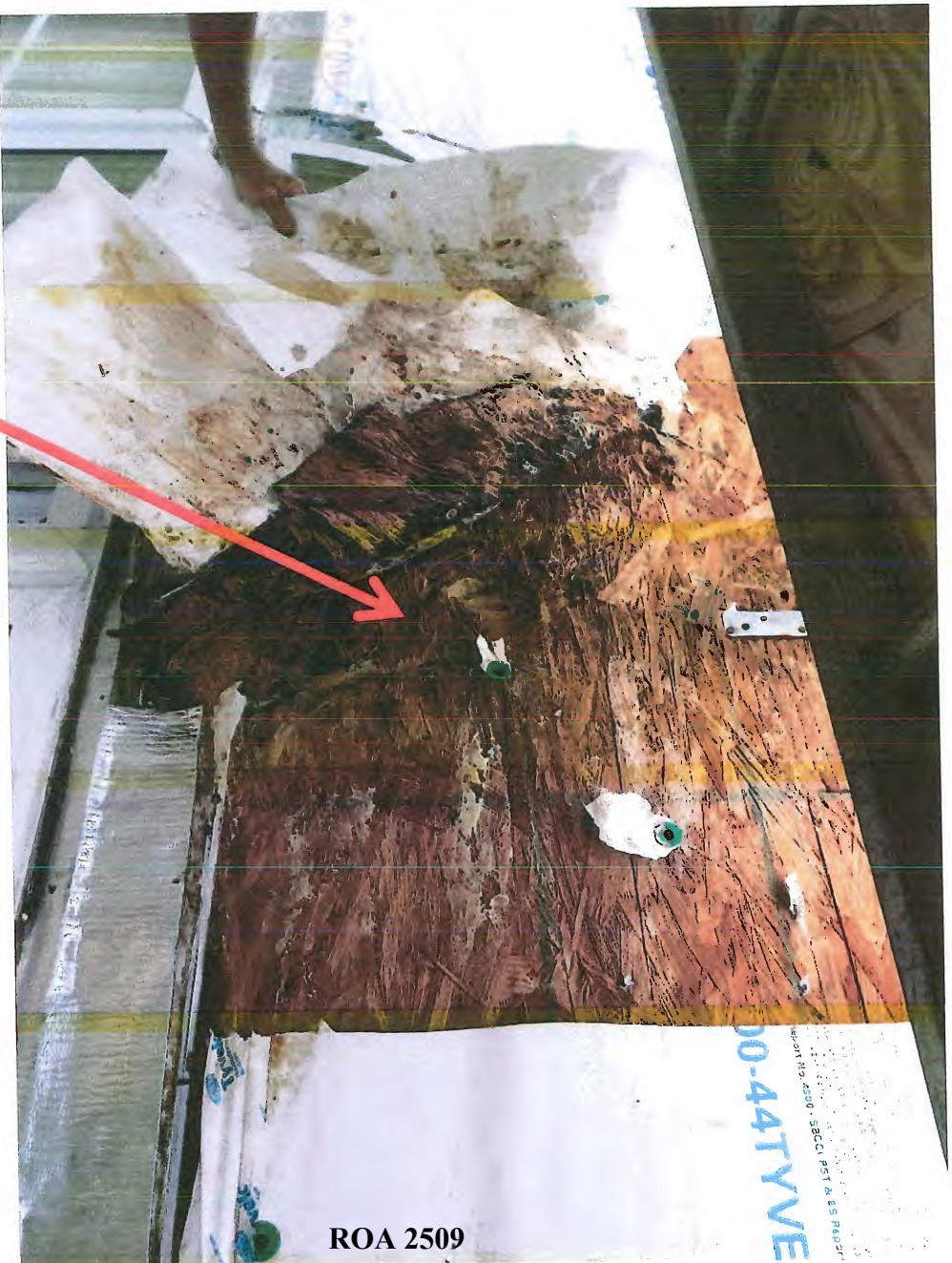
ROTTED WOOD SHEATHING
