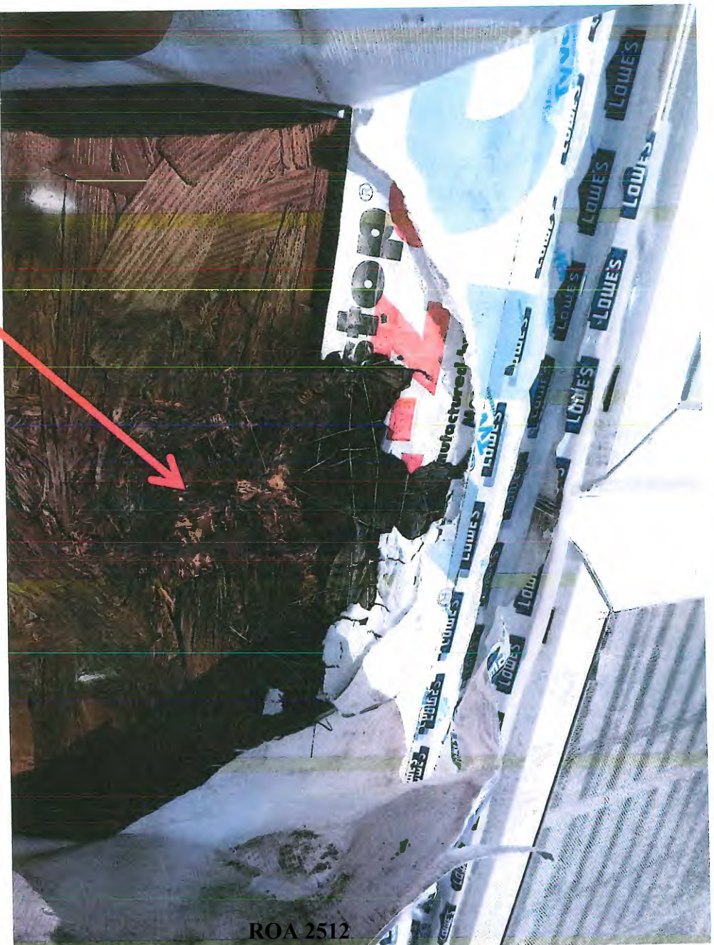
ROTTED WOOD SHEATHING
