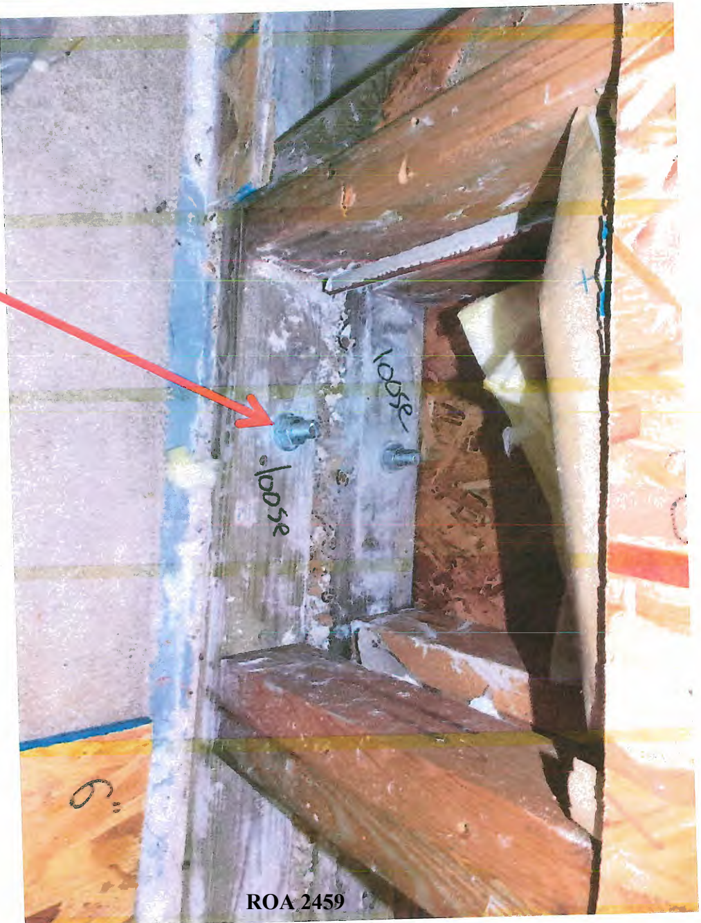
LOOSE ANCHOR BOLT NUTS
