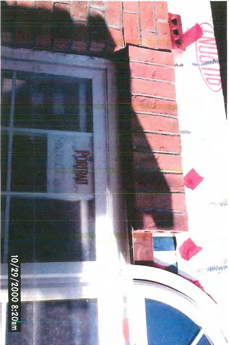
WW-07 Short Lintel Over Window Unsupported at Center ..... 142 of 147
