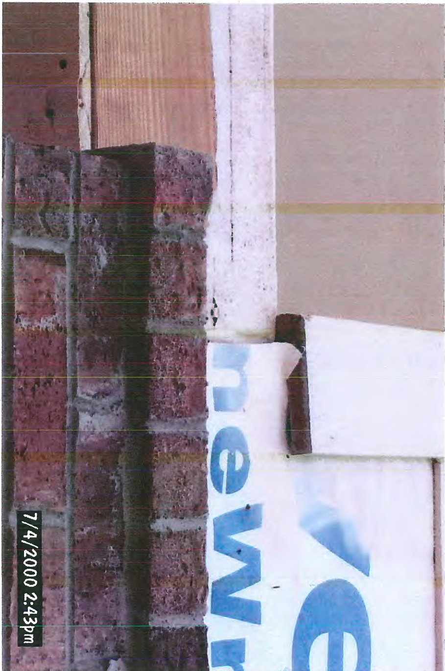
WW-02 (Pad 6) Raw Edge Trim Board near Rowlock (Wicking Risk) ..... 7 of 90
