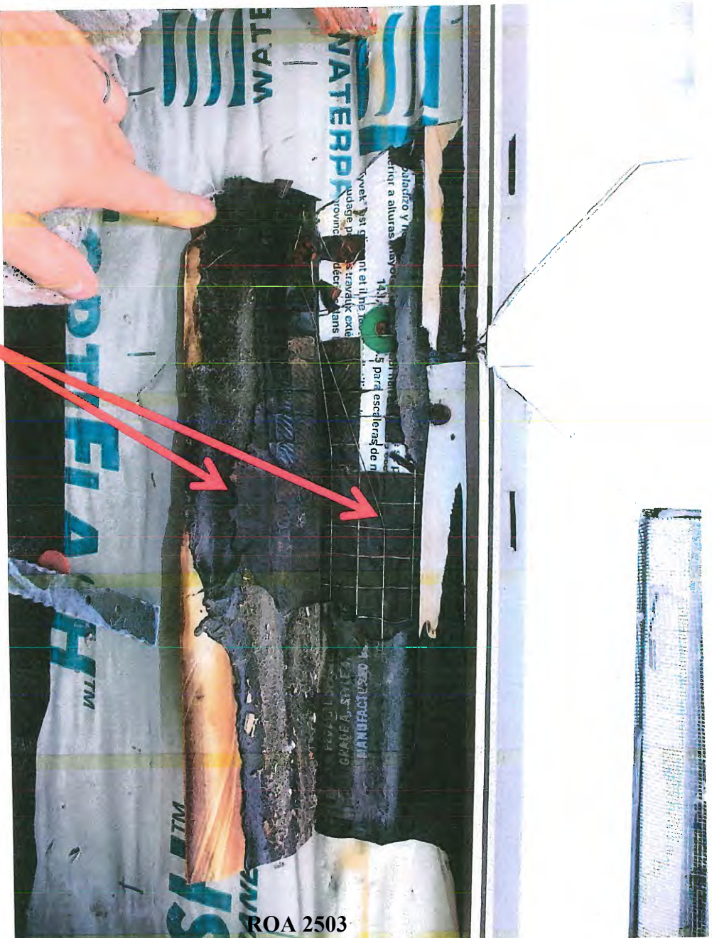
DEFECTIVE FLASHING- FALLING APART
