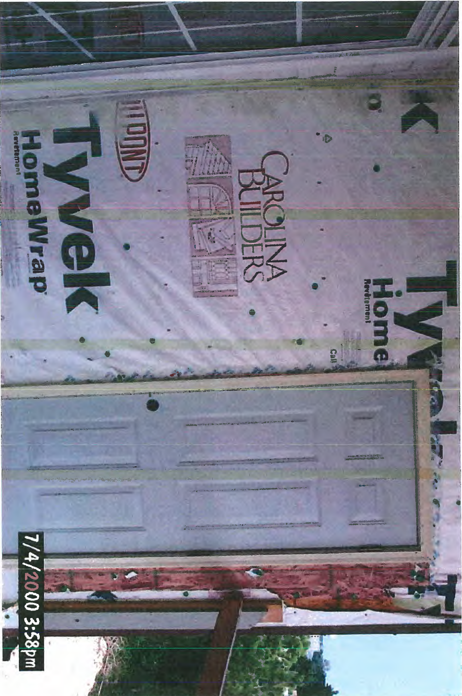
WW-02 Unit 3-2 Tyvek™ System Breached at Balcony ..... 20 of 90
