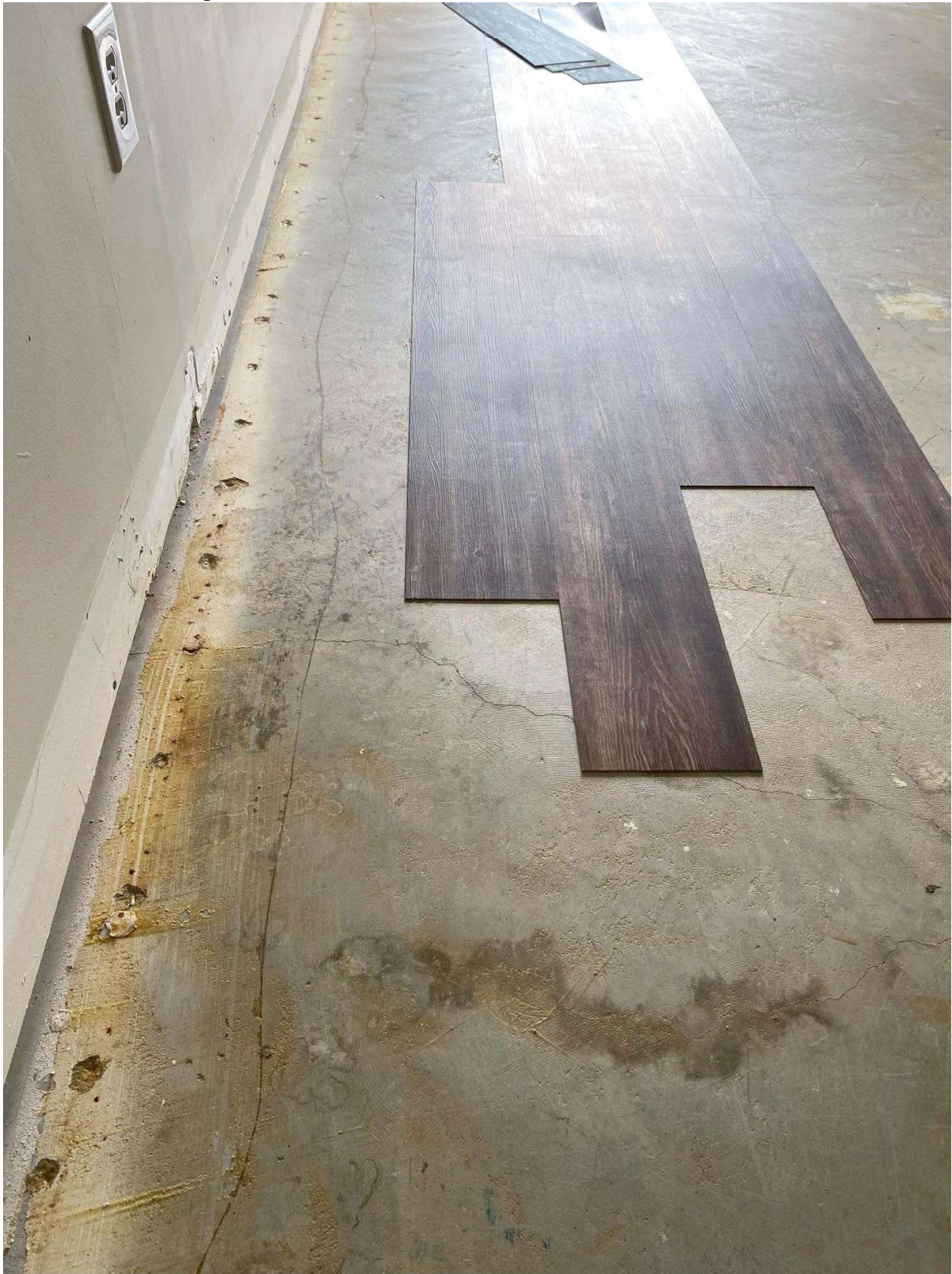
Picture 38: Sub-floor cracks, holes, and deviations not appropriately prepped. Porous substrate absorbed glue
