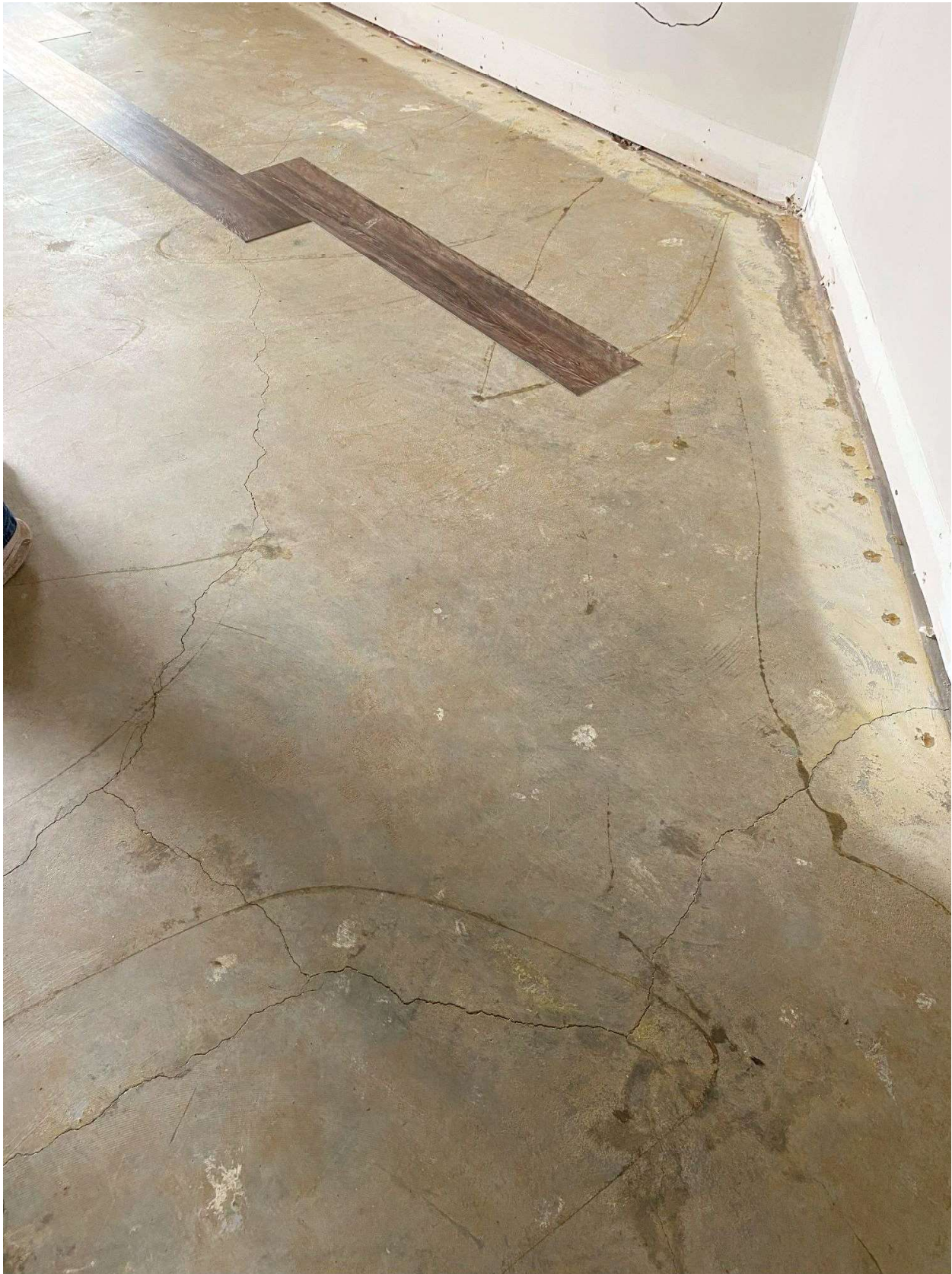
Picture 34: Substrate not smooth, free of old paint and old adhesive. Products not rolled with a roller to create transfer.
