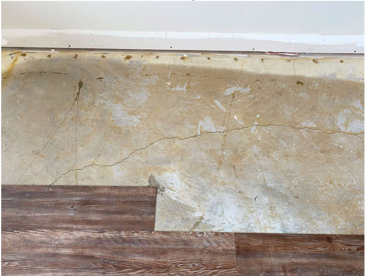
Picture 1: Porous and cracked subfloor absorbed glue
