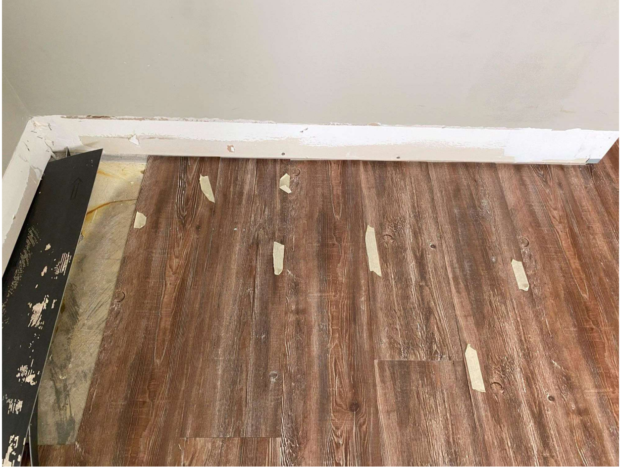
Picture 44: Failure to comply to the installation guidelines as required by the manufacturer
