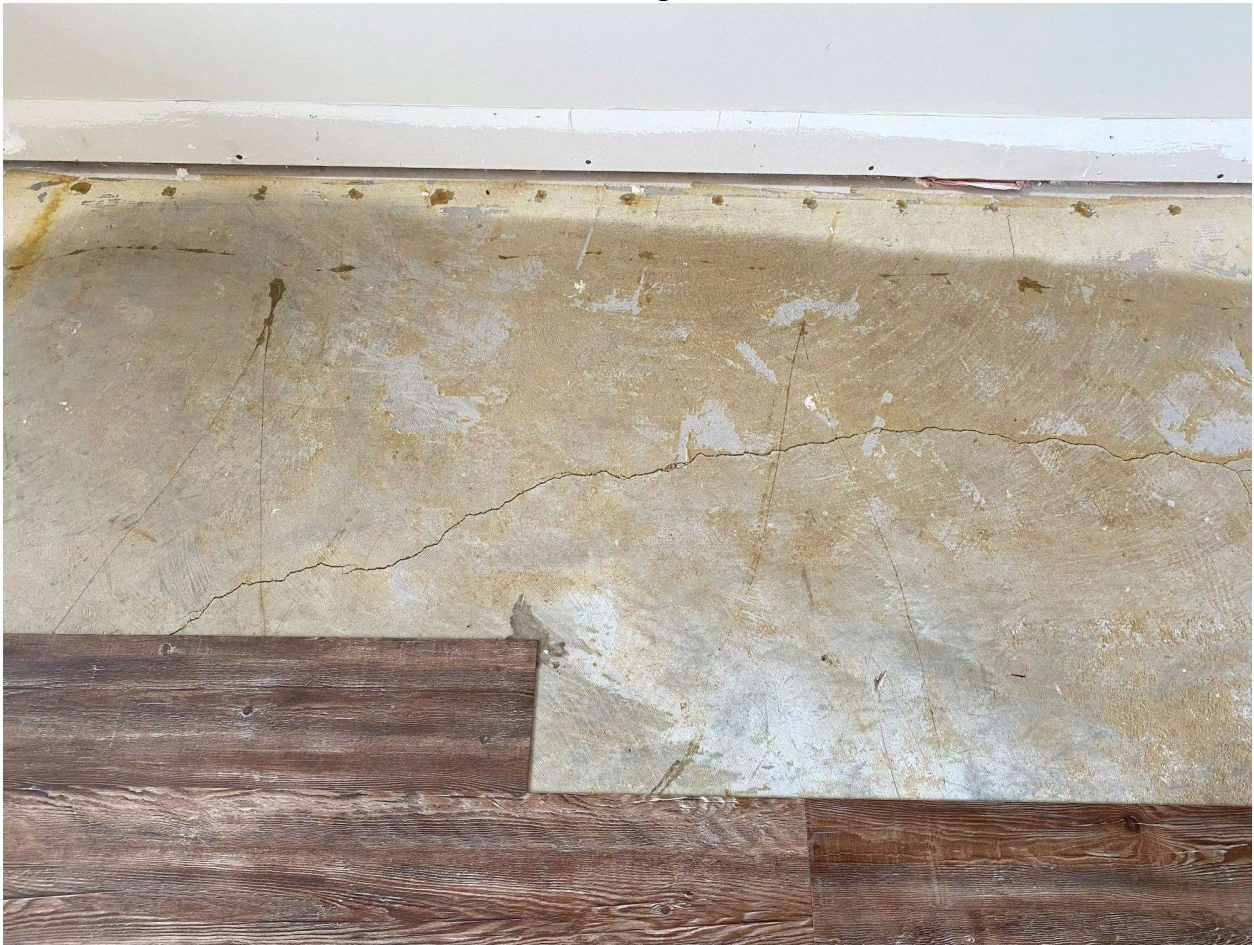
Picture 1: Porous and cracked subfloor absorbed glue
