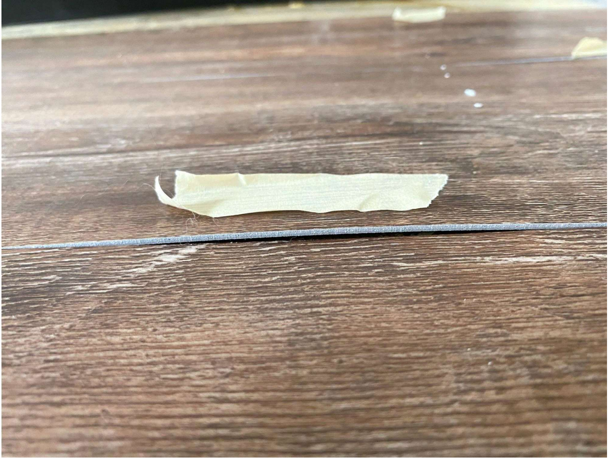
Picture 42: Failure to comply to the installation guidelines as required by the manufacturer
