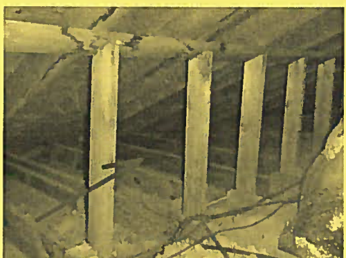
No insulation present in rear of attic
