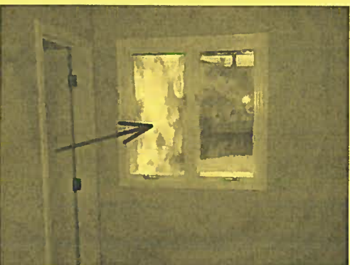
Insulated glass seal has failed (glass fogged)
