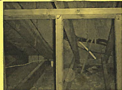
Vertical wall in sunroom is missing insulation
