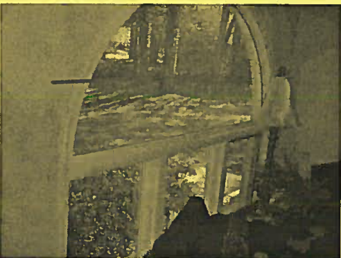
Insulated glass seal has failed (glass fogged)
