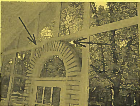
Broken glass on R and both sections are not sealed
