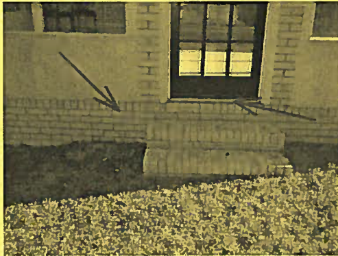
Stress crack and gap under door
