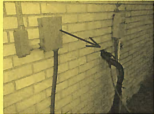
Wall penetrations are not sealed
