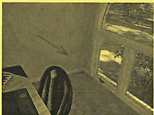
This wall outlet is not working
