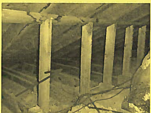
No insulation present in rear of attic
