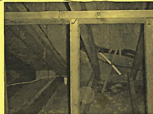
Vertical wall in sunroom is missing insulation
