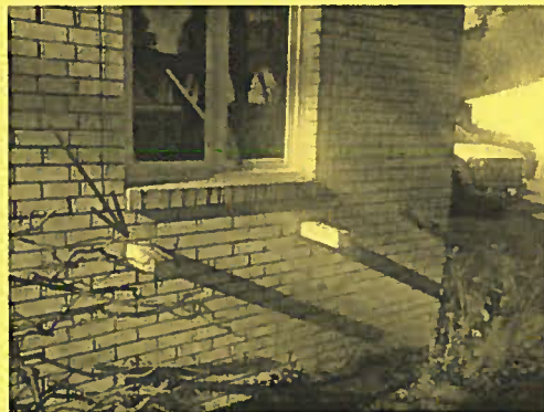
Windowsill on R front has water damaged. Deco woodpost are loose in wall
