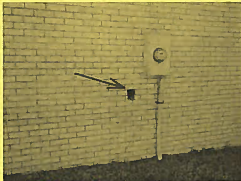
Wall penetrations are not sealed, several of these
