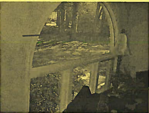
Insulated glass seal has failed (glass fogged)
