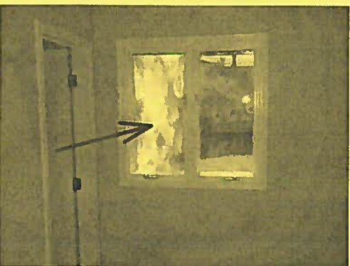
Insulated glass seal has failed (glass fogged)
