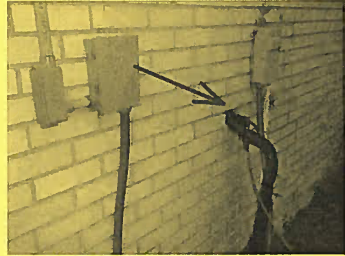
Wall penetrations are not sealed
