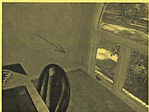
This wall outlet is not working
