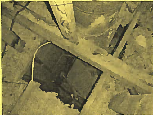
Rust on fireplace box and flue from previous leaks. Open area (chase) around fireplace is not sealed
