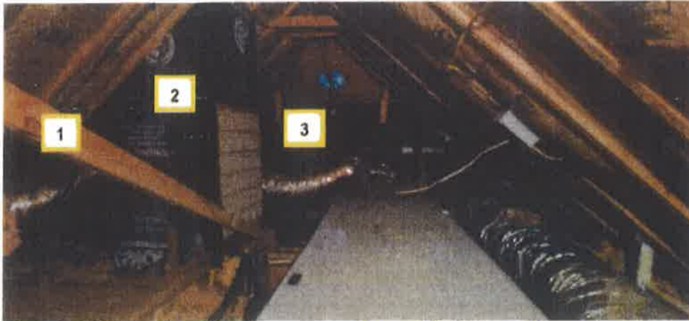
Photo 3. Attic overview. (1) loose gable end brace, (2) chimney, (3) over-framed portion of roof.
