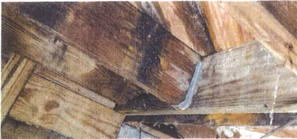
Photo 27. Deck ledger (no lag screws observed).
