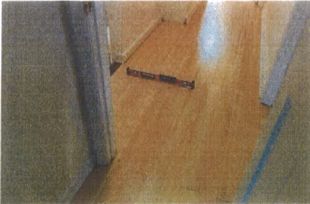
6. Floor slope 2.8% at stair landing.
