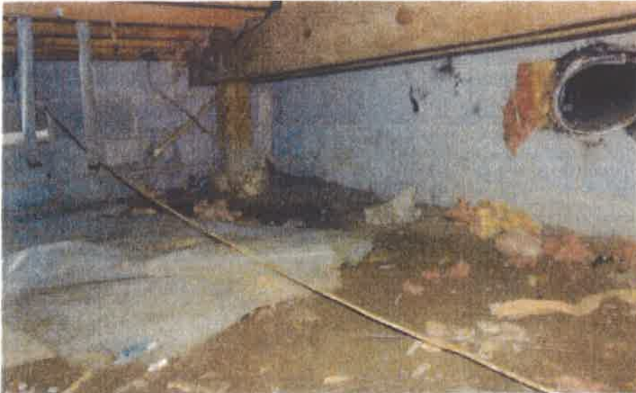
23. Drop girder in crawl space. The girder does not contact the joists and ore, does not support the floor framing.
