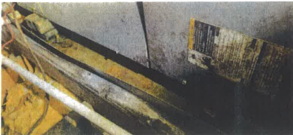
Photo 4. AHU catch pan. Note fungal hyphae and evidence of deterioration to AHU platform.
