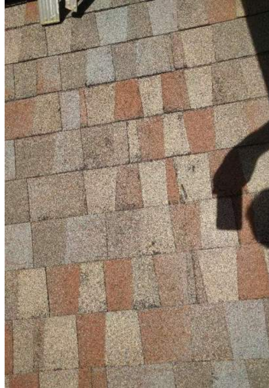
MARRED SHINGLES DUE TO A HOT WEATHER INSTALLATION
