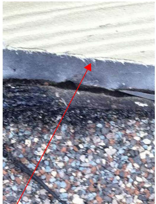
Cut Edges Not Primed, Painted Or Caulked
