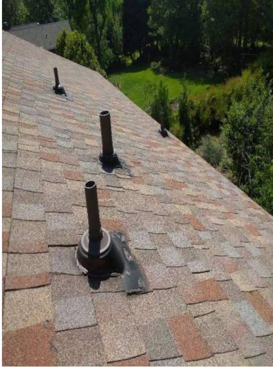
PAINT PEELING ON BOOTS
