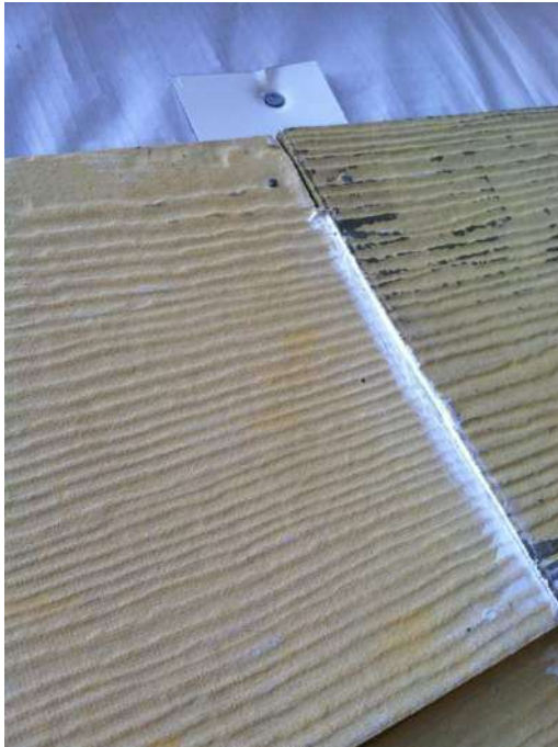
Butt Joint W/ Wrong Type Of Nails (Finish Nails Are Not Acceptable Here)
