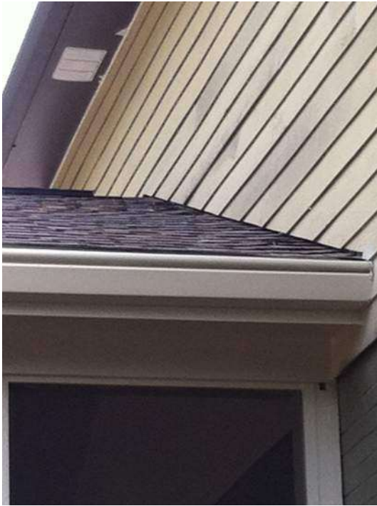
Step & Kick Out Flashing Not Installed Where Roof Meets Wall
