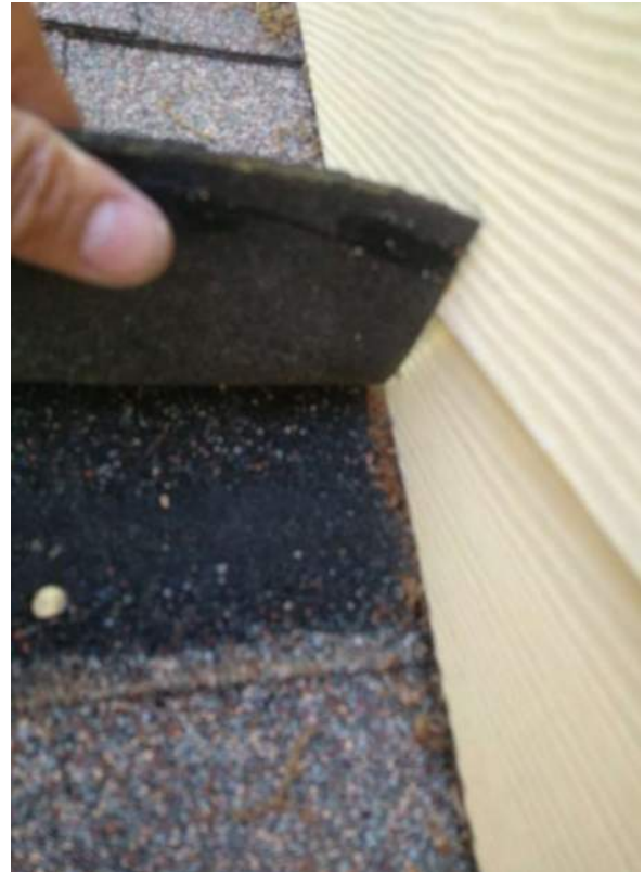
NO STEP FLASHING ON WALL
