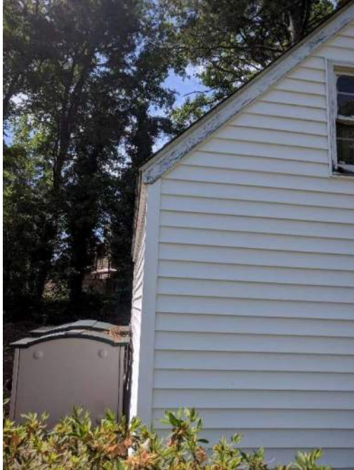
SHED IS MISSING DRIP EDGE
