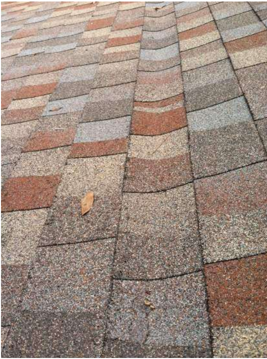
Shingles Installed With A Gutter Effect (GAF Technical Support Advised This Will Eventually Start Leaking)
