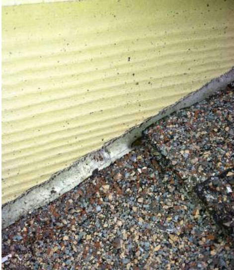
Step Flashing Not Installed
