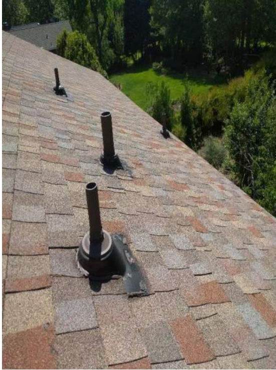
PAINT PEELING ON BOOTS
