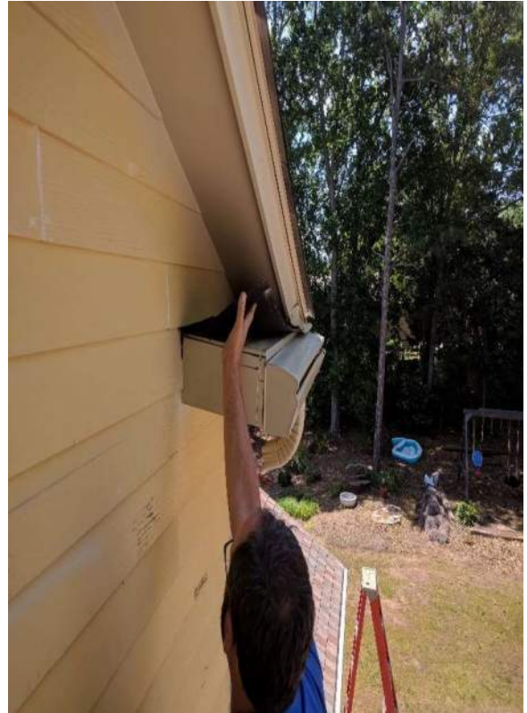
NO UNDERLAYMENT INSTALLED
