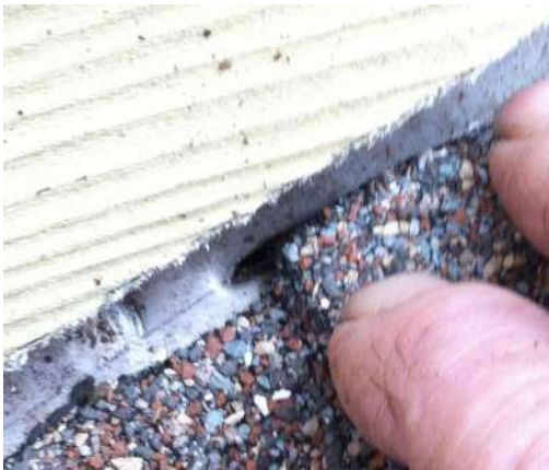
Slit In Flashing (Several Places)
