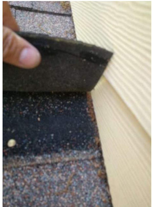
NO STEP FLASHING ON WALL
