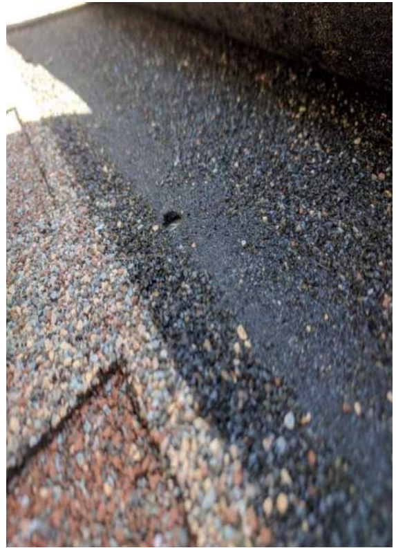
NAILS HAVE SHOT THROUGH
