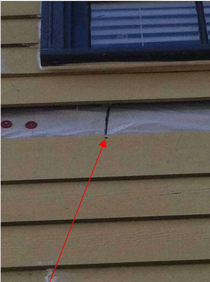
COUNTERSUNK NAIL BUT NO SECOND NAIL
