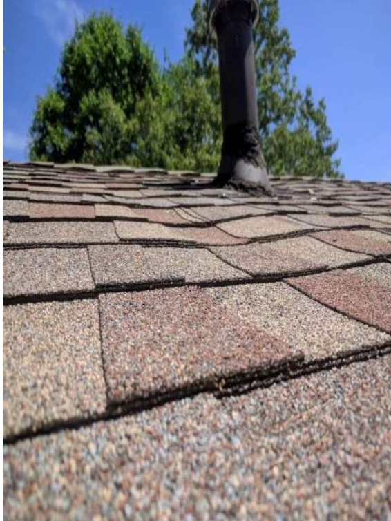
SOFT UNEVEN WOOD ON TOP PART OF HOUSE
