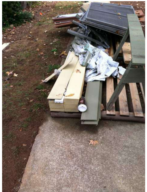
Hardie Plank Was Left Uncovered. That Is A No No
