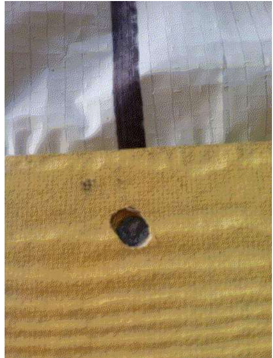
Countersunk Nails (Should Have Been Caulked And A Second Nail Installed)
