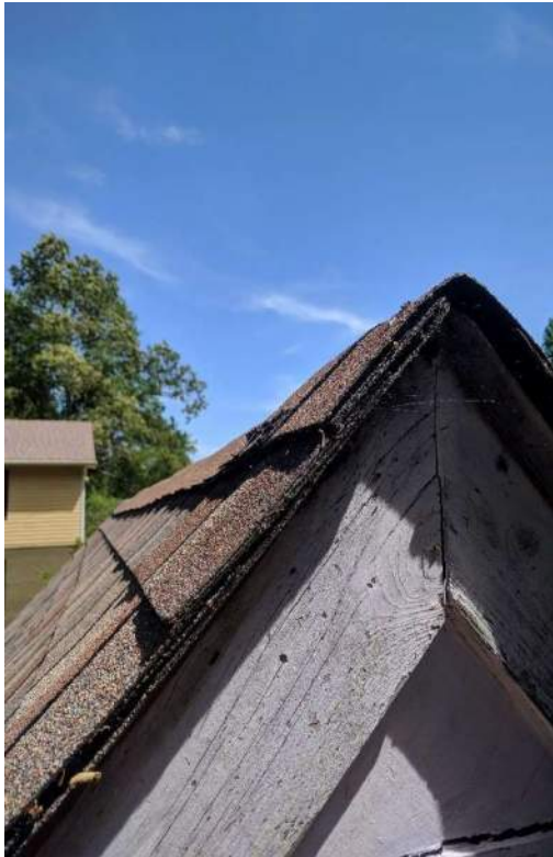
POOR VENTILATION ON SHED
