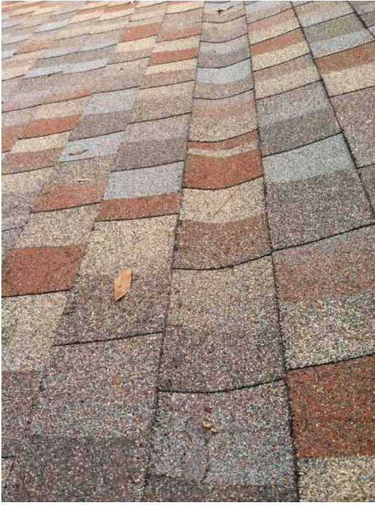
Shingles Installed With A Gutter Effect (GAF Technical Support Advised This Will Eventually Start Leaking)
