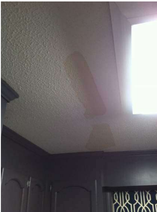
Damaged Kitchen Ceiling From Water Leak
