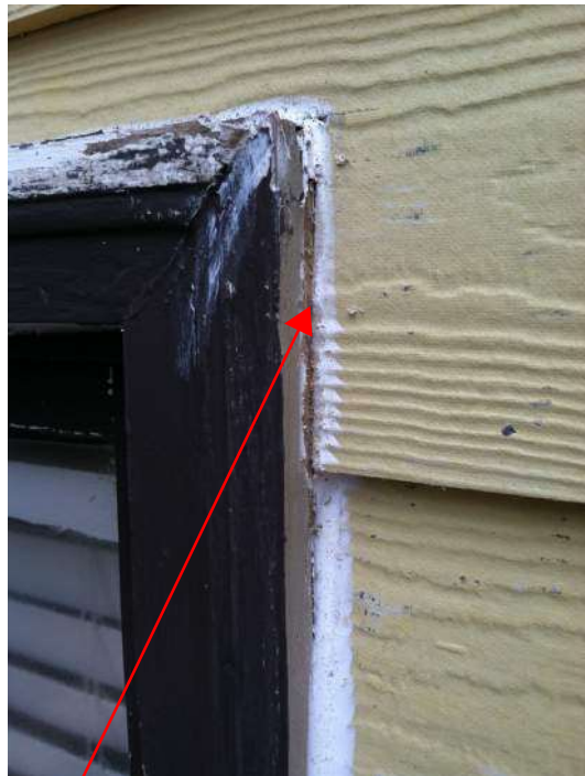
Gap Not Provided At Windows For Caulking
