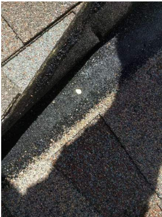
HIGH NAIL ON THE TOP ROOF
