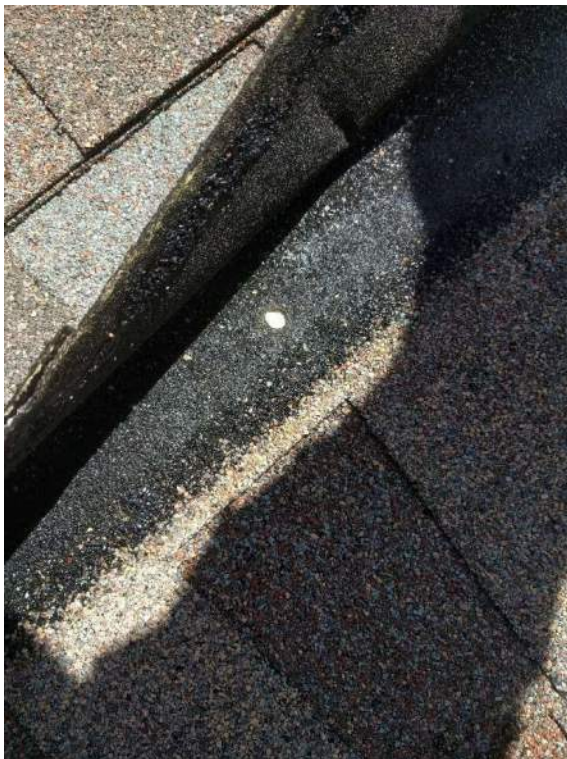
HIGH NAIL ON THE TOP ROOF
