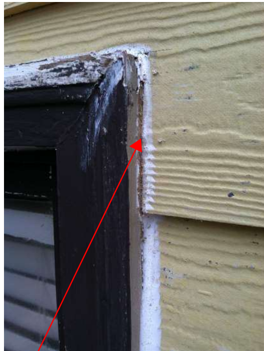
Gap Not Provided At Windows For Caulking
