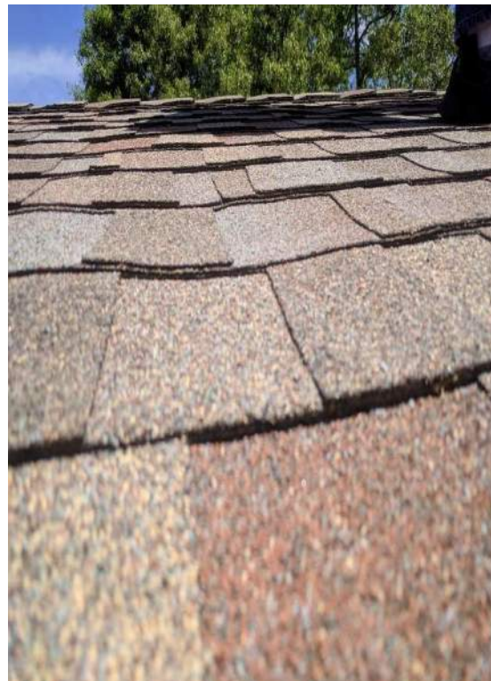
DECK BUCKLING ON THE TOP ROOF
