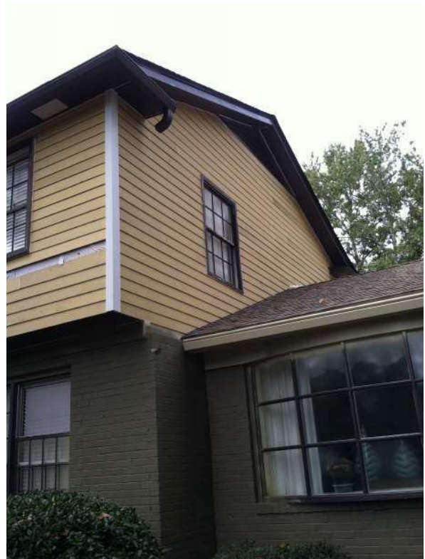
Step Flashing Not Installed Where Roof Meets Wall
