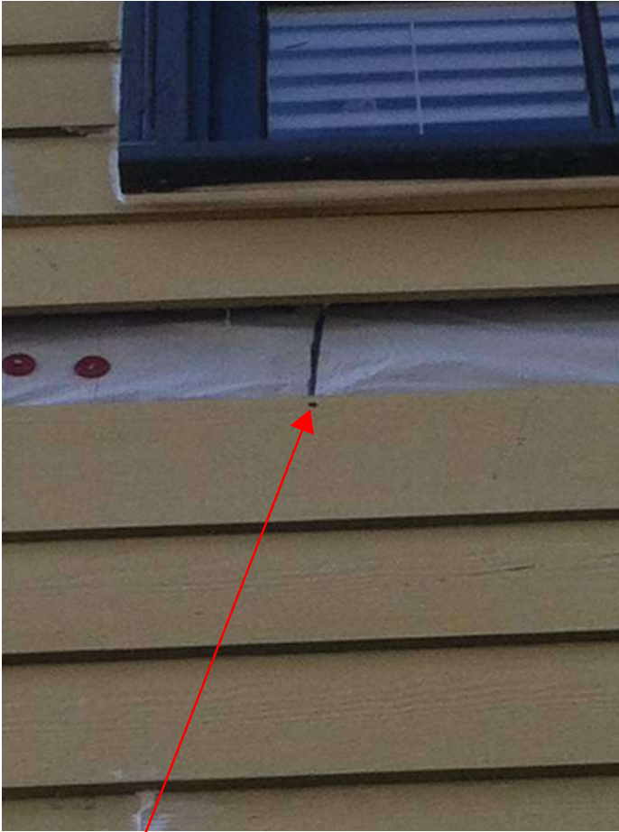
COUNTERSUNK NAIL BUT NO SECOND NAIL
