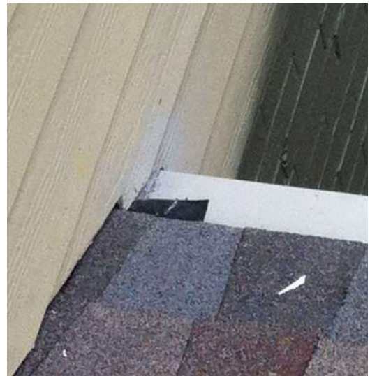
Kick Out Flashing Not Installed
