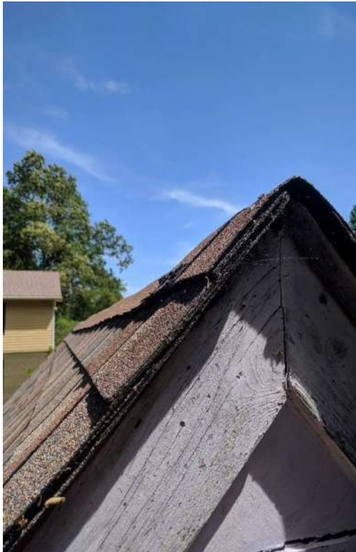
POOR VENTILATION ON SHED
