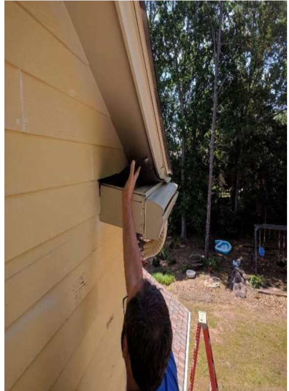
NO UNDERLAYMENT INSTALLED
