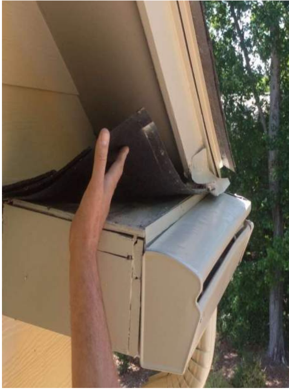
POOR WORK ON RETURNS, FEW NAILS
