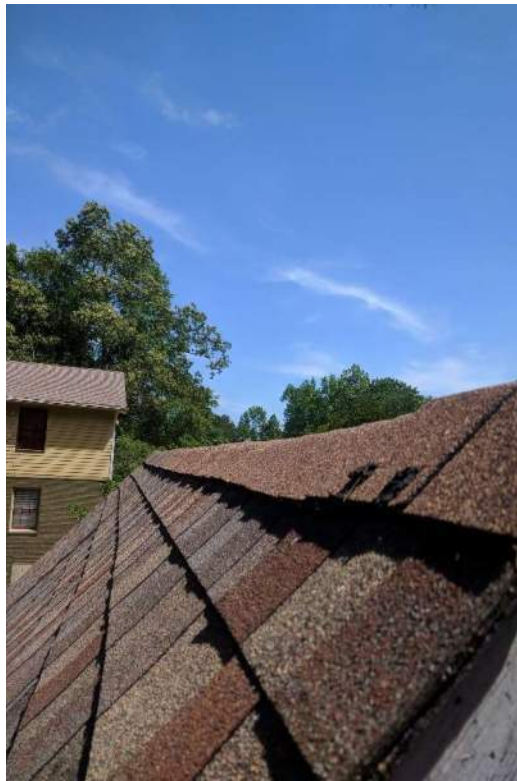
POOR VENTILATION ON SHED
