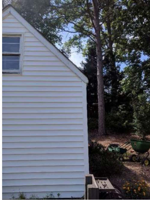
SHED IS MISSING DRIP EDGE
