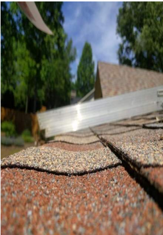
DIP IN ROOF HOLDS WATER
