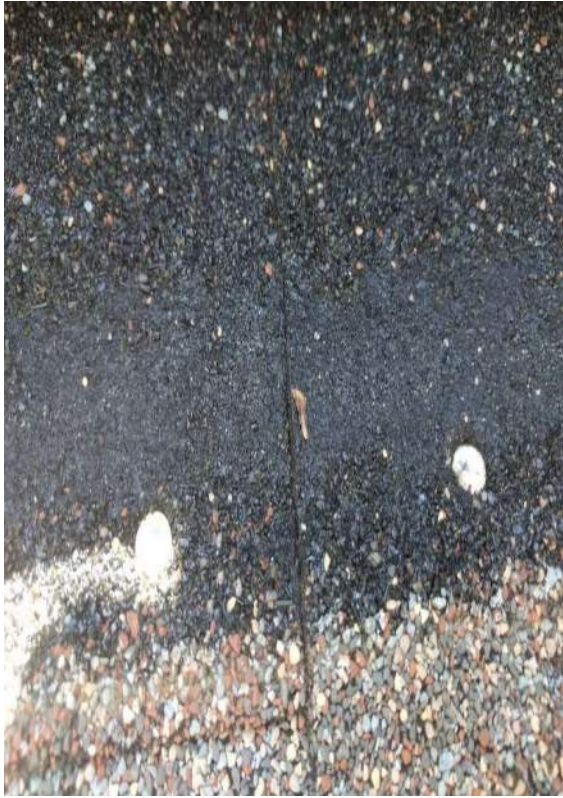
UNEVEN NAILING PATTERN
