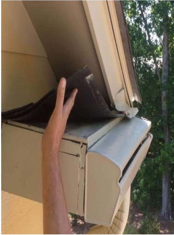
POOR WORK ON RETURNS, FEW NAILS
