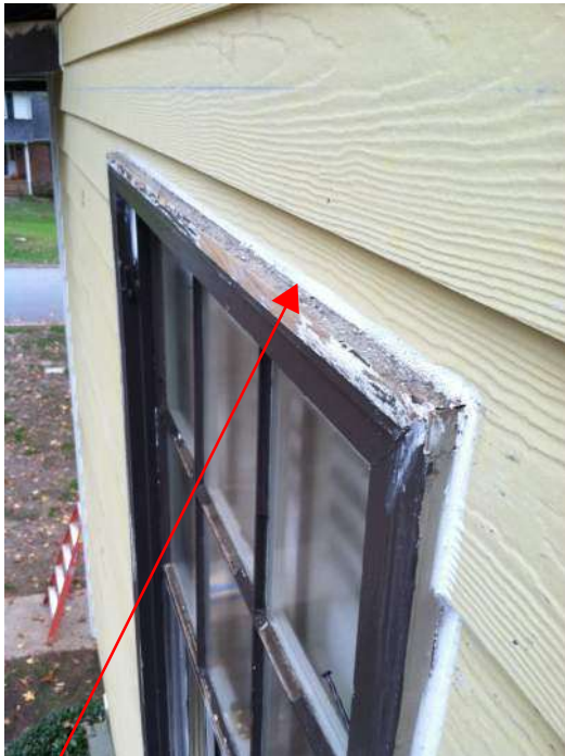
Metal Flashing Over Windows Not Provided
