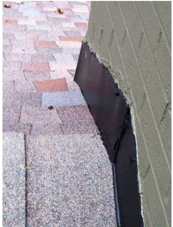
Step Flashing Improperly Nailed At Chimney
