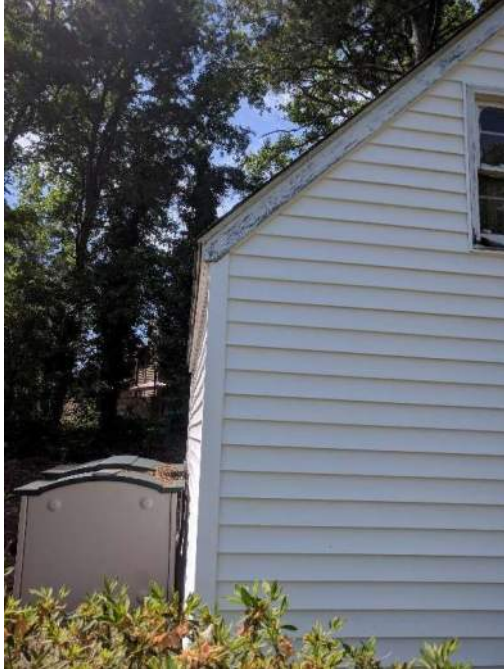
SHED IS MISSING DRIP EDGE
