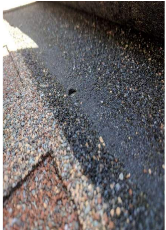
NAILS HAVE SHOT THROUGH
