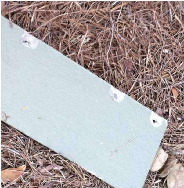
Countersunk Nail Holes With No Second Nail?
