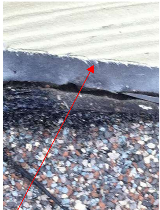
Cut Edges Not Primed, Painted Or Caulked
