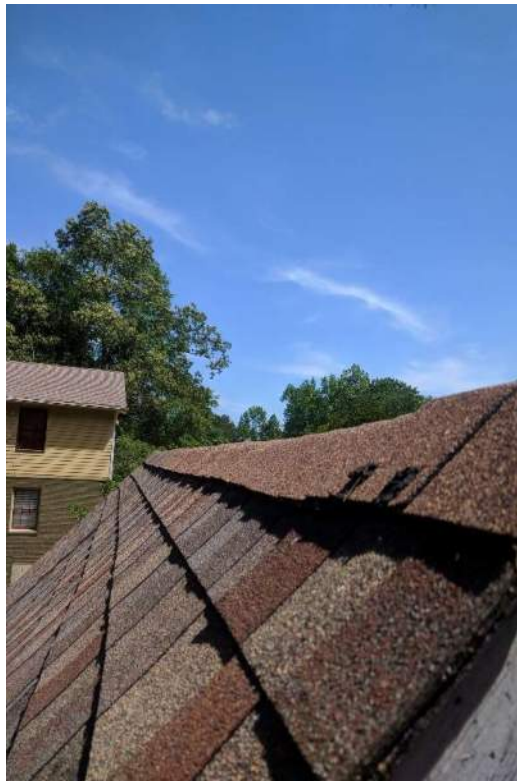
POOR VENTILATION ON SHED
