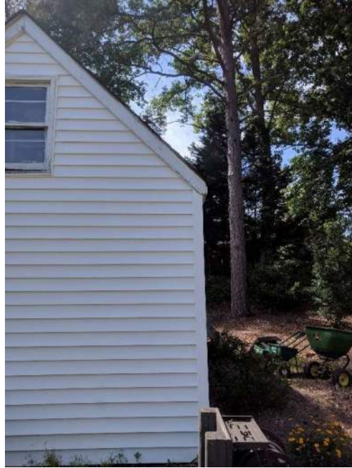
SHED IS MISSING DRIP EDGE
