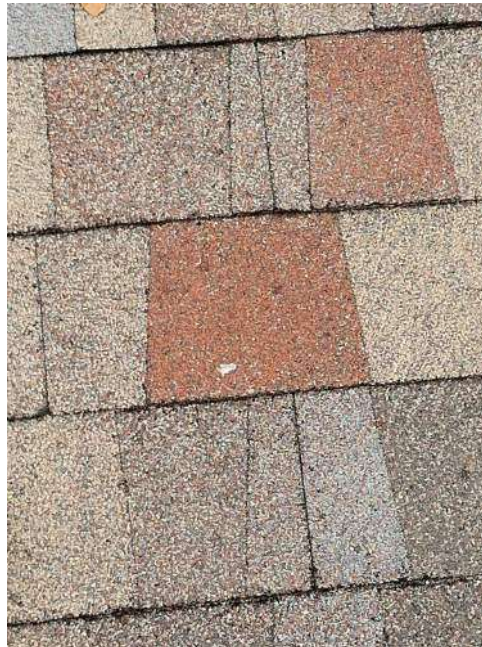
88 Some Spacing Between Shingle Joints On Adjacent Rows Is Too Close
