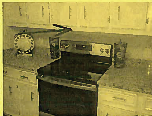
Low clearance above stove, 30in to combustibles required.
