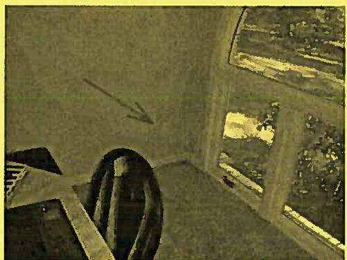
This wall outlet is not working
