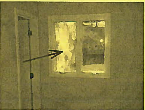
Insulated glass seal has failed (glass fogged)
