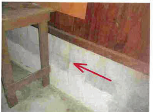
Stress crack in block wall of garage
