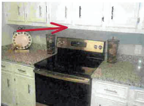
Low clearance above stove, 30in to combustables required.
