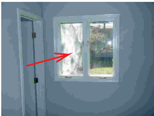
Insulated glass seal has failed (glass fogged)
