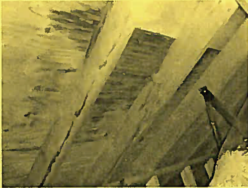
Dry stains in attic, possibly old, confirm all leaks have been repaired
