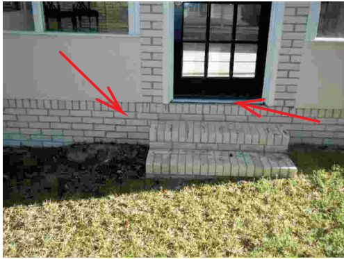
Stress crack and gap under door
