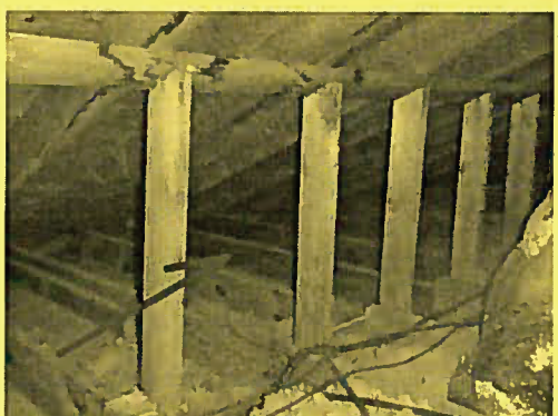
No insulation present in rear of attic
