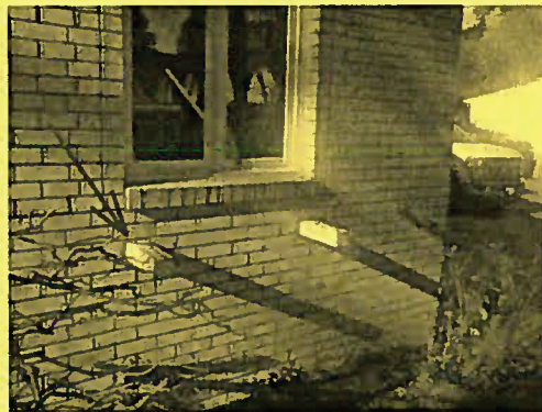
Windowsill on R front has water damaged. Deco woodpost are loose in wall
