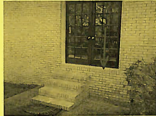
Master bedroom back doors are missing handrailing and one door opens without steps or landing below
