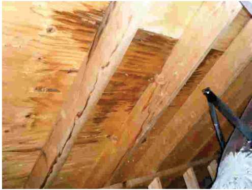
Dry stains in attic, possibly old, confirm all leaks have been repaired
