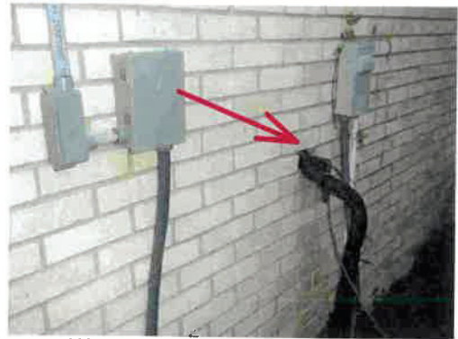
Wall penetrations are not sealed
