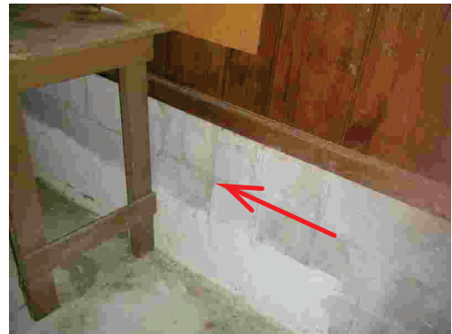
Stress crack in block wall of garage
