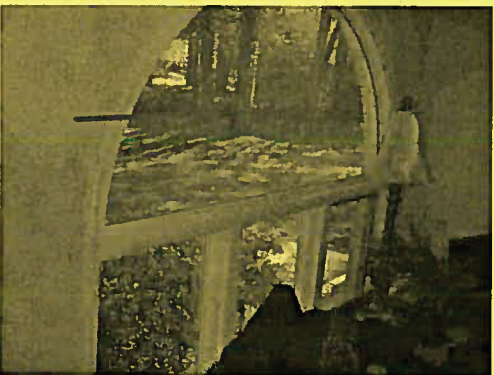
Insulated glass seal has failed (glass fogged)
