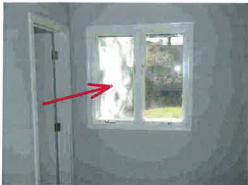
Insulated glass seal has failed (glass fogged)
