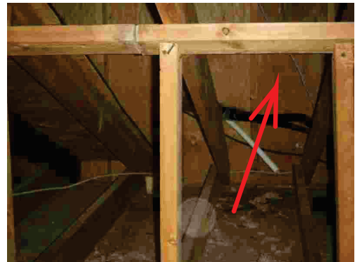
Vertical wall in sunroom is missing insulation
