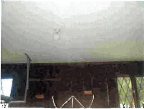
Ceiling texture loose and peeling in garage, not due to leaks
