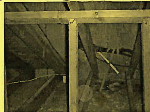
Vertical wall in sunroom is missing insulation
