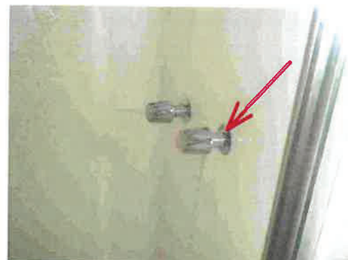
Master shower valve stems are leaking
