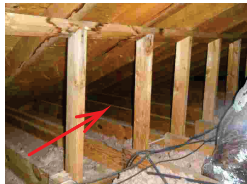
No insulation present in rear of attic
