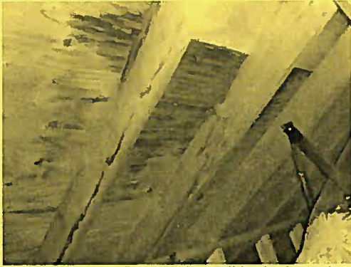
Dry stains in attic, possibly old, confirm all leaks have been repaired
