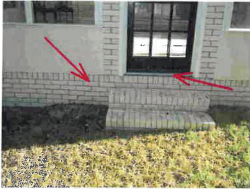
Stress crack and gap under door
