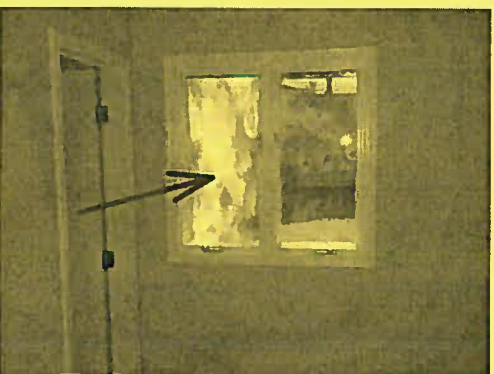
Insulated glass seal has failed (glass fogged)
