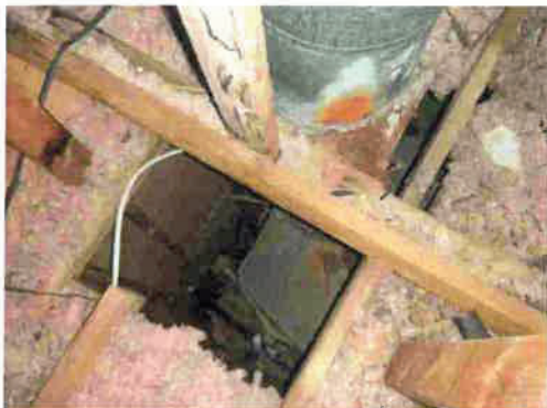
Rust on fireplace box and flue from previous leaks. Open area (chase) around fireplace is not sealed
