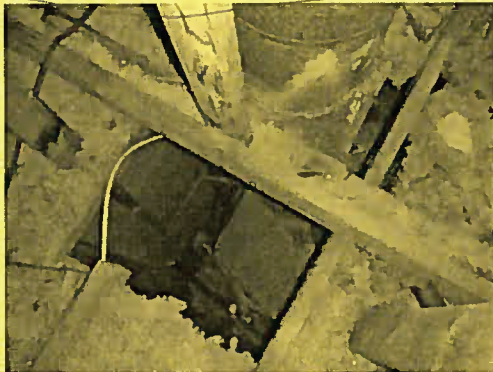
Rust on fireplace box and flue from previous leaks. Open area (chase) around fireplace is not sealed
