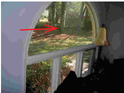
Insulated glass seal has failed (glass fogged)
