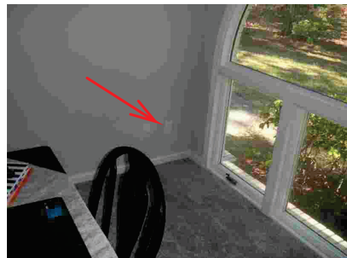
This wall outlet is not working
