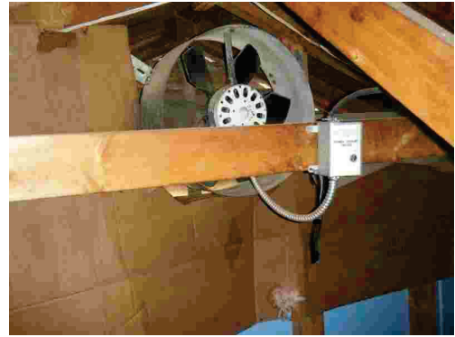
Motors are burned out in attic vent fans (both units)
