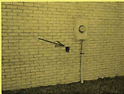
Wall penetrations are not sealed, several of these
