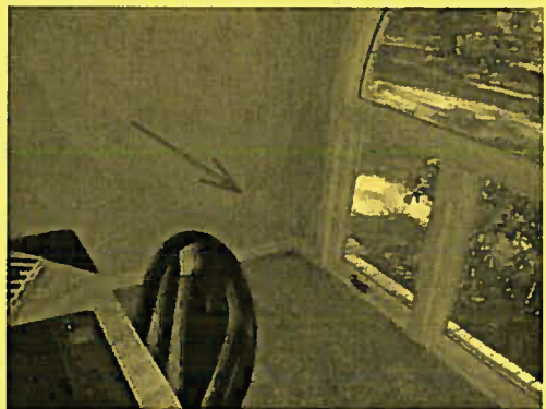
This wall outlet is not working
