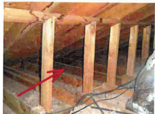
No insulation present in rear of attic
