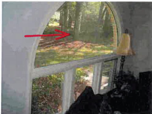
Insulated glass seal has failed (glass fogged)
