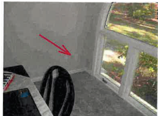
This wall outlet is not working
