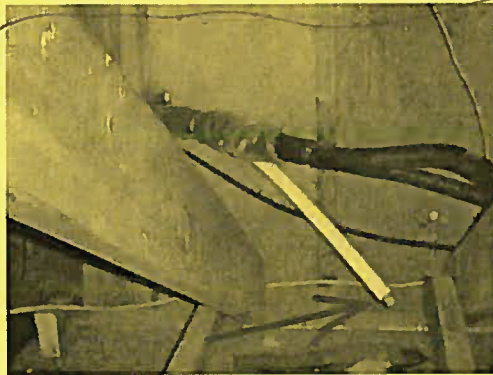
Appears installation is not complete for sunroom mini split system.
