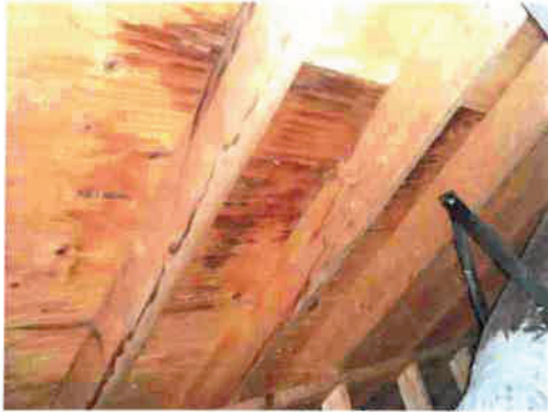
Dry stains in attic, possibly old, confirm all leaks have been repaired
