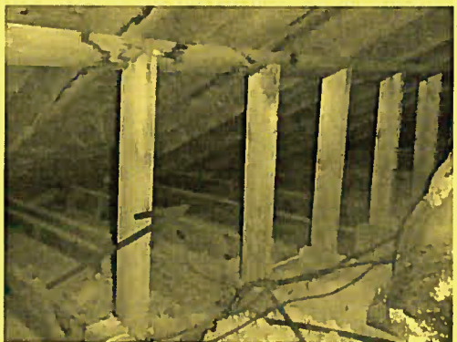
No insulation present in rear of attic
