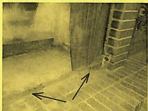
Metal fireplace is rusting out in some areas
