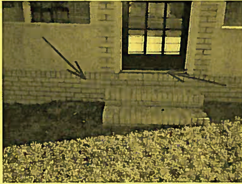
Stress crack and gap under door
