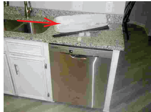
Some of the dishwasher parts have not been installed
