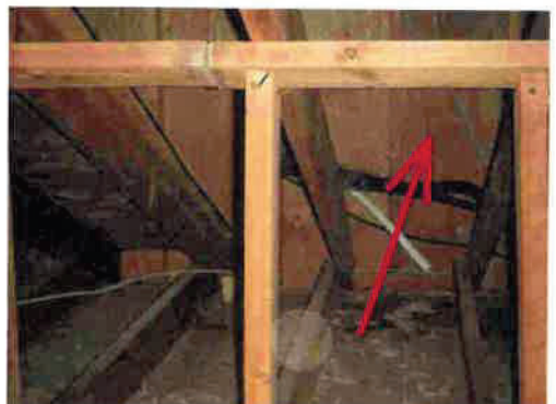
Vertical wall in sunroom is missing insulation
