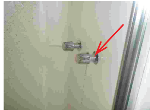
Master shower valve stems are leaking
