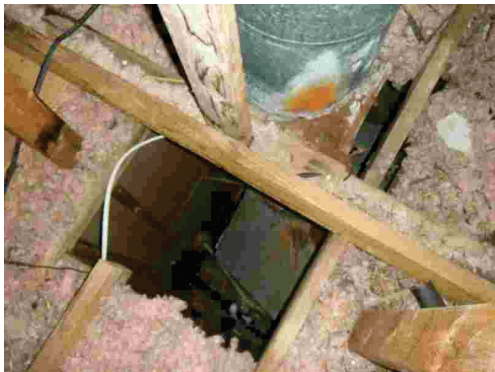
Rust on fireplace box and flue from previous leaks. Open area (chase) around fireplace is not sealed
