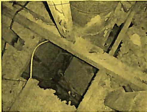
Rust on fireplace box and flue from previous leaks. Open area (chase) around fireplace is not sealed
