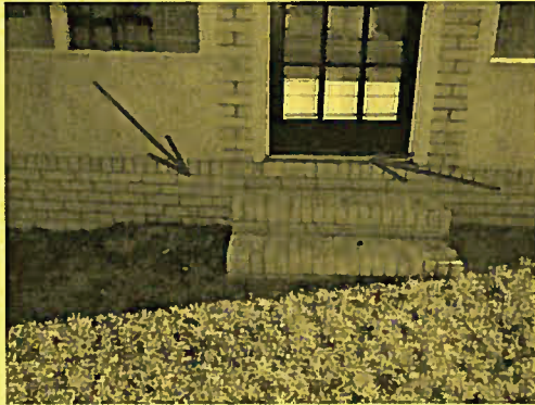
Stress crack and gap under door
