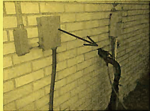
Wall penetrations are not sealed
