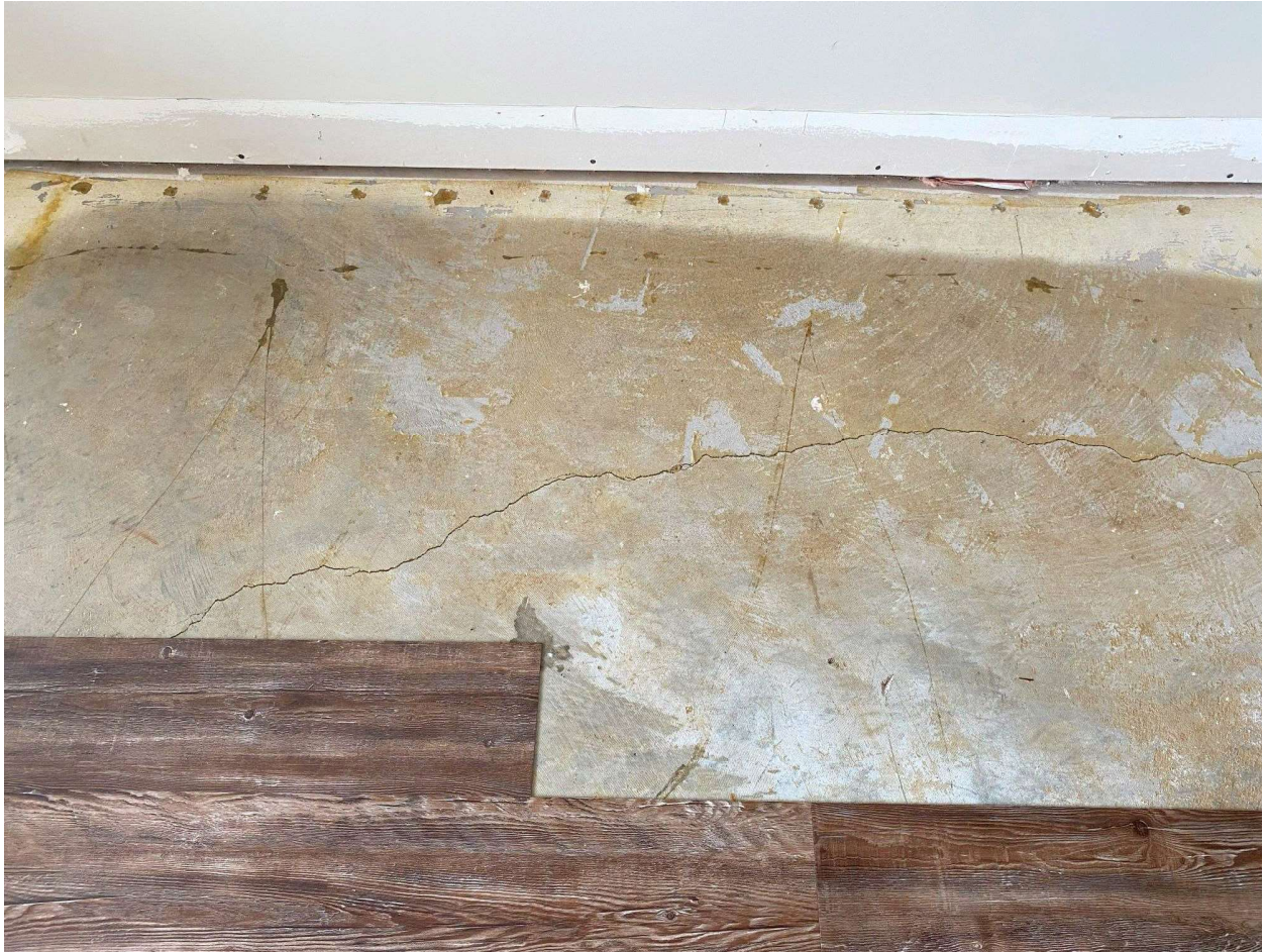
Picture 1: Porous and cracked subfloor absorbed glue
