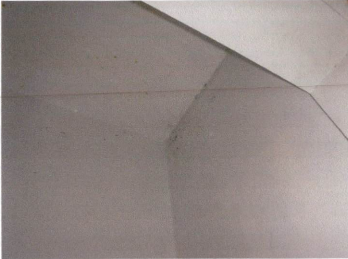
Mold at linen closet wall and ceiling at hall bath.
