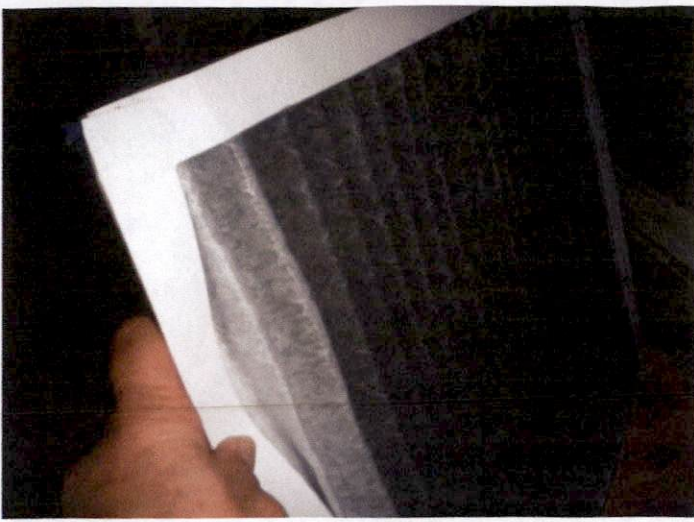
Very heavy debris at HVAC return vent filter.
