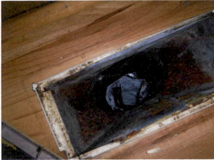
Very heavy rust, debris, and water, at kitchen HVAC supply vent.
