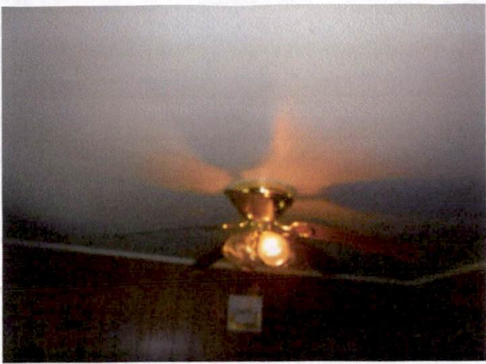
Fan blades warped from excessive humidity.
