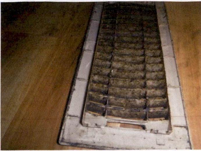
Very heavy debris at HVAC supply vent cover.
