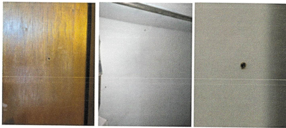
Bullet hole in my closet door and through the back wall of the closet
