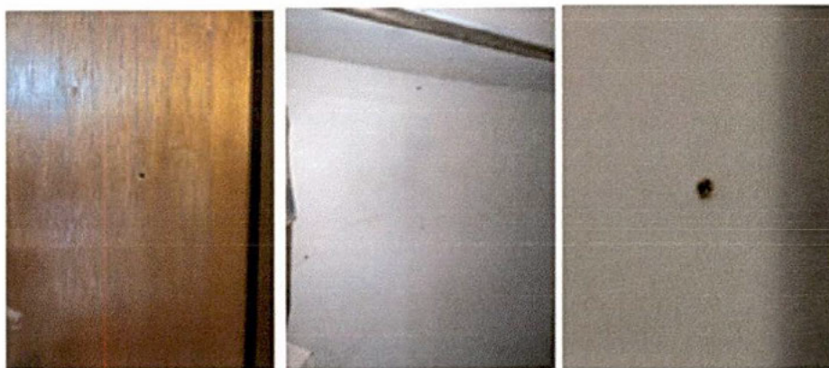
Bullet hole in my closet door and through the back wall of the closet
