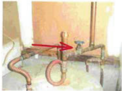
Valve at top of water heater is leaking
