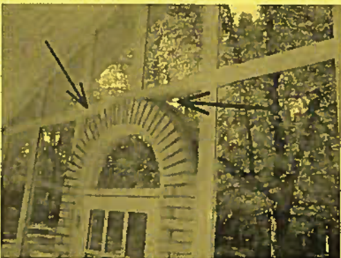
Broken glass on R and both sections are not sealed
