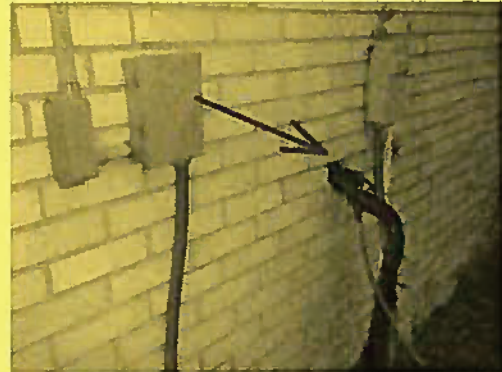
Wall penetrations are not sealed
