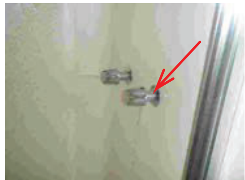
Master shower valve stems are leaking
