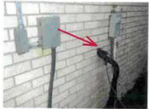
Wall penetrations are not sealed
