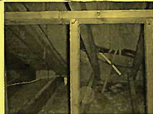
Vertical wall in sunroom is missing insulation
