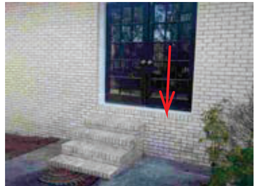
Master bedroom back doors are missing handrailing and one door opens without steps or landing below
