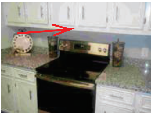
Low clearance above stove, 30in to combustibles required.
