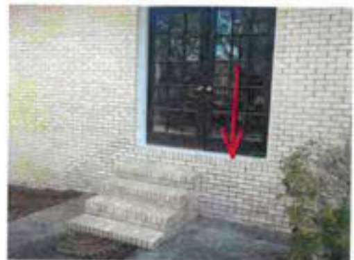
Master bedroom back doors are missing handrailing and one door opens without steps or landing below
