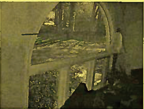
Insulated glass seal has failed (glass fogged)
