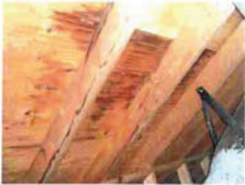
Dry stains in attic, possibly old, confirm all leaks have been repaired
