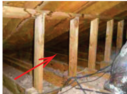
No insulation present in rear of attic
