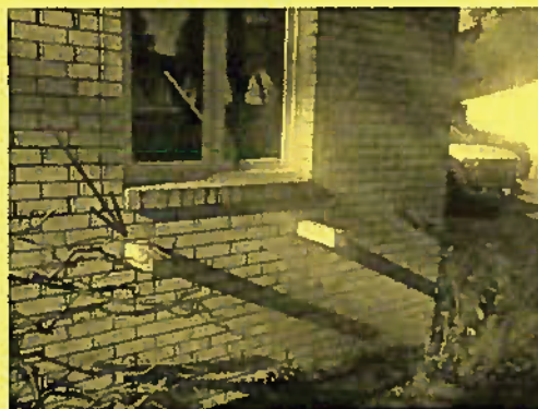
Windowsill on R front has water damaged. Deco woodpost are loose in wall
