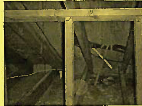
Vertical wall in sunroom is missing insulation
