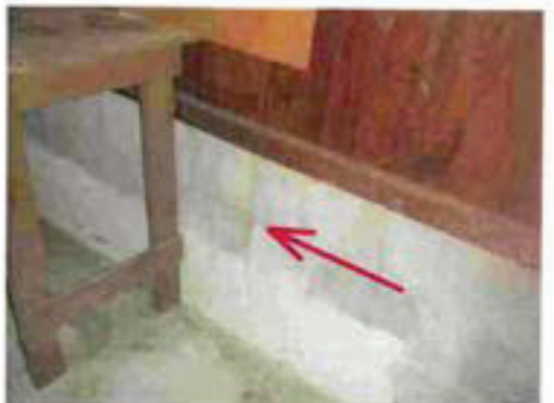
Stress crack in block wall of garage
