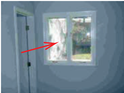
Insulated glass seal has failed (glass fogged)
