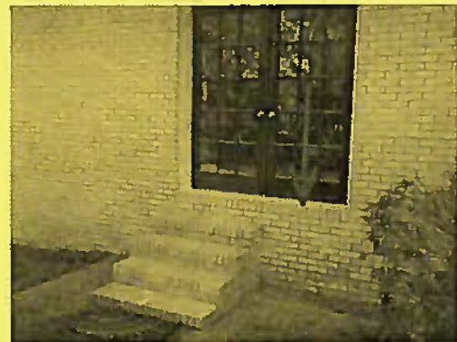
Master bedroom back doors are missing handrailing and one door opens without steps or landing below
