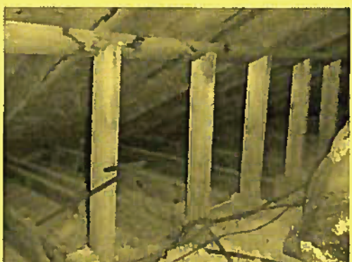
No insulation present in rear of attic
