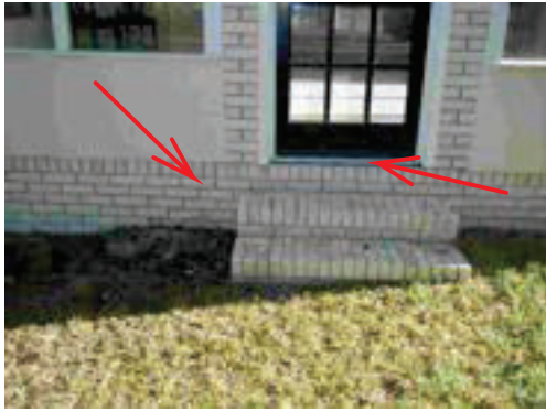
Stress crack and gap under door
