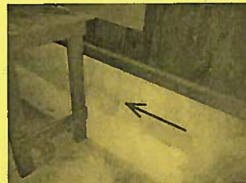
Stress crack in block wall of garage
