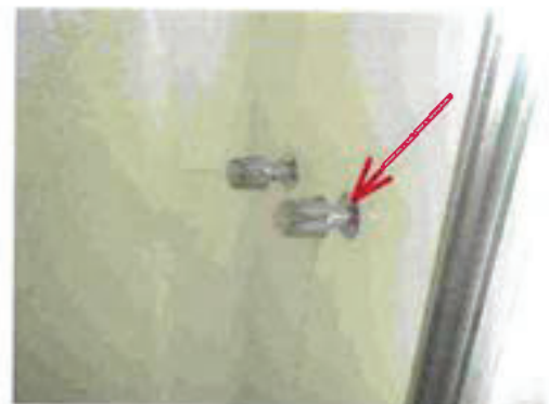
Master shower valve stems are leaking
