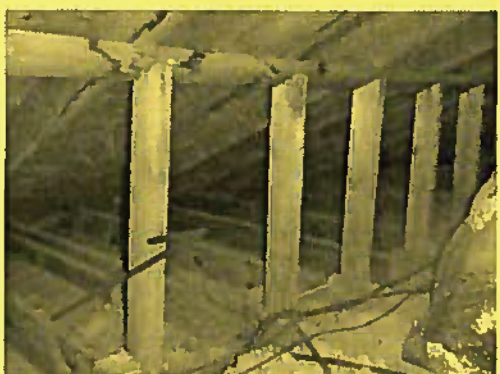
No insulation present in rear of attic
