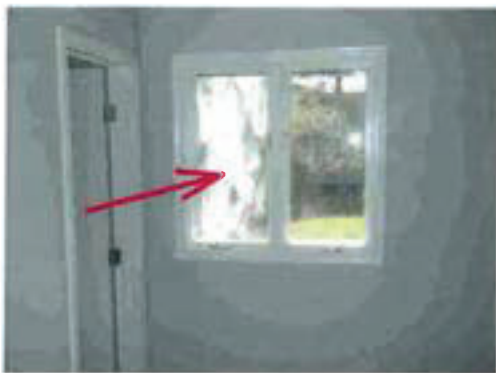
Insulated glass seal has failed (glass fogged)
