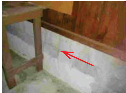
Stress crack in block wall of garage
