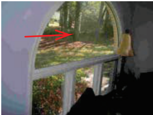
Insulated glass seal has failed (glass fogged)
