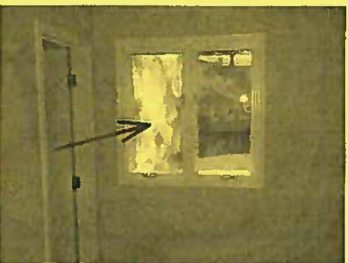
Insulated glass seal has failed (glass fogged)
