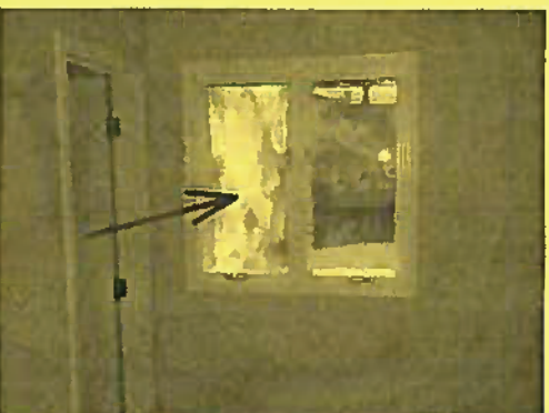
Insulated glass seal has failed (glass fogged)
