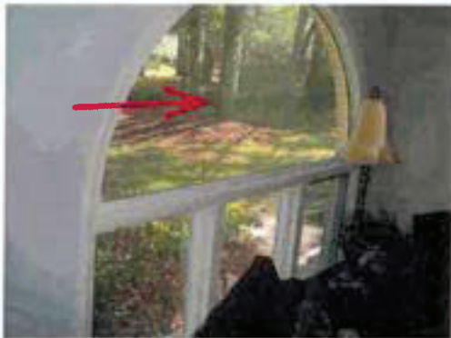
Insulated glass seal has failed (glass fogged)
