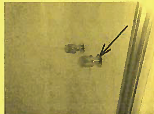
Master shower valve stems are leaking
