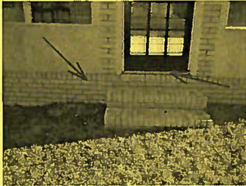
Stress crack and gap under door
