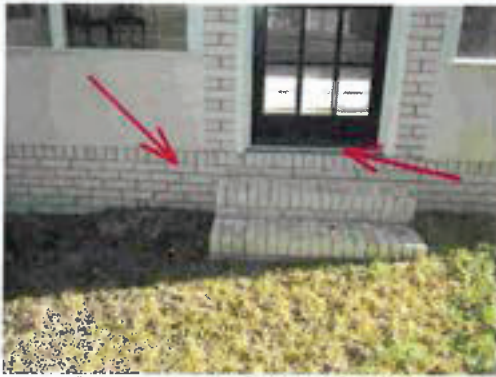
Stress crack and gap under door
