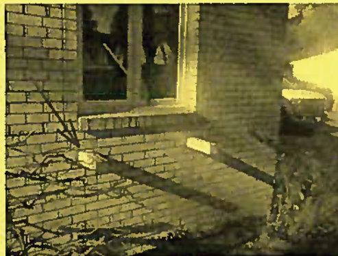
Windowsill on R front has water damaged. Deco woodpost are loose in wall
