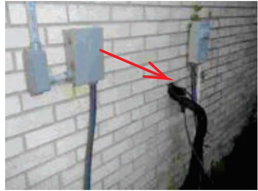
Wall penetrations are not sealed
