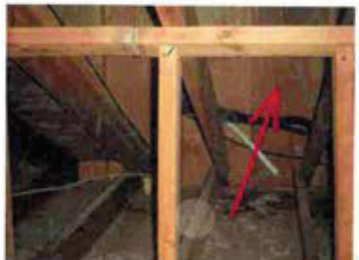
Vertical wall in sunroom is missing insulation
