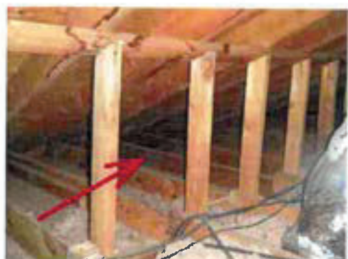
No insulation present in attic
