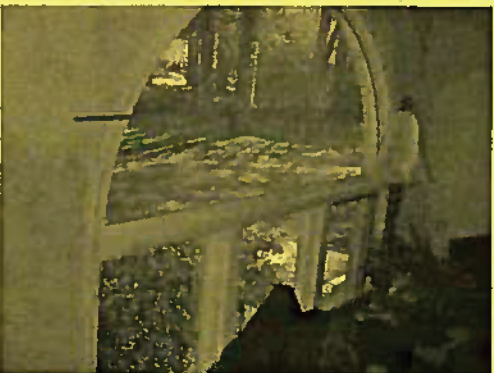
Insulated glass seal has failed (glass fogged)
