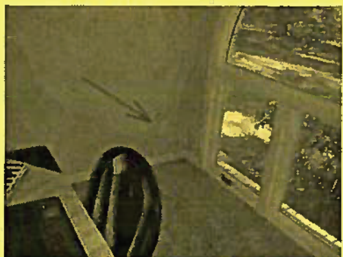
This wall outlet is not working
