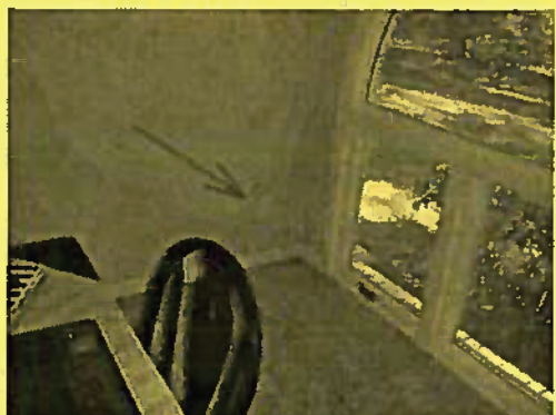
This wall outlet is not working
