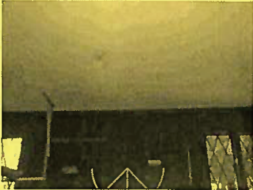
Ceiling texture loose and peeling in garage, not due to leaks
