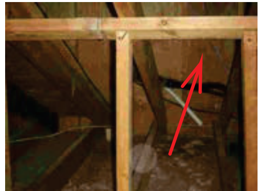
Vertical wall in sunroom is missing insulation
