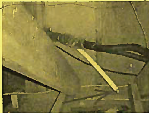
Appears installation is not complete for sunroom mini split system.
