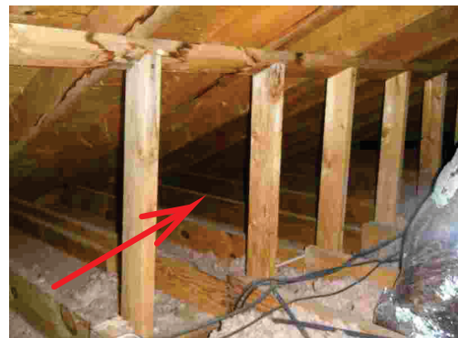
No insulation present in rear of attic
