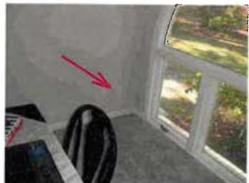
This wall outlet is not working
