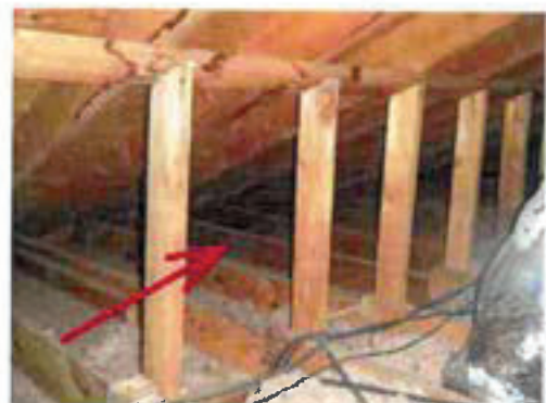
No insulation present in rear of attic
