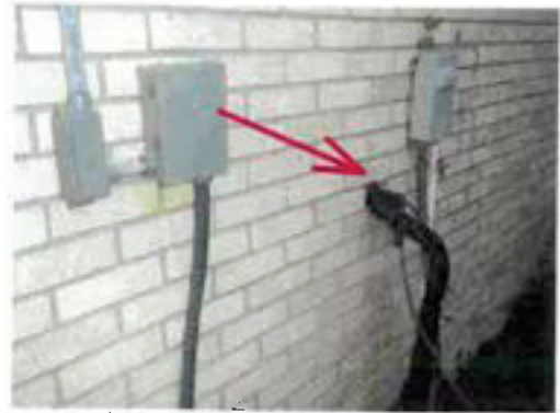
Wall penetrations are not sealed
