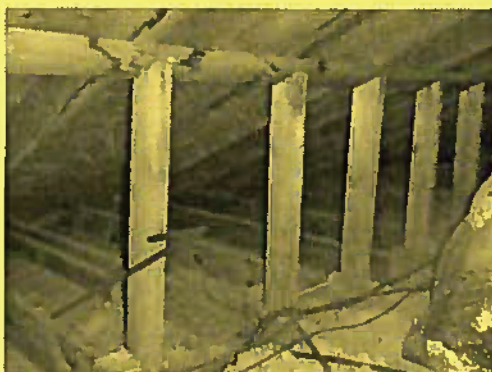
No insulation present in rear of attic
