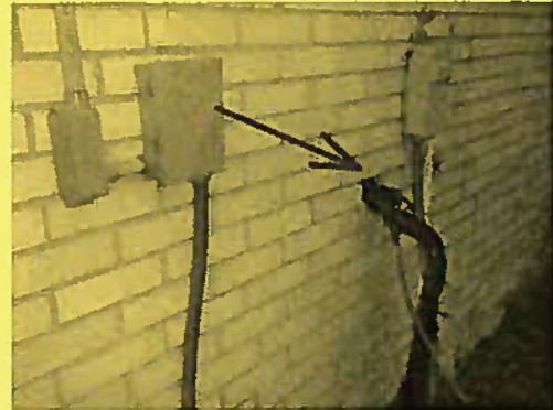
Wall penetrations are not sealed
