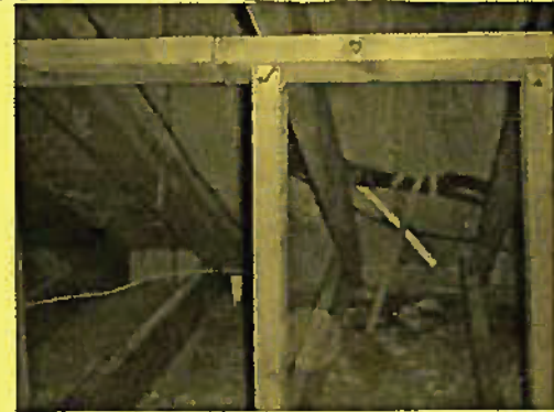
Vertical wall in sunroom is missing insulation
