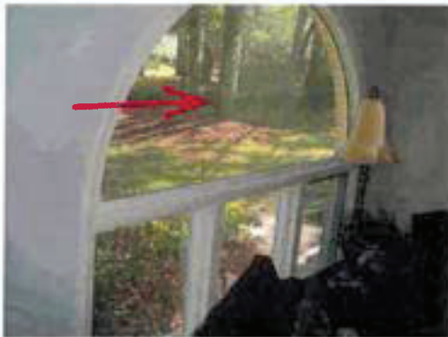
Insulated glass seal has failed (glass fogged)
