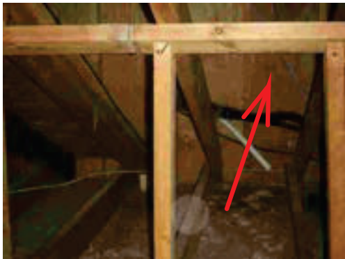
Vertical wall in sunroom is missing insulation
