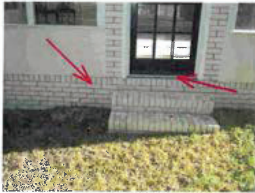
Stress crack and gap under door
