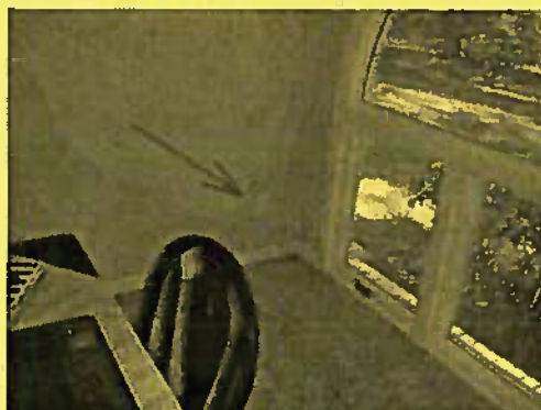
This wall outlet is not working
