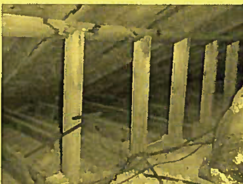
No insulation present in rear of attic
