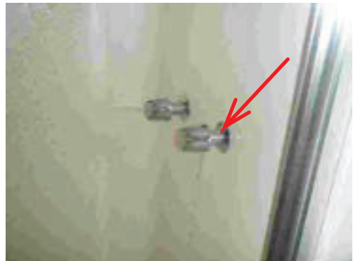
Master shower valve stems are leaking
