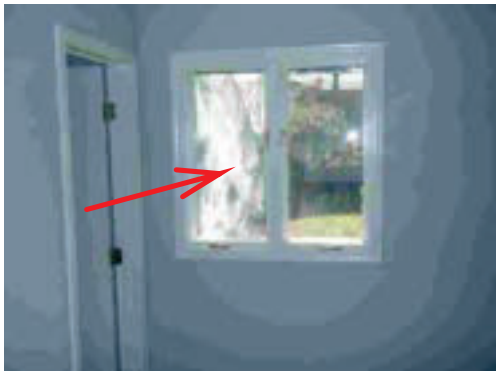
Insulated glass seal has failed (glass fogged)
