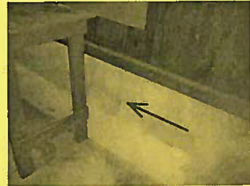
Stress crack in block wall of garage
