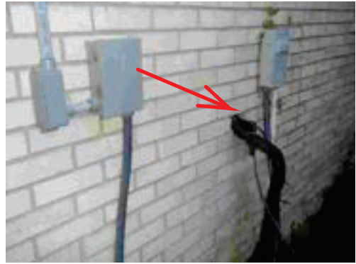
Wall penetrations are not sealed
