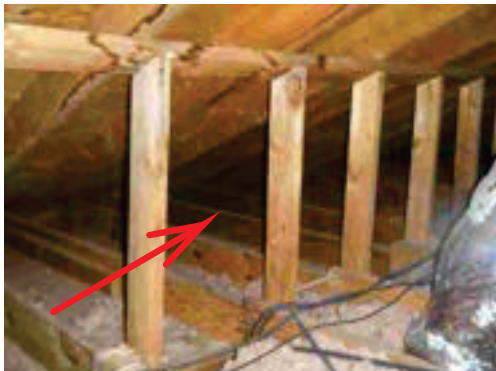
No insulation present in rear of attic
