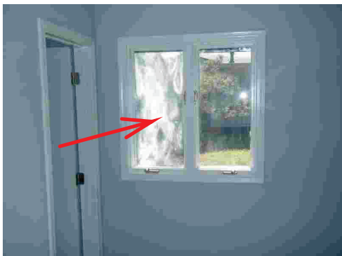
Insulated glass seal has failed (glass fogged)
