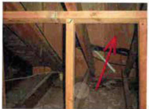
Vertical wall in sunroom is missing insulation
