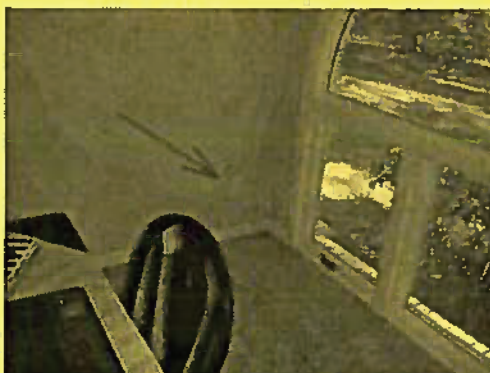
This wall outlet is not working
