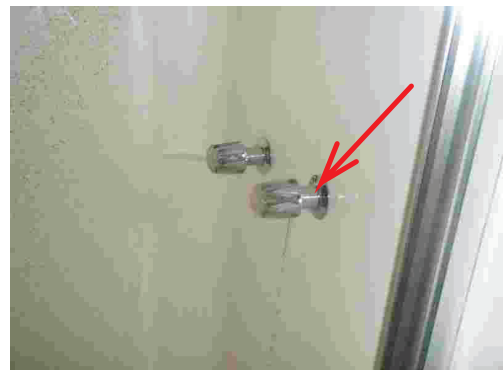
Master shower valve stems are leaking
