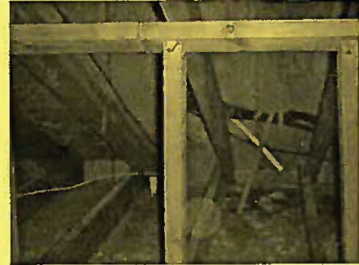
Vertical wall in sunroom is missing insulation
