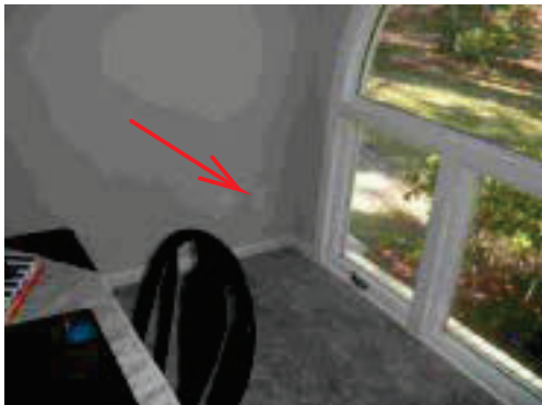
This wall outlet is not working
