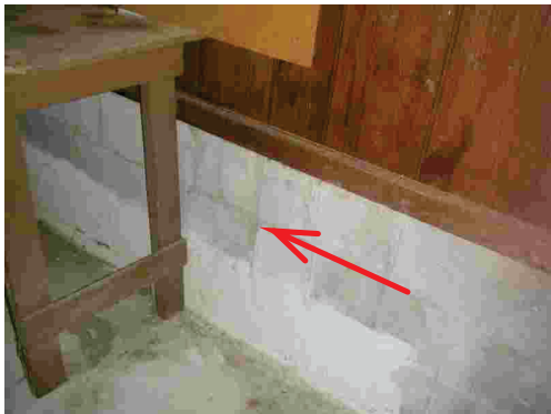
Stress crack in block wall of garage
