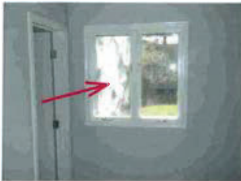
Insulated glass seal has failed (glass fogged)
