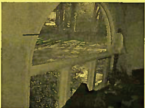
Insulated glass seal has failed (glass fogged)
