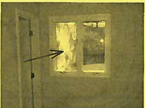
Insulated glass seal has failed (glass fogged)
