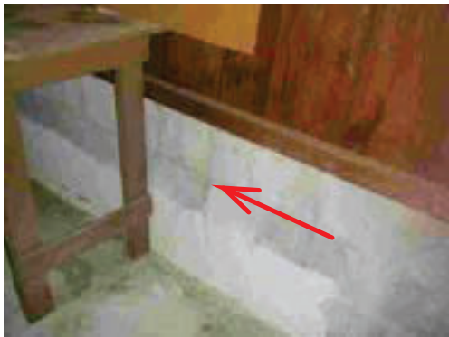
Stress crack in block wall of garage
