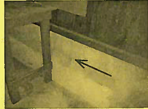
Stress crack in block wall of garage
