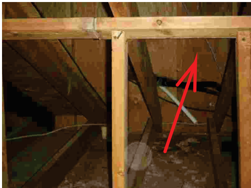
Vertical wall in sunroom is missing insulation
