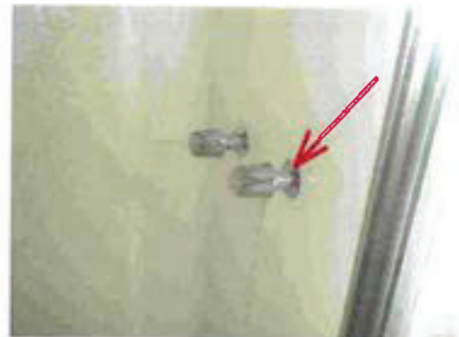
Master shower valve stems are leaking
