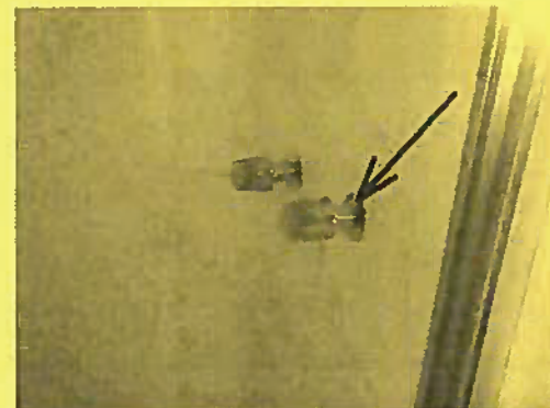
Master shower valve stems are leaking
