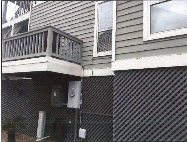
UNIT 1-B MARINERS CAY DRIVE SIDE -LEFT NOTE: ONE METER FOR BUILDING
