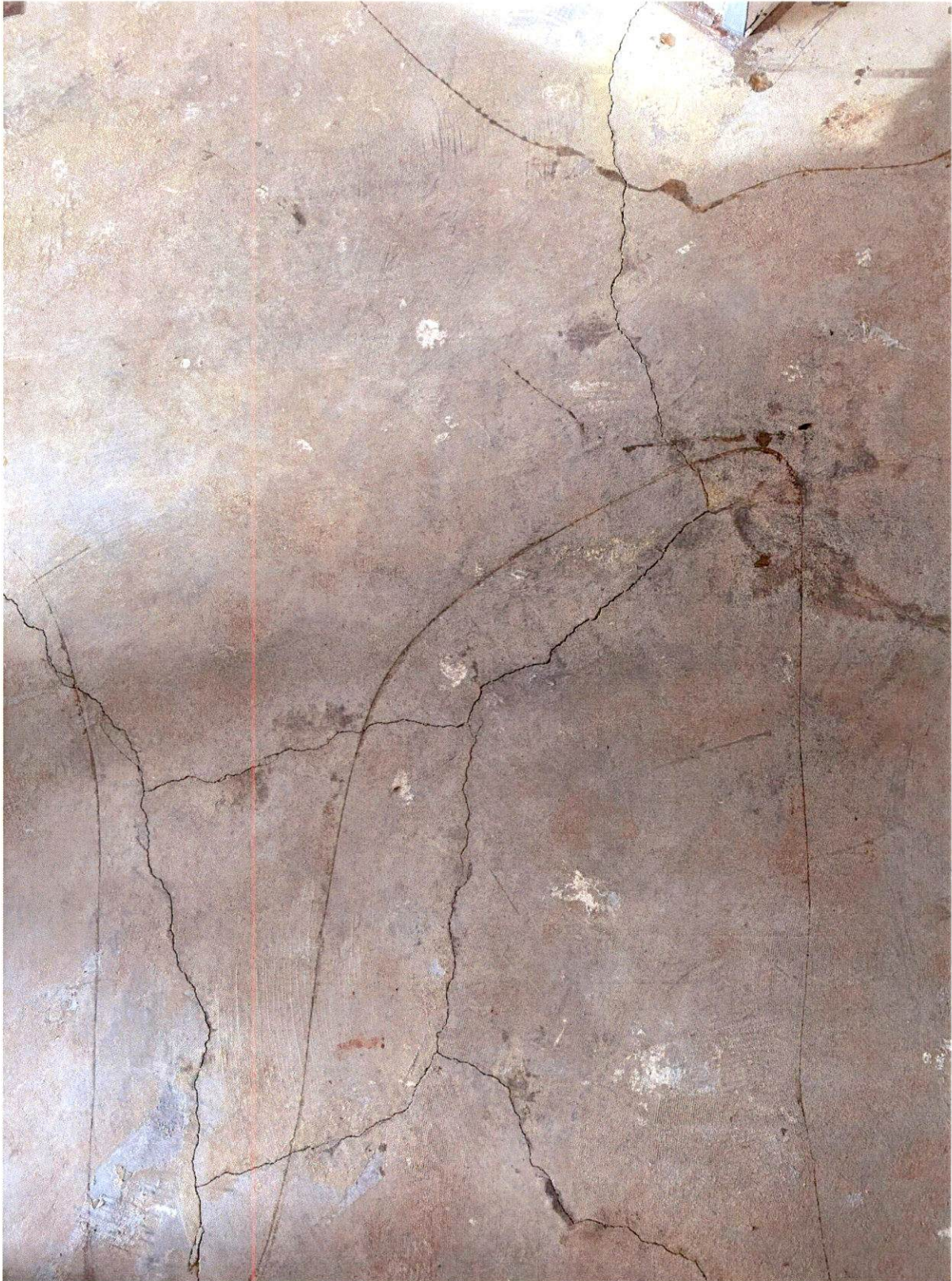
Picture 33: Substrate not smooth, free of old paint and old adhesive. Products not rolled with a roller to create transfer
