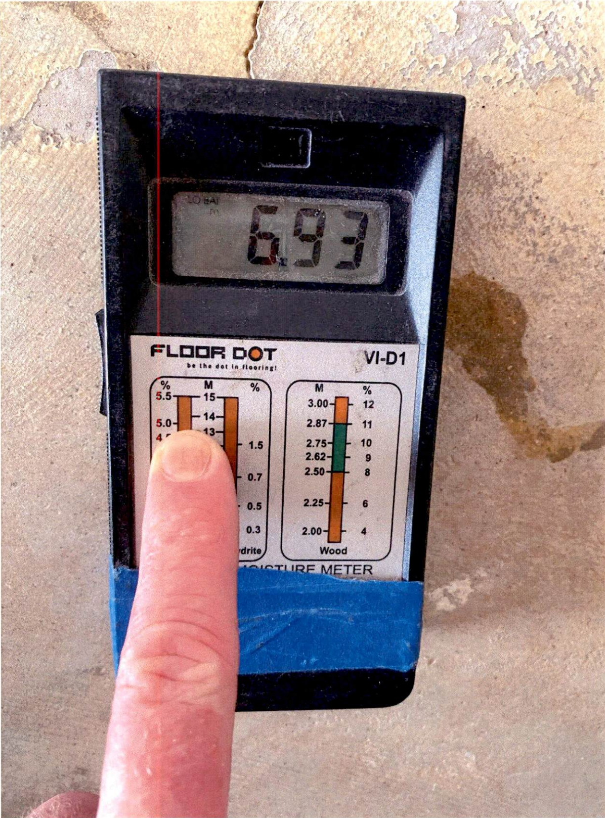
Picture 7: Family room: subfloor moisture
