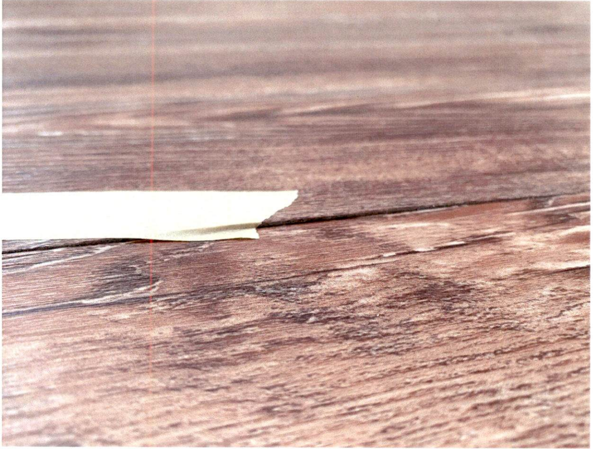
Picture 13: Continuously lifting throughout, severe tripping hazard
