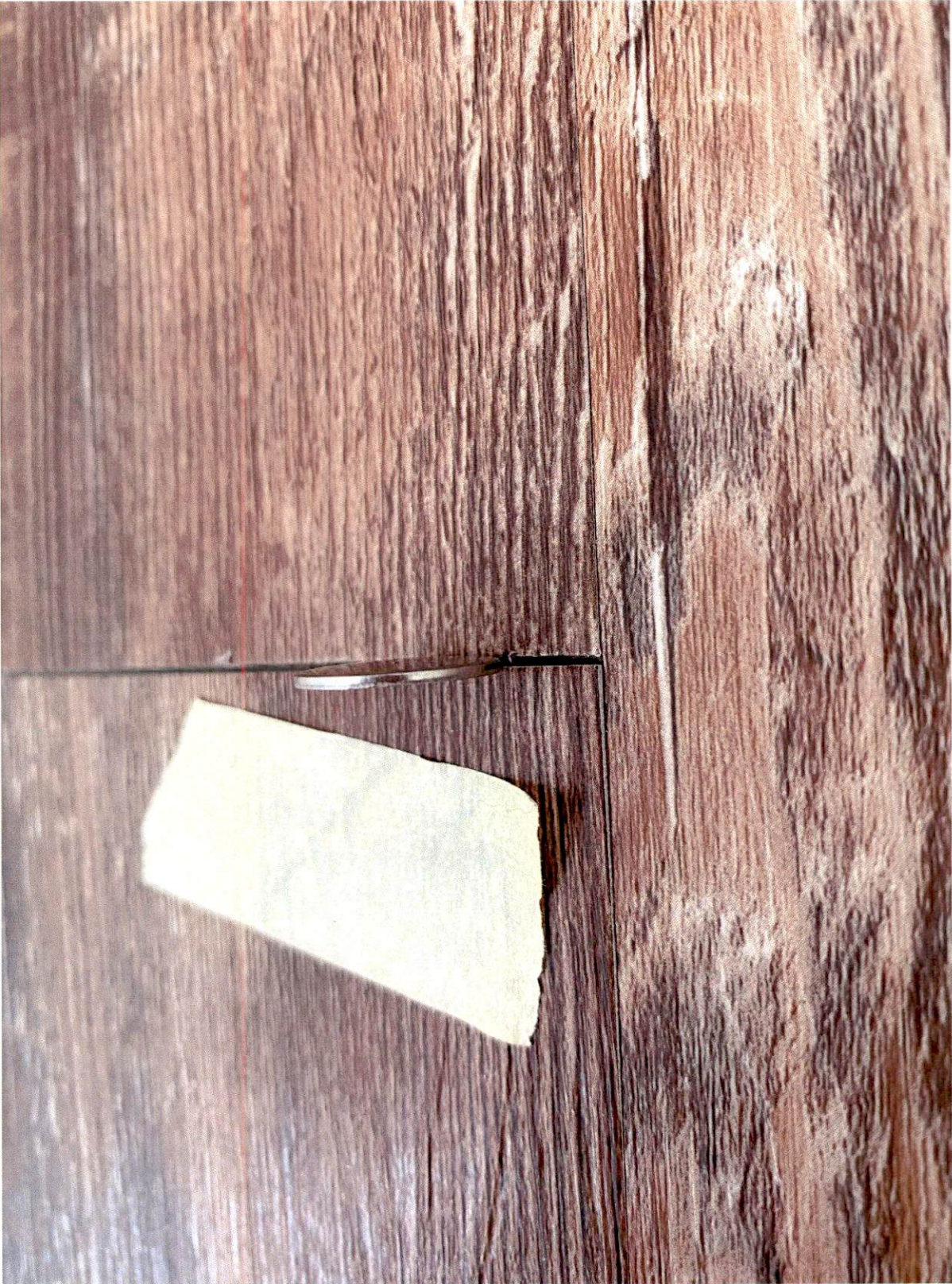
Picture 19: Butt-end joints gapped 1/16", not filled with adhesive
