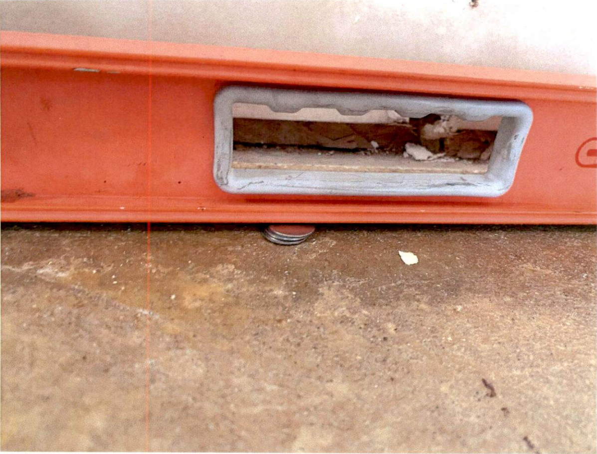
Picture 20: Subfloor not prepped: major deviations
