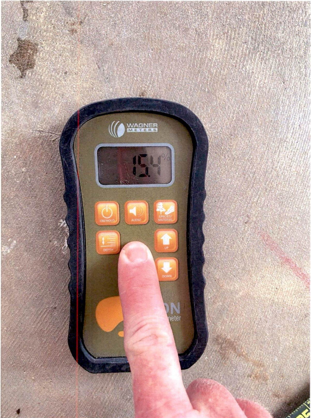
Picture 11: Family room: subfloor moisture
