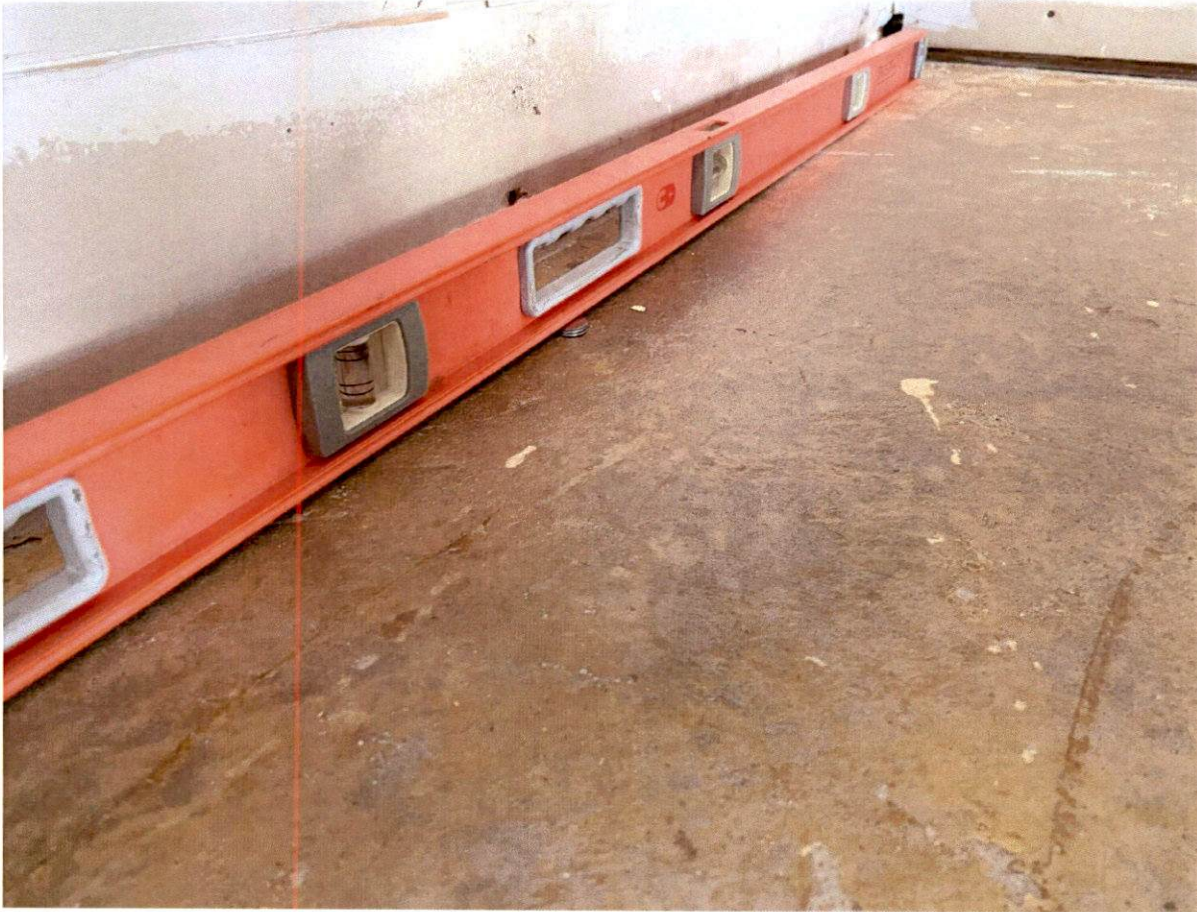
Picture 21: Subfloor not prepped: major deviations
