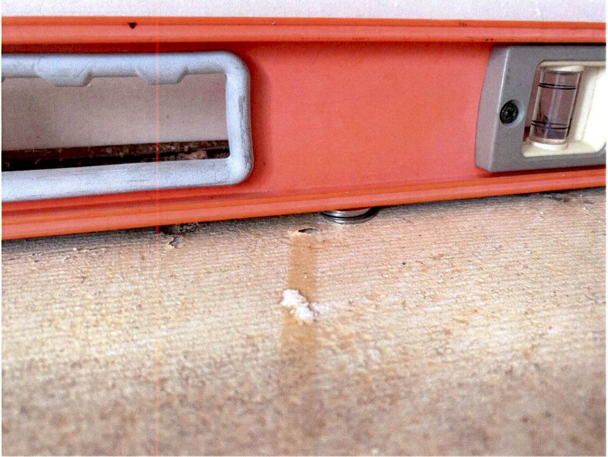
Picture 25: Sub-floor not prepped: major deviations
