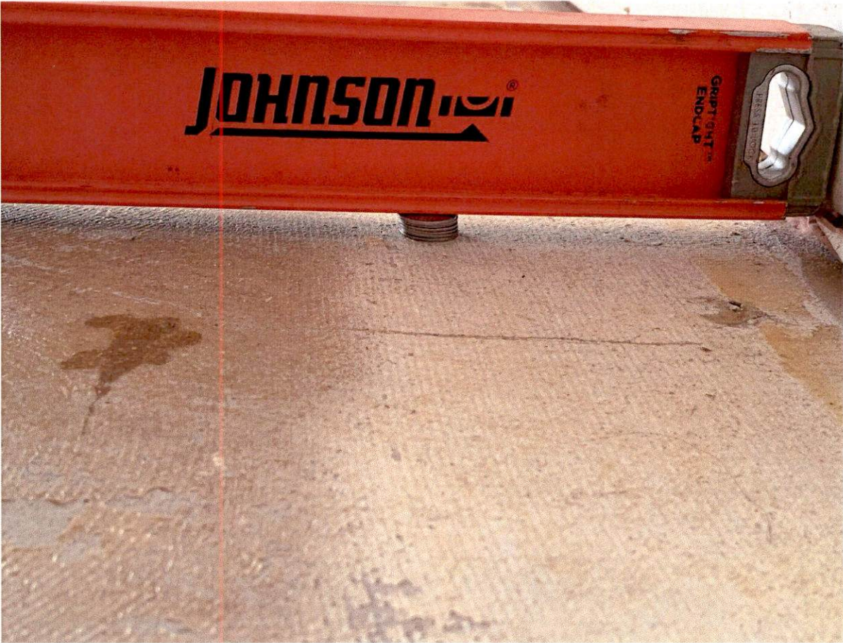
Picture 26: Sub-floor not prepped: major deviations not filled, old paint not removed
