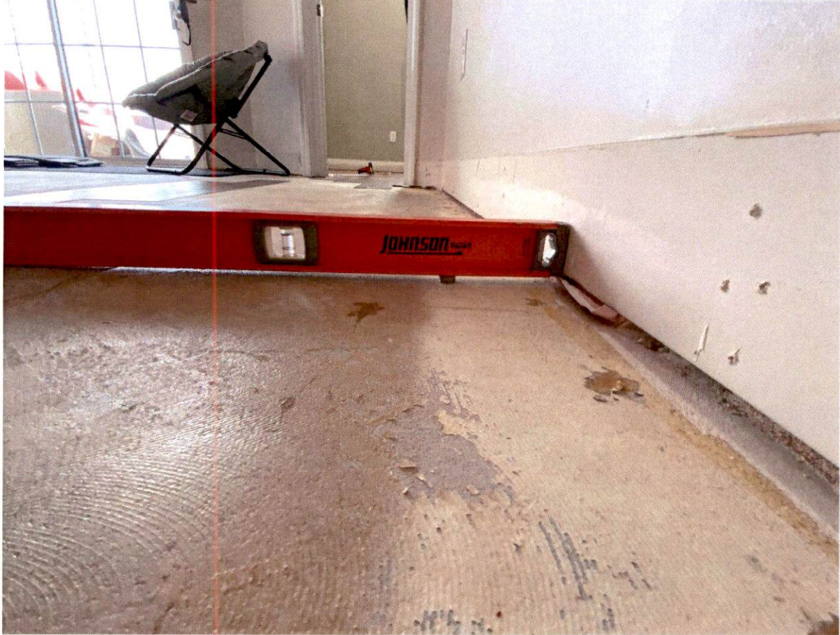
Picture 27: Sub-floor not prepped: major deviations not filled, old paint not removed
