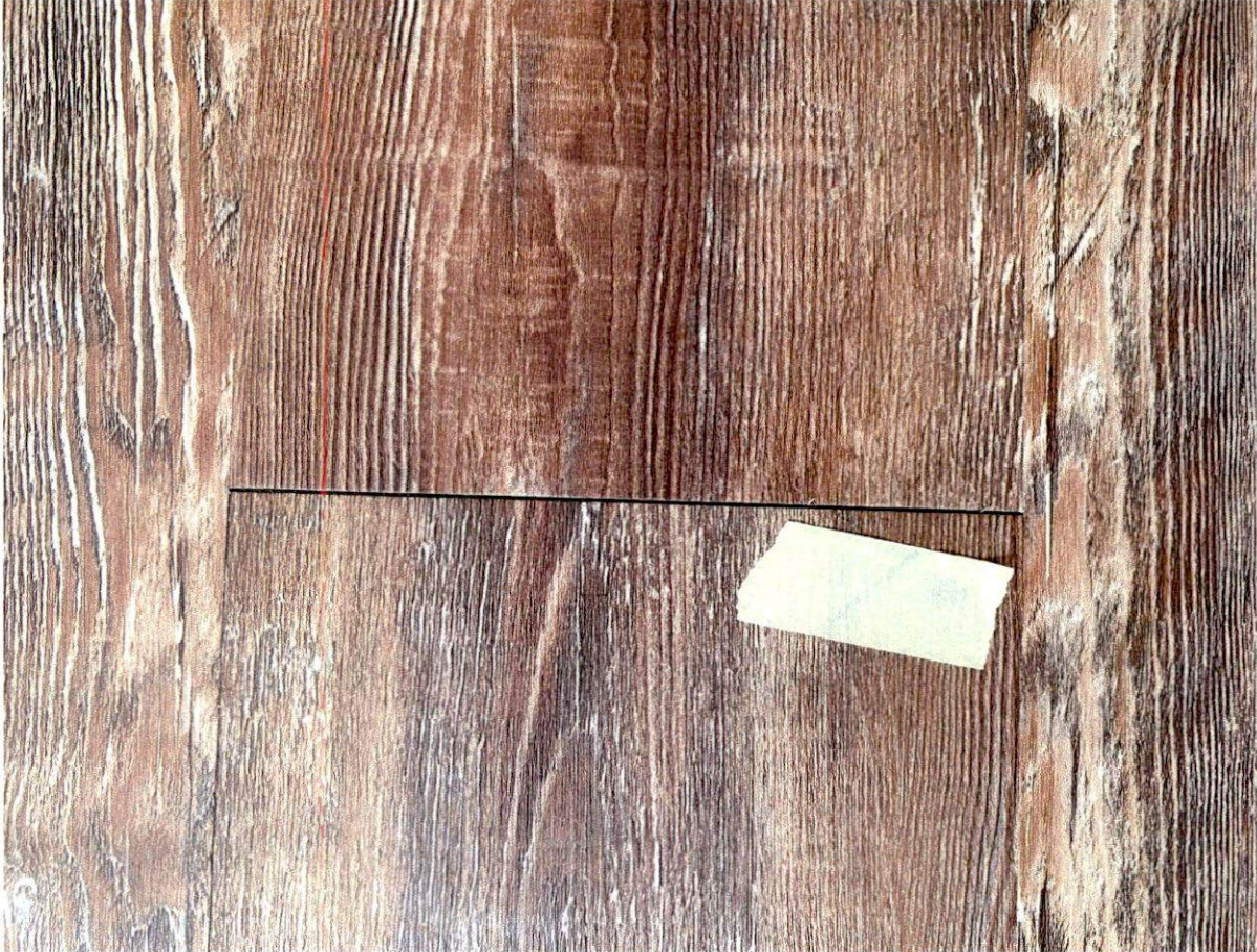
Picture 17: Butt-end joints gapped 1/16", not filled with adhesive
