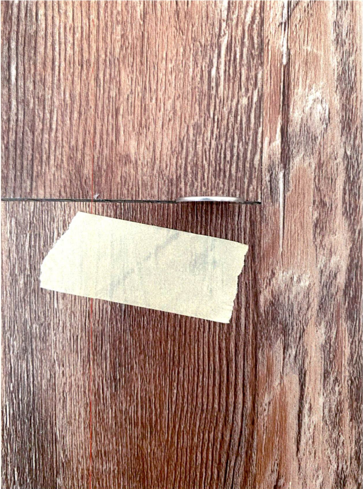
Picture 18: Butt-end joints gapped 1/16", not filled with adhesive
