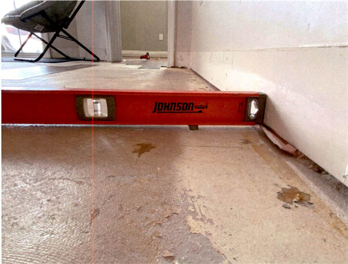
Picture 28: Sub-floor not prepped: major deviations not filled, old paint not removed
