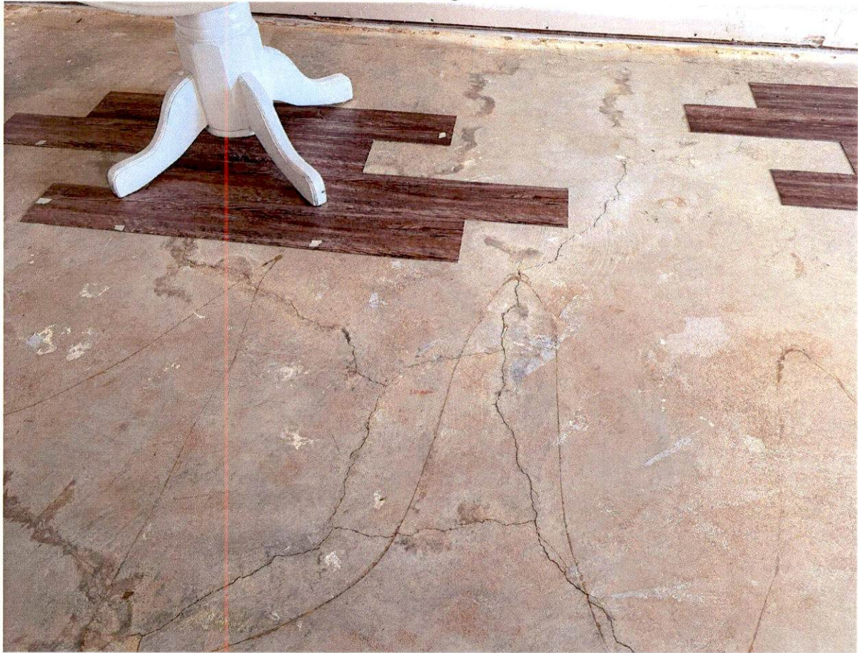
Picture 2: Porous and cracked subfloor absorbed glue
