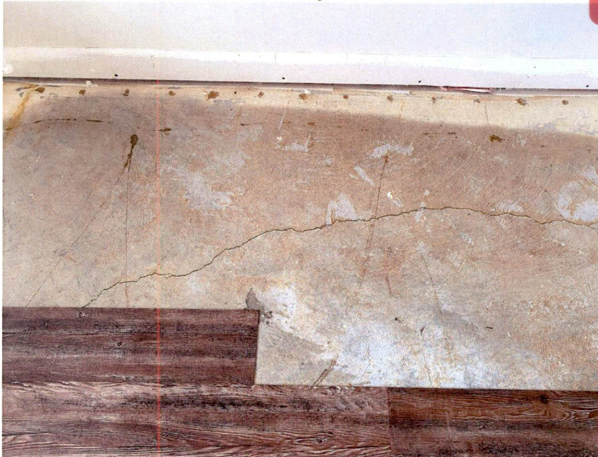
Picture 1: Porous and cracked subfloor absorbed glue
