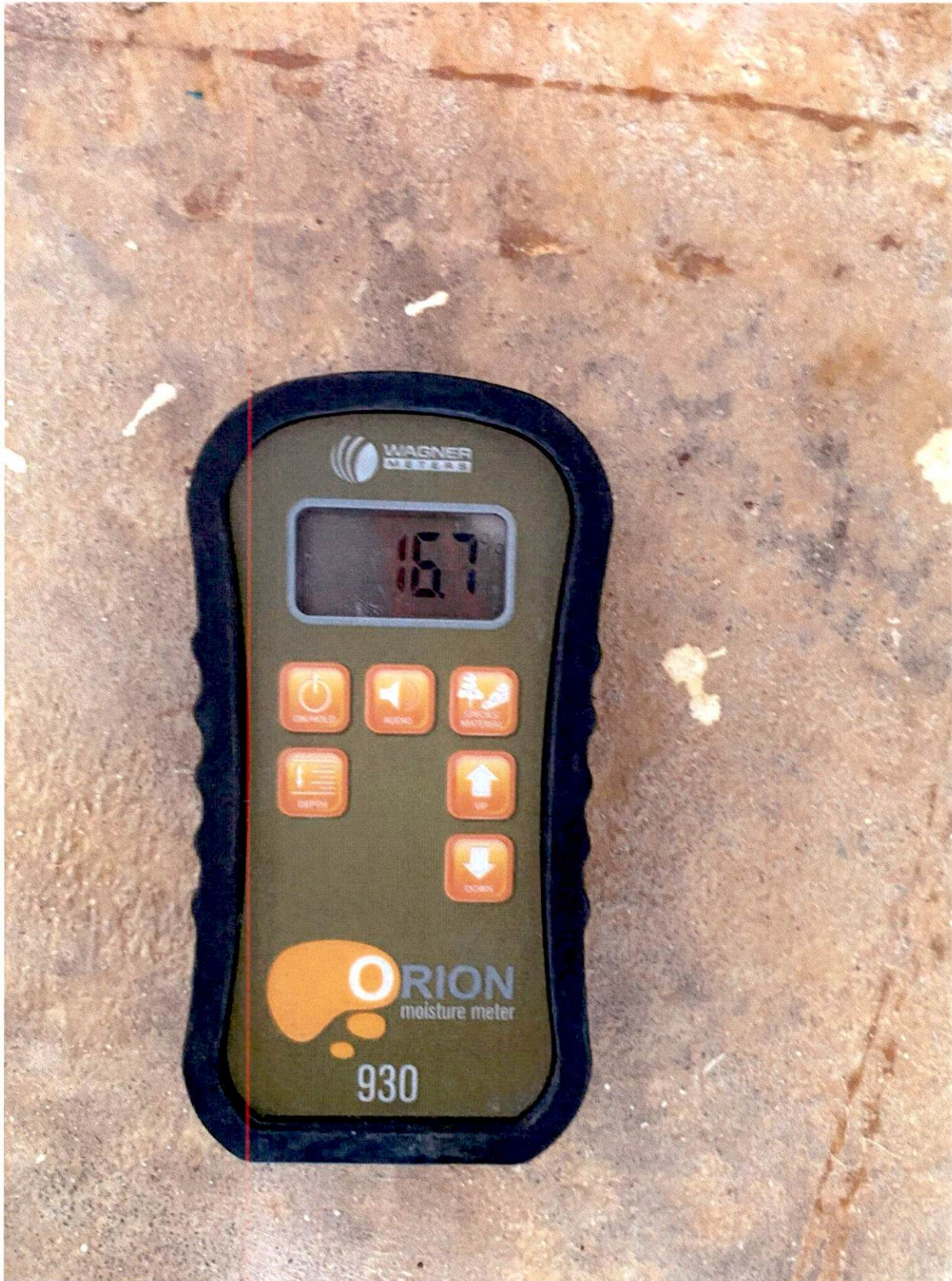
Picture 23: Excessive moisture in front corner of family room
