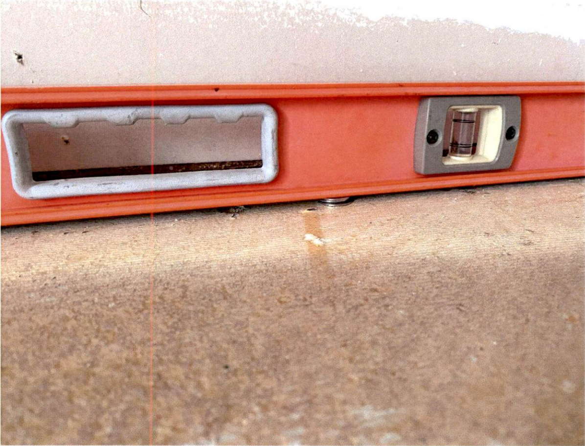
Picture 24: Sub-floor not prepped: major deviations
