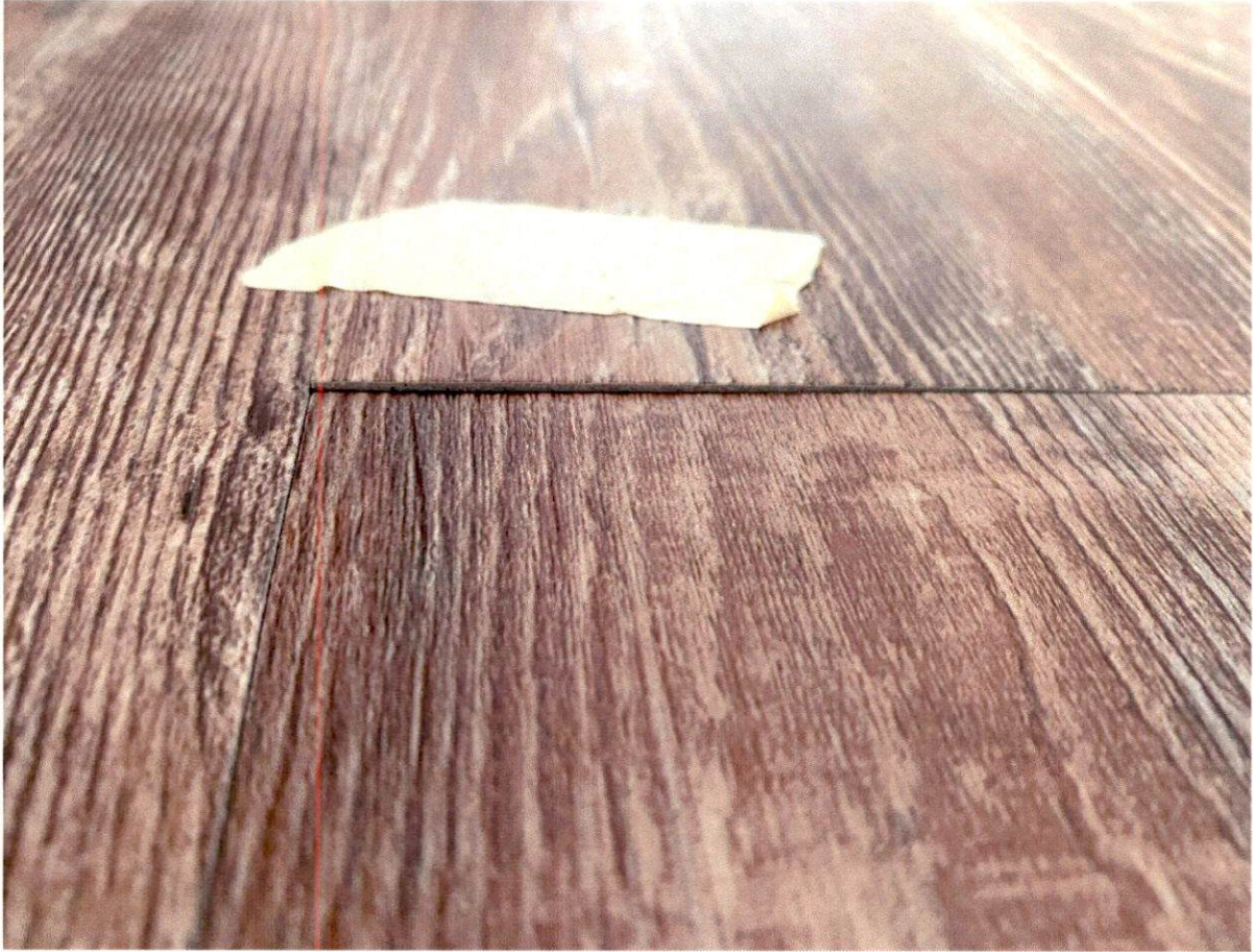
Picture 15: Continuously lifting throughout, severe tripping hazard
