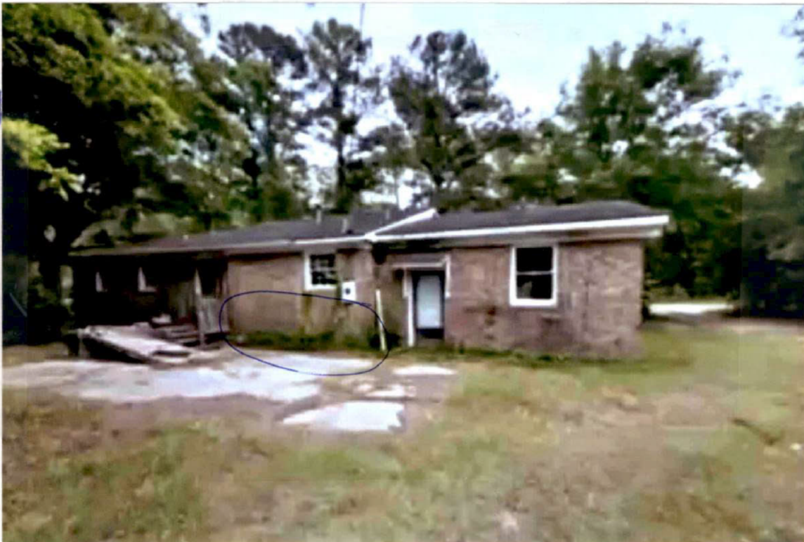
Main House Rear HVAC missing Ramp Destroyed
