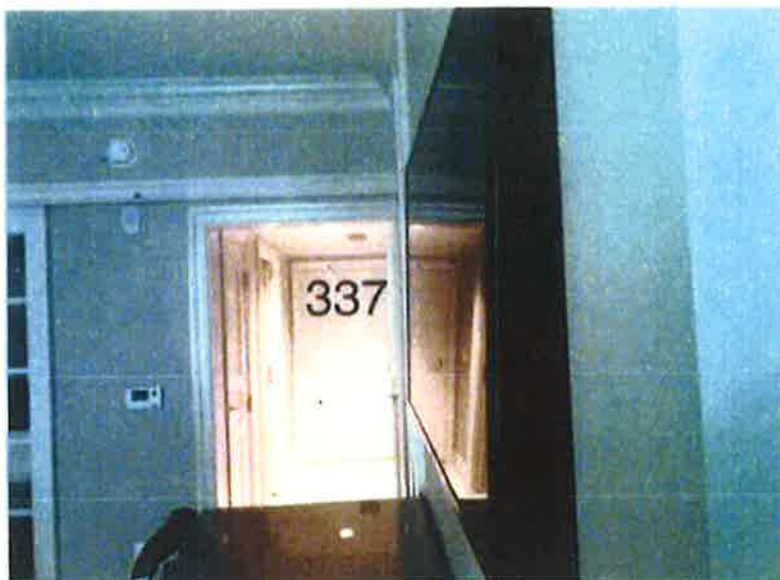
Owner LV Contractor installing TV out of plumb
