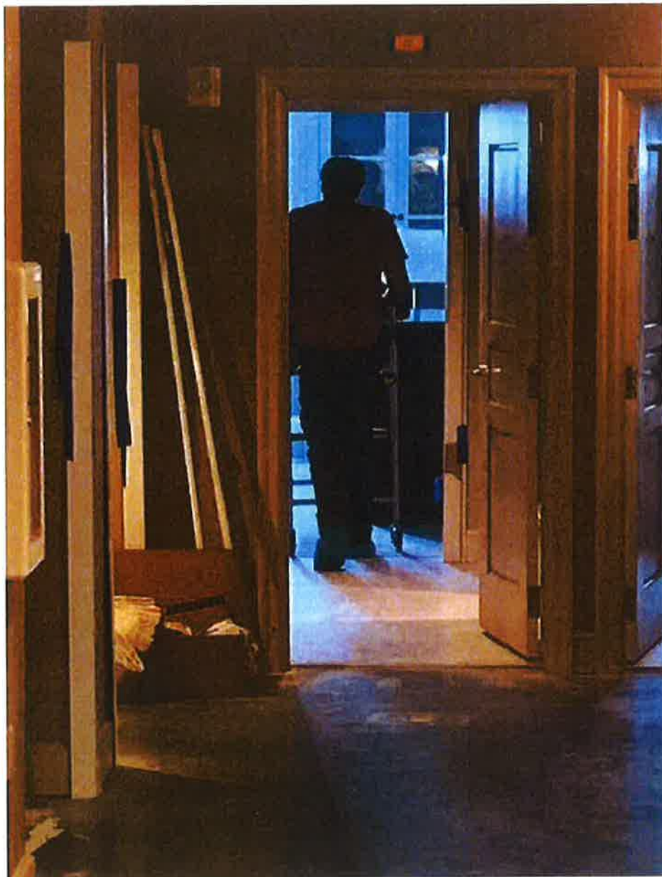
Owner installing Drapes with no protection on equipment and drape rods leaning Against Walls with no protection.
