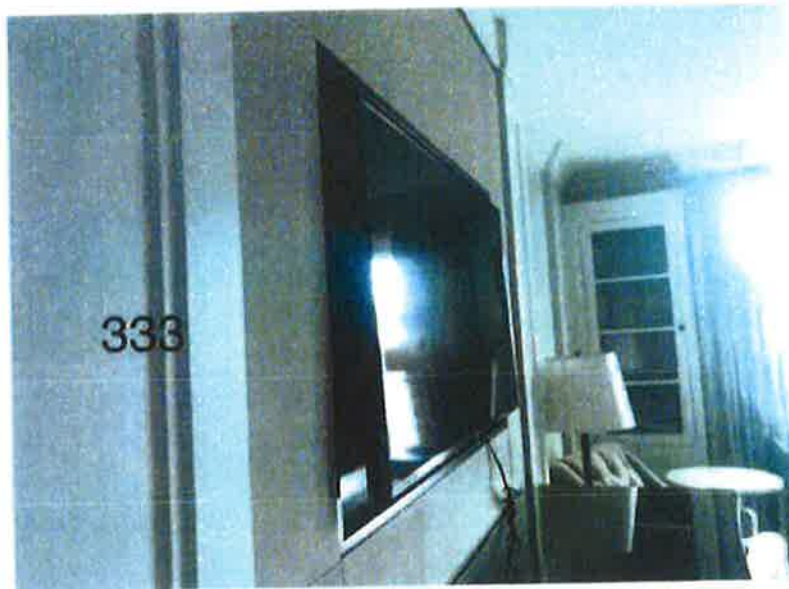
Owner Install of tv after install of dimmers. TV kicked out at bottom
