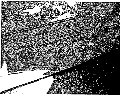
Damaged paint in master bedroom window.
