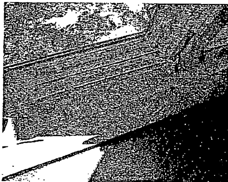
Damaged paint in master bedroom window.
