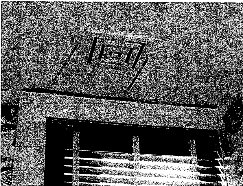
PHOTO 6B: View of mildew/mold on ceiling in media room bathroom, above window trim.
