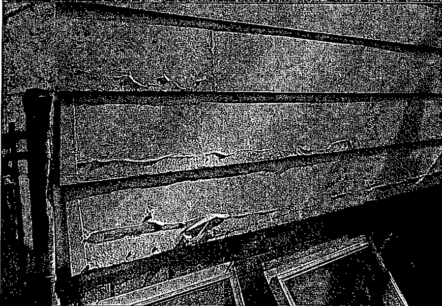
8391 Winnsboro Road DETERIORATING SIDING
