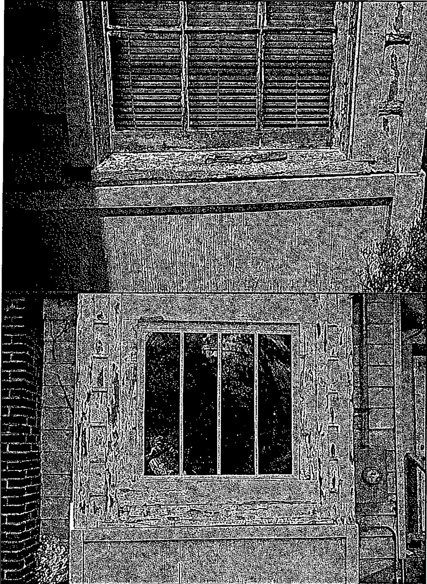
4824 Linden Street PEELING PAINT
