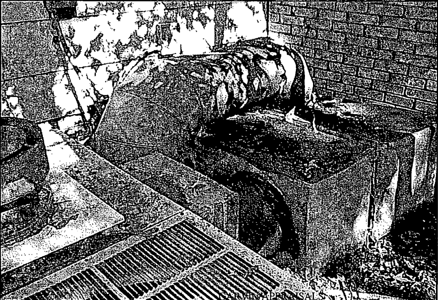
8391 Winnsboro Road HVAC SYSTEM
