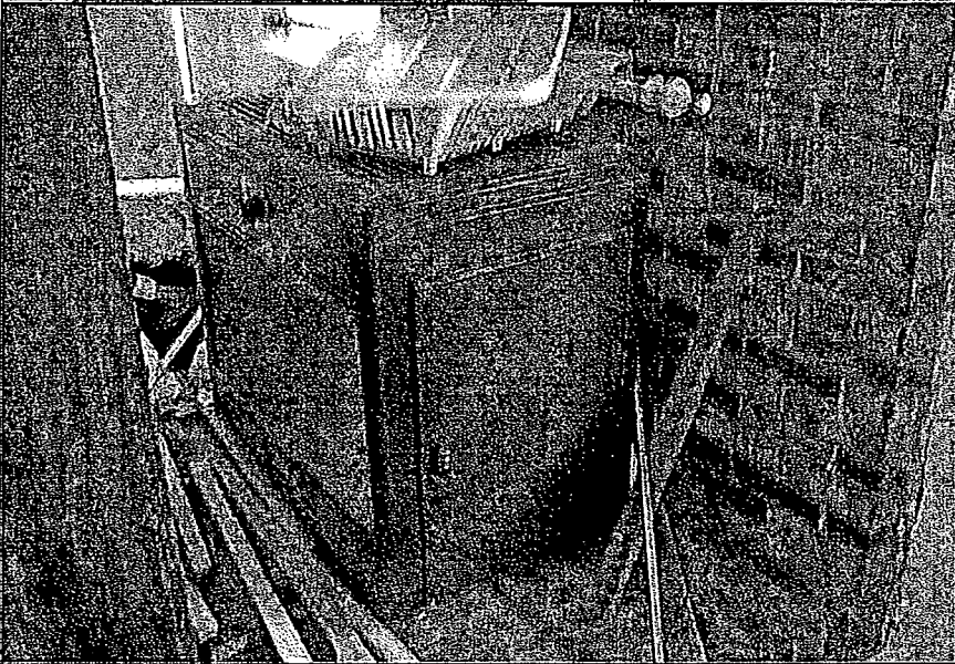
8391 Winnsboro Road HEATING SYSTEM IN LR
