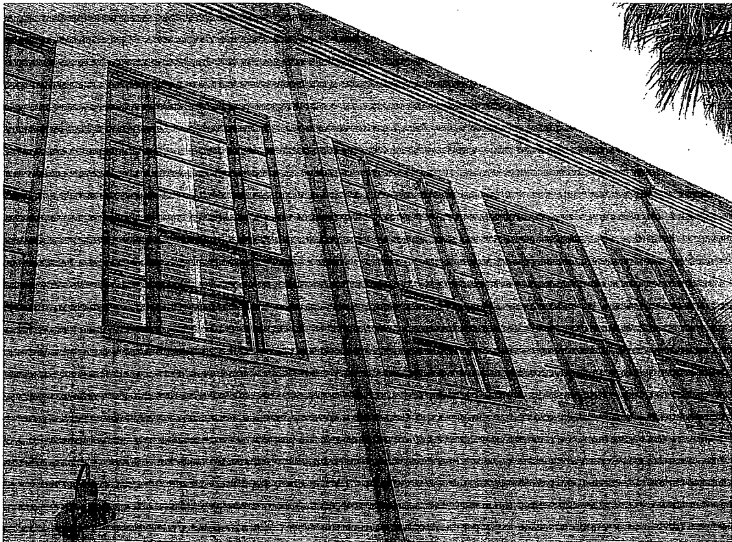
Figure 2 illustrates the typical wood windows installed at the facility. The subject photo was taken looking along the second story of the gymnasium building's north elevation.
