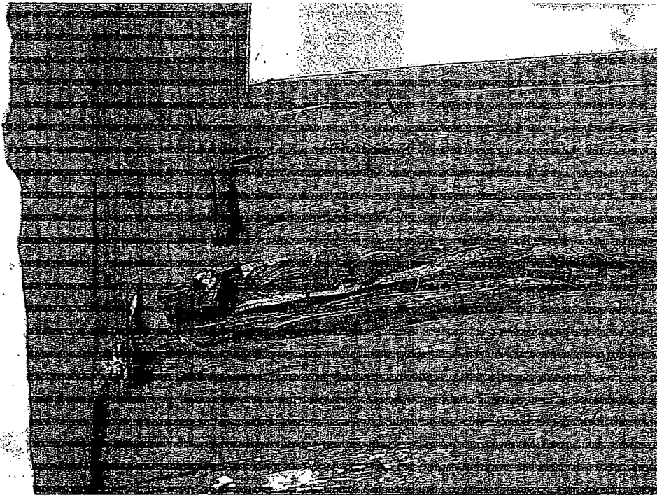
Figure 4 illustrates the severity of the wood decay on some of the windows identified as “new windows to match existing” on the architectural plans.
