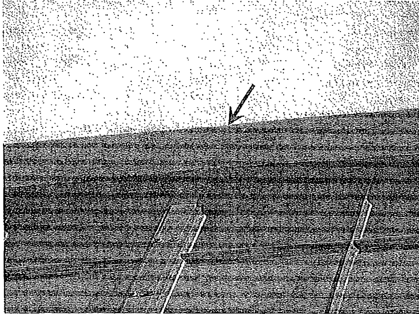
Figure 1: Staining visible in the stucco along the window head. No evidence of a drip screed/through-wall flashing was visible at the vertical to horizontal stucco transition (red arrow).
