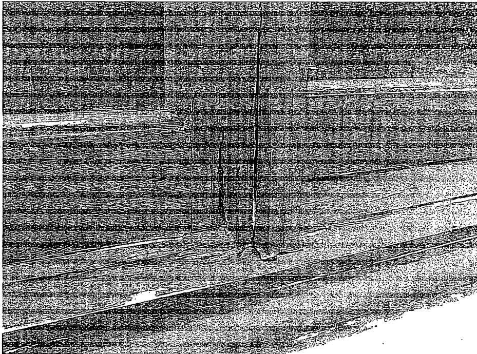
Figure 3 reveals the decay observed along the majority of the wood window frames at the subject facility.
