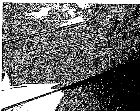
Damaged paint in master bedroom window.
