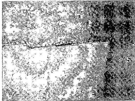
Figure 30-Grout voids, office shower
