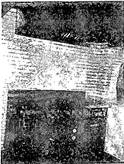
Figure 27-Caumartin gas range and commercial style hood
