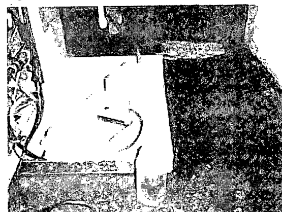
Figure 46-Closeup of previous figure: water on crawlspace floor
