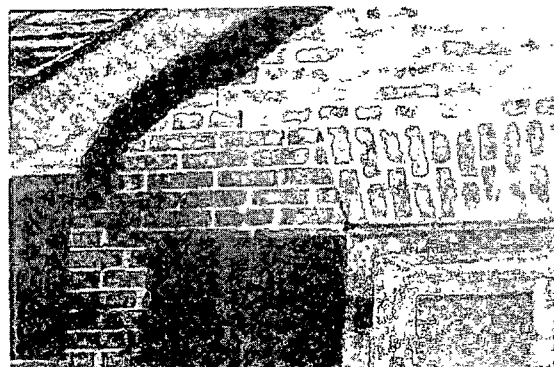
Figure 22-Closeup of previous figure: minor settlement
