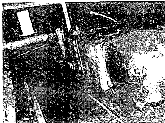
Figure 42-Attic furnace: above service wing
