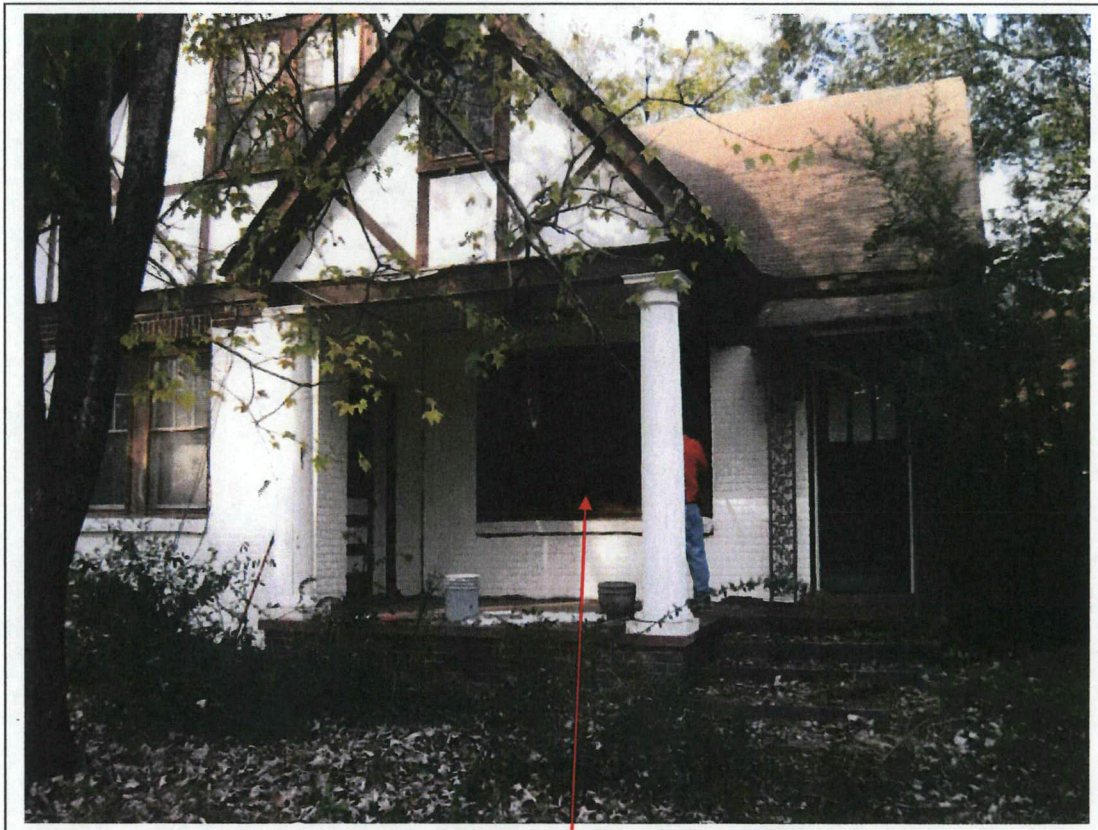
Windows removed without approval or permits.
