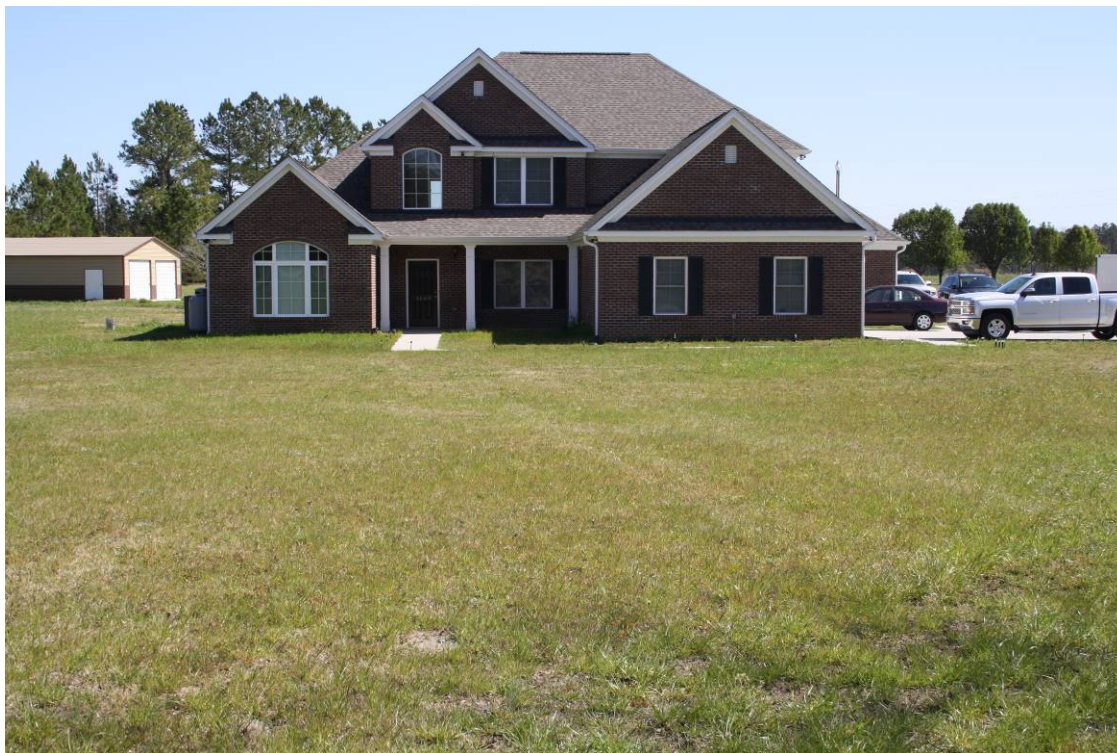
Figure 1. A front view of the residence looking northeast. Note: The residence is constructed in a depression and there is improper grading away from the building in violation of the building codes.
