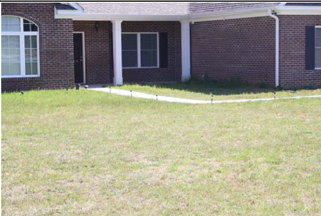
Figure 8. A closer view of the front entrance. Note: The residence is constructed in a depression and there is improper grading away from the building in violation of the building codes. The original plans called for a raised porch with steps.
