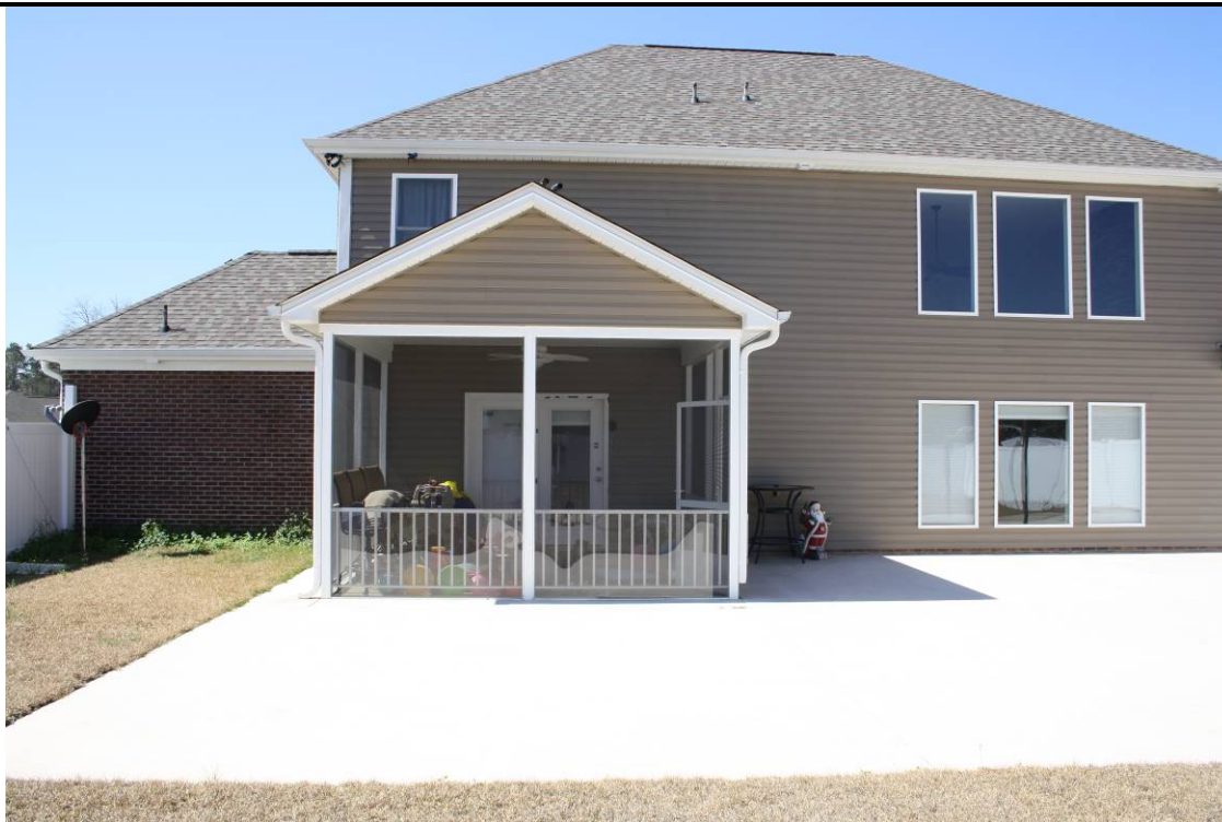
Figure 2. A rear view of the residence looking southwest. Note: The slab and rear yard are flat with minimal grading away from the building.
