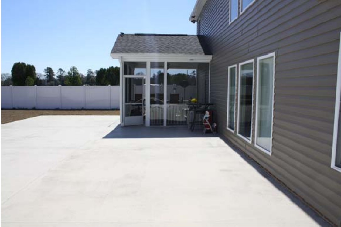
Figure 3. A rear view of the residence looking northwest. Note: The slab and rear yard are flat with minimal grading away from the building.
