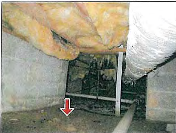
7.6 Item 3(Picture) Missing vapor barrier - damp ground
