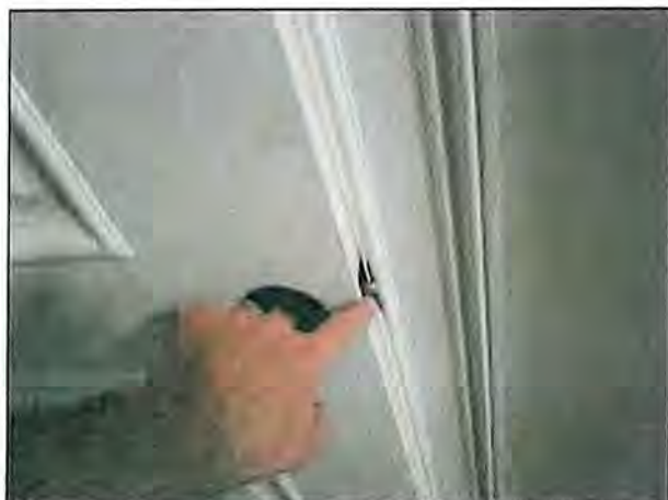
5.4 Item 1(Picture) Door does not latch
