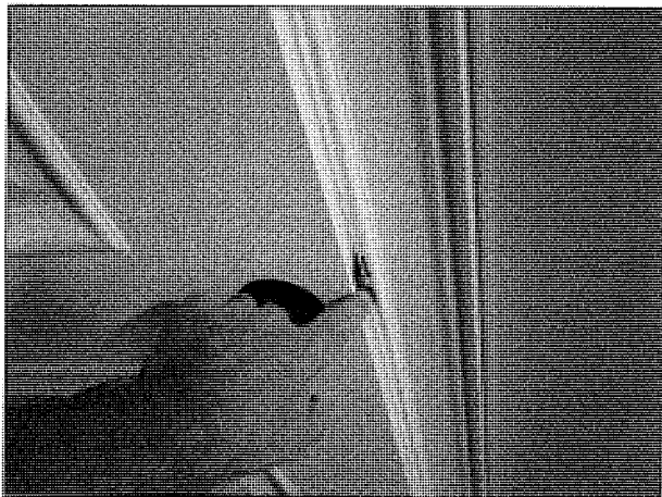
5.4 Item 1(Picture) Door does not latch
