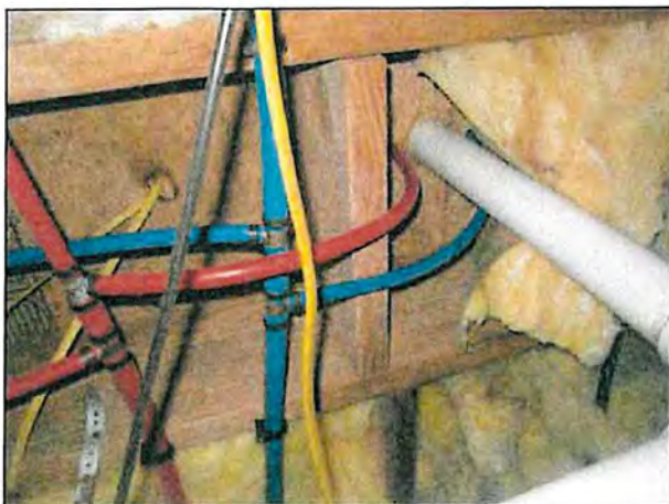
7.5 Item 3(Picture) Missing insulation
