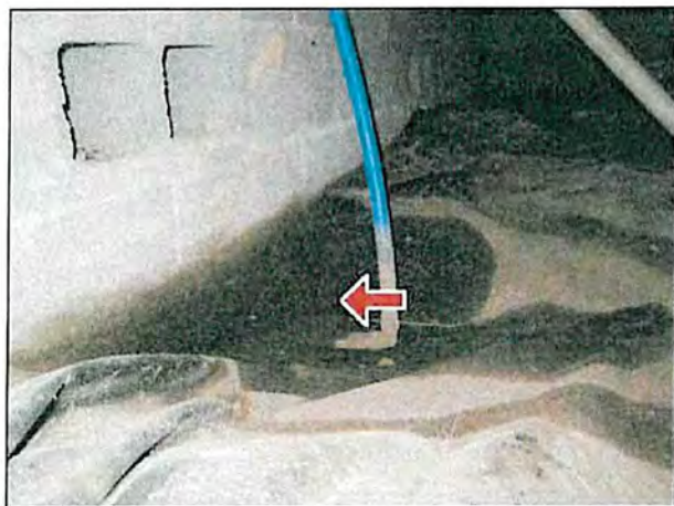
7.6 Item 1(Picture) Dampness in crawl space
