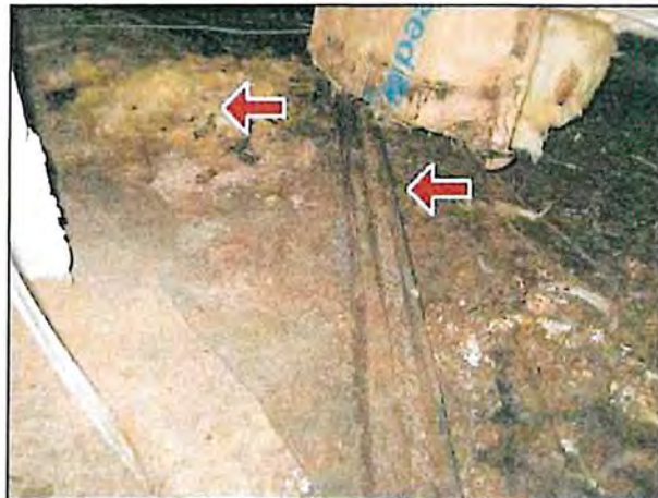
7.6 Item 4(Picture) Wet debris on top of vapor barrier
