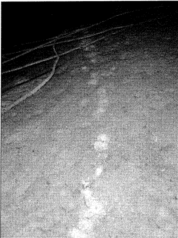
7.6 Item 5(Picture) Missing vapor barrier - damp ground
