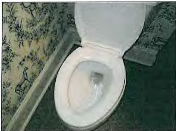
6.7 Item 1(Picture) Toilet will move/tip when pushed
