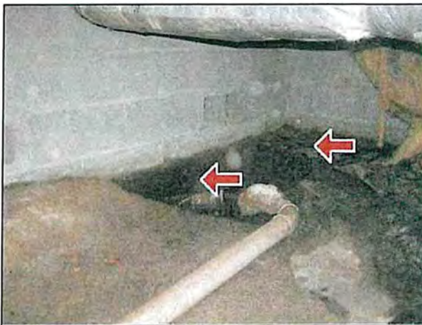
7.6 Item 2(Picture) Dampness in crawl space - missing vapor barrier
