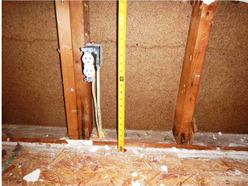
Photo 14 – Waterline stain mark on the inside of the fiber board exterior wall sheathing at approximately 16- to 17-inches above the subfloor. Photo by ABS taken 12/13/2018.
