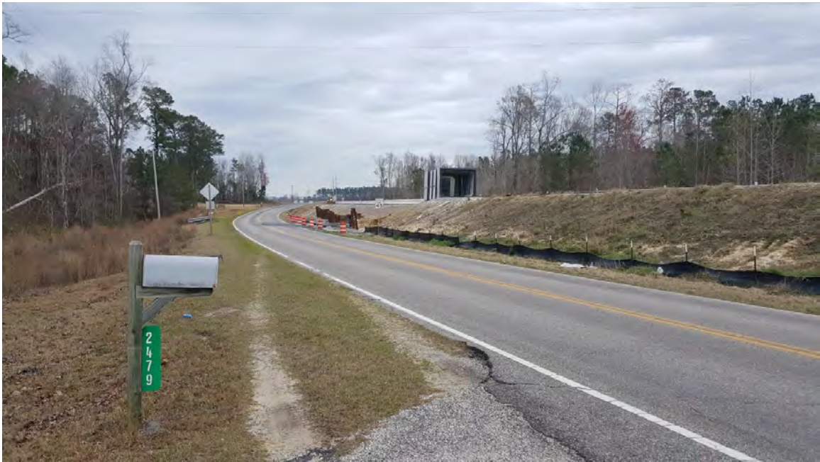
Photo 6 – This construction photo depicts the new roadbed substantially higher in elevation than the existing road in front of the Marlowe property, looking east. Photo provided by Hopkins Law Firm.
