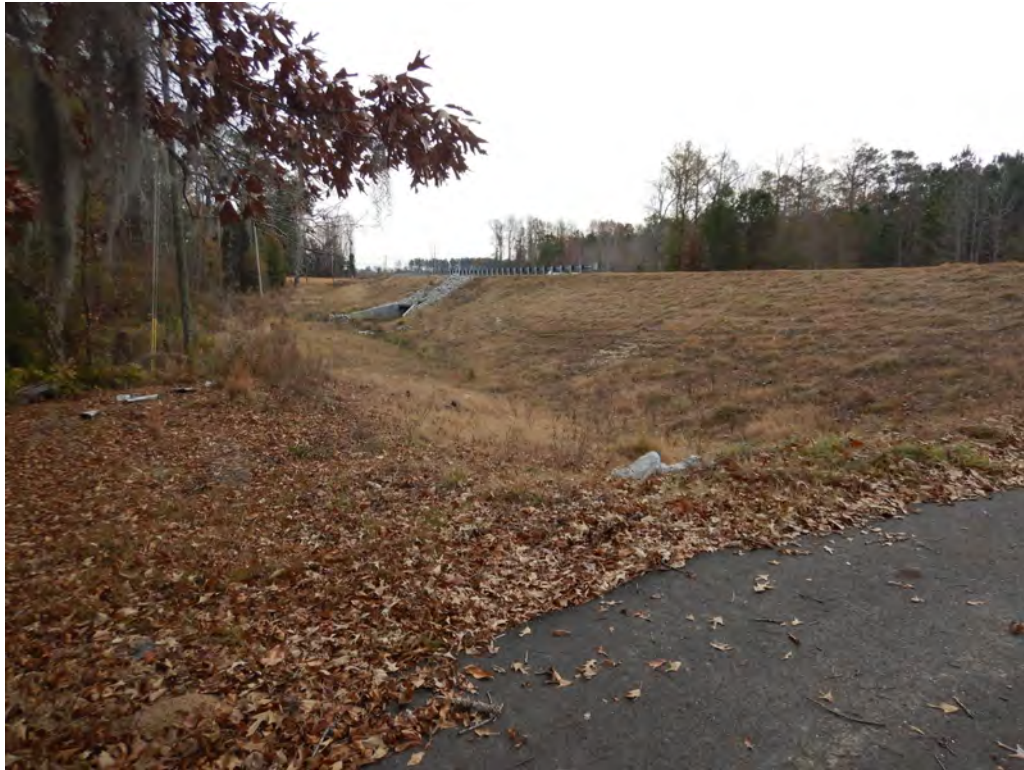
Photo 23 – View of the culvert inlet as seen from the Marlowe driveway. Photo by ABS taken 12/13/2018.
