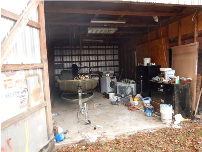
Photo 18 – Waterline staining on the rear shed was measured to extend 6'-0" to 6'-4" above the ground surface. Photo by ABS taken 12/13/2018.
