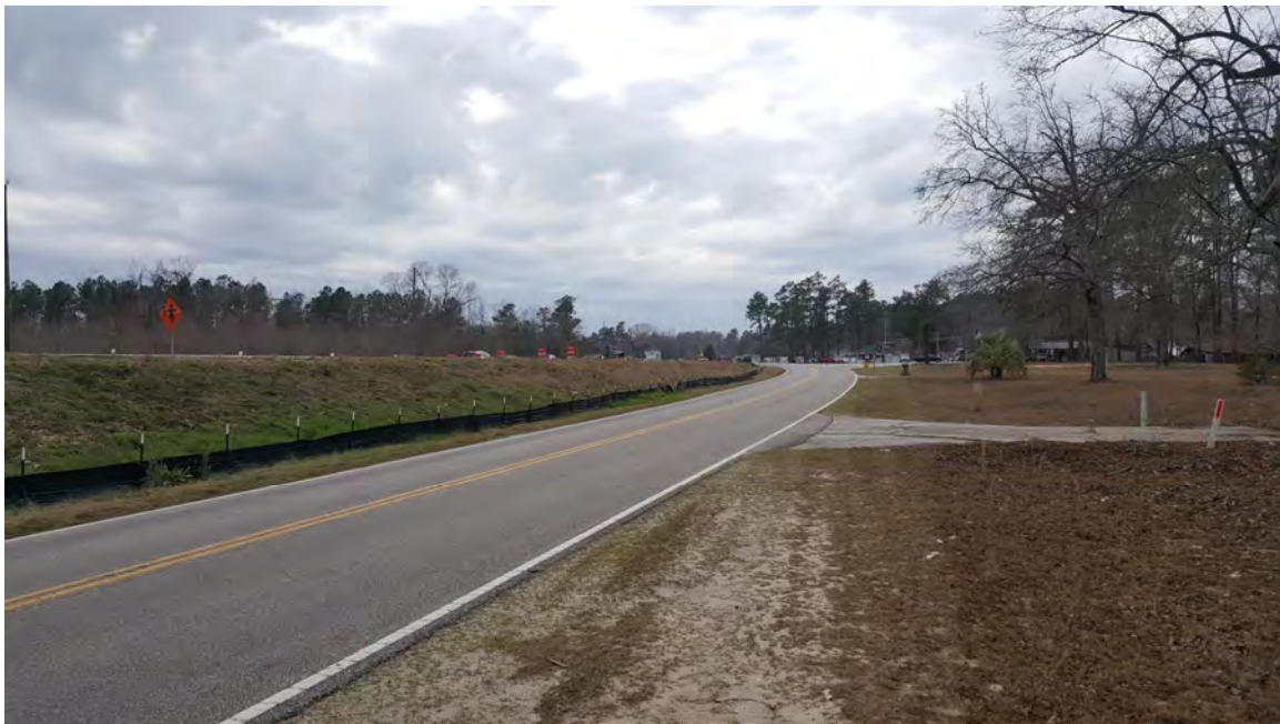
Photo 7 – This photo taken during construction depicts the new roadbed substantially higher than the existing road in front of the Marlowe property, looking west. Photo provided by Hopkins Law Firm.
