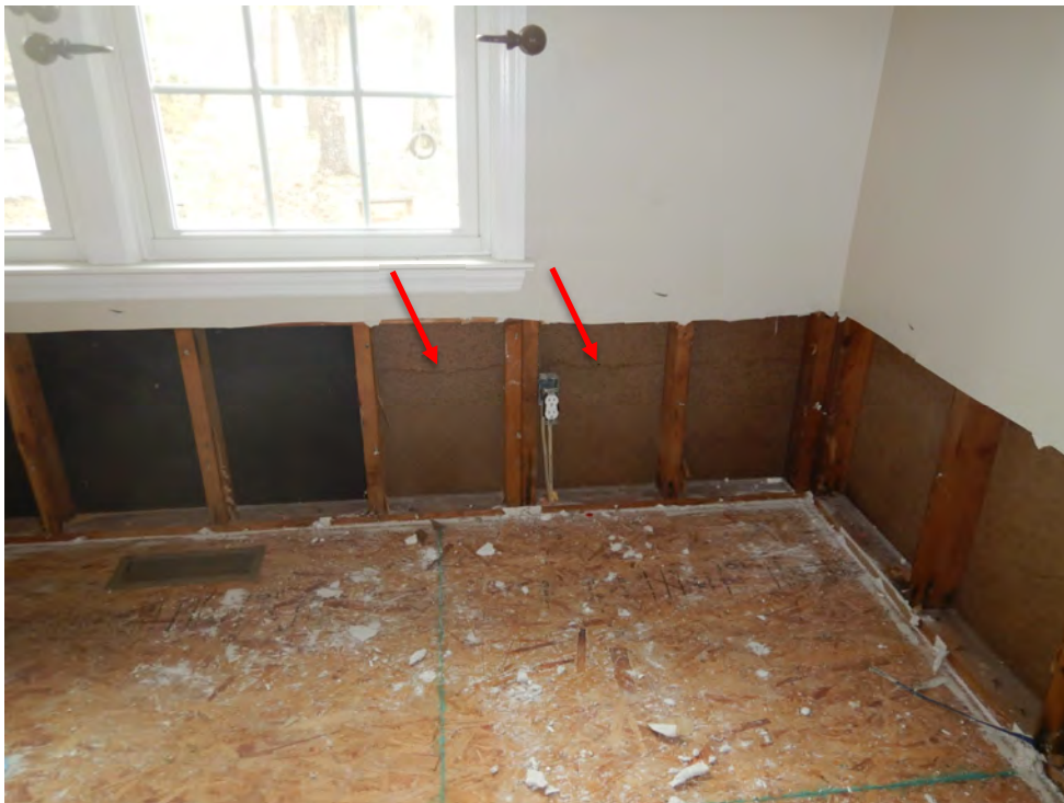
Photo 13 – Interior conditions at the subject residence with the waterline stain indicated. Photo by ABS taken 12/13/2018.
