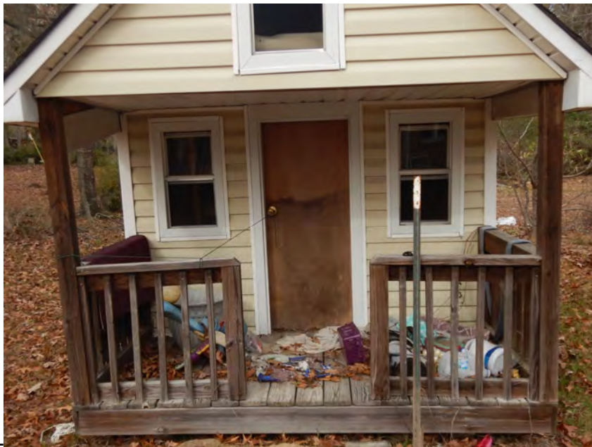
Photo 19 – Waterline staining on the door of an accessory structure. Photo by ABS taken 12/13/2018.
