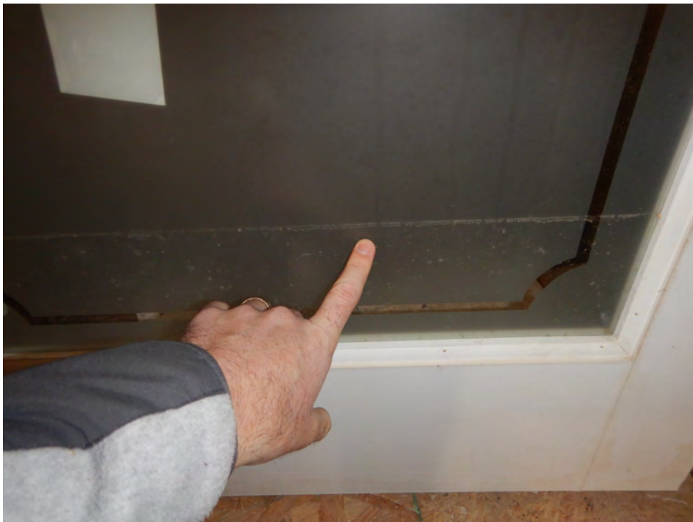
Photo 11 – Water stain mark on a glass door panel. Photo by ABS taken 12/13/2018.
