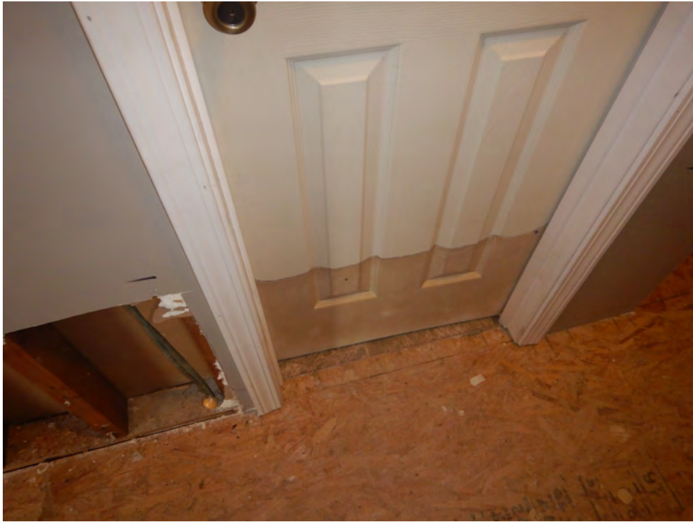
Photo 12 – Water stain mark on an interior door panel. Photo by ABS taken 12/13/2018.
