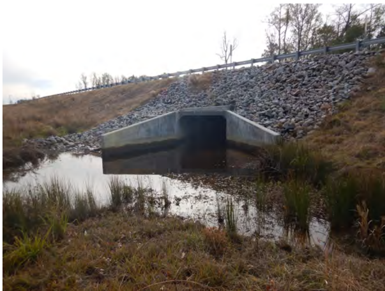
Photo 24 – Closer view of the culvert inlet at the subject stream crossing with US 378. Photo by ABS taken 12/13/2018.
