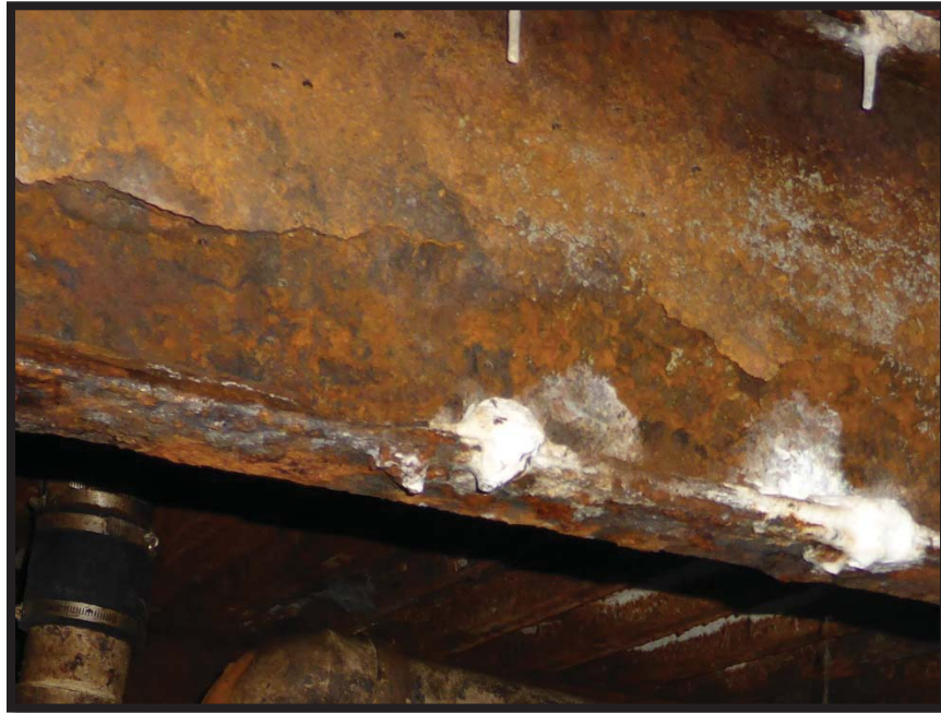
Photo 9: Severe Rust, Deterioration, and Delamination Observed on Joist Support Beam
