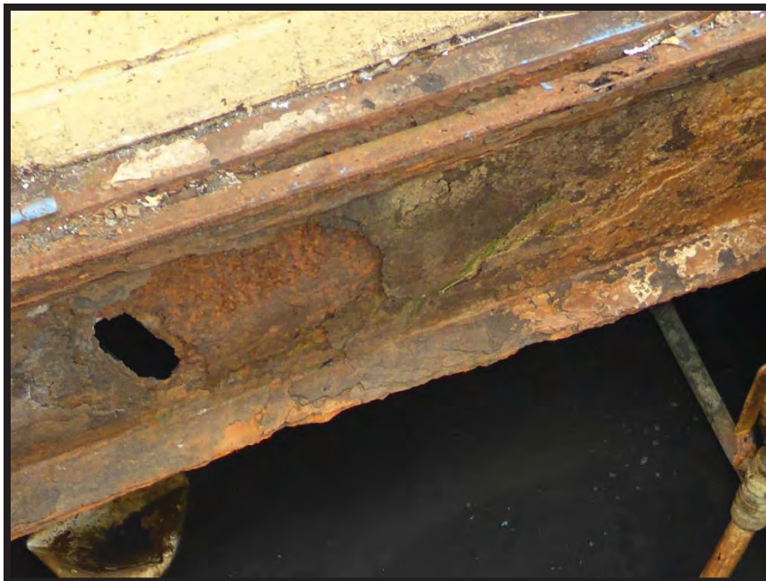
Photo 10: Severe Rust, Deterioration, and Delamination Observed on Perimeter Support Beam
