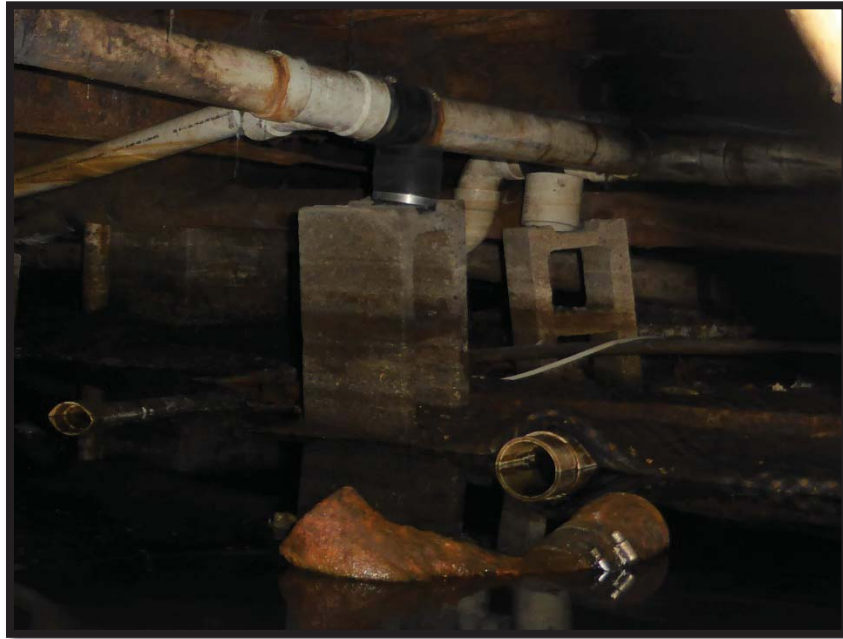
Photo 13: No Shoring Observed for Elevated Slab or Steel Frame
