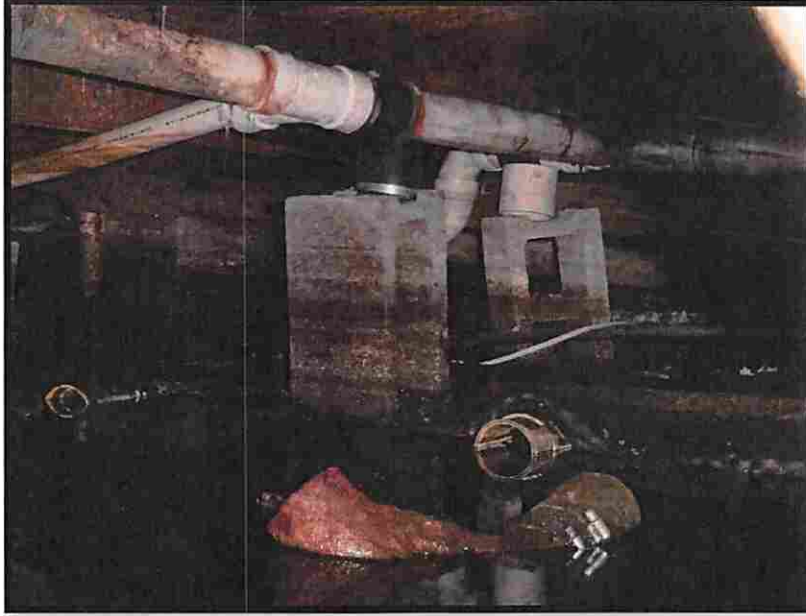
Photo 13: No Shoring Observed for Elevated Slab or Steel Frame
