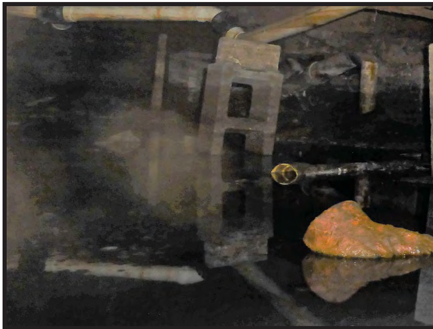
Photo 14: No Shoring Observed for Floor Decking
