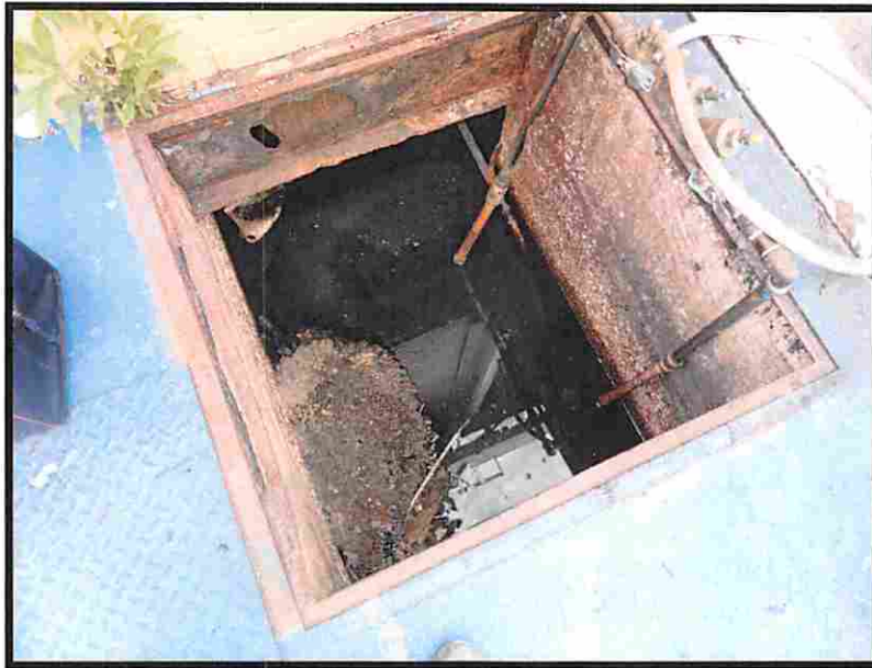
Photo 5: Standing Water at Entrance of Crawlspace
