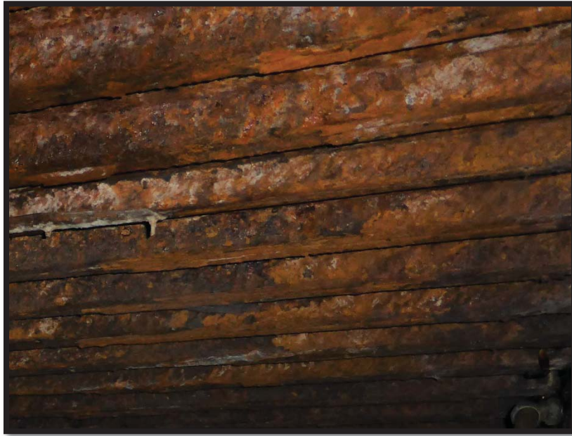
Photo 11: Observed Severe Rusting of Metal Decking, and Exposed Concrete
