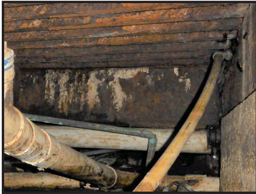
Photo 7: Rust, Deterioration, and Delamination Observed on Interior Girder Beam
