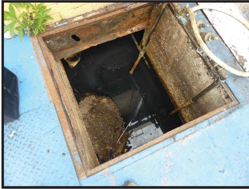
Photo 5: Standing Water at Entrance of Crawlspace
