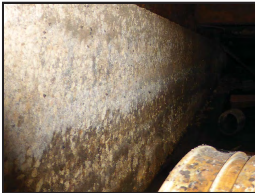
Photo 6: Evidence of Standing Water Observed on Perimeter Retaining Wall
