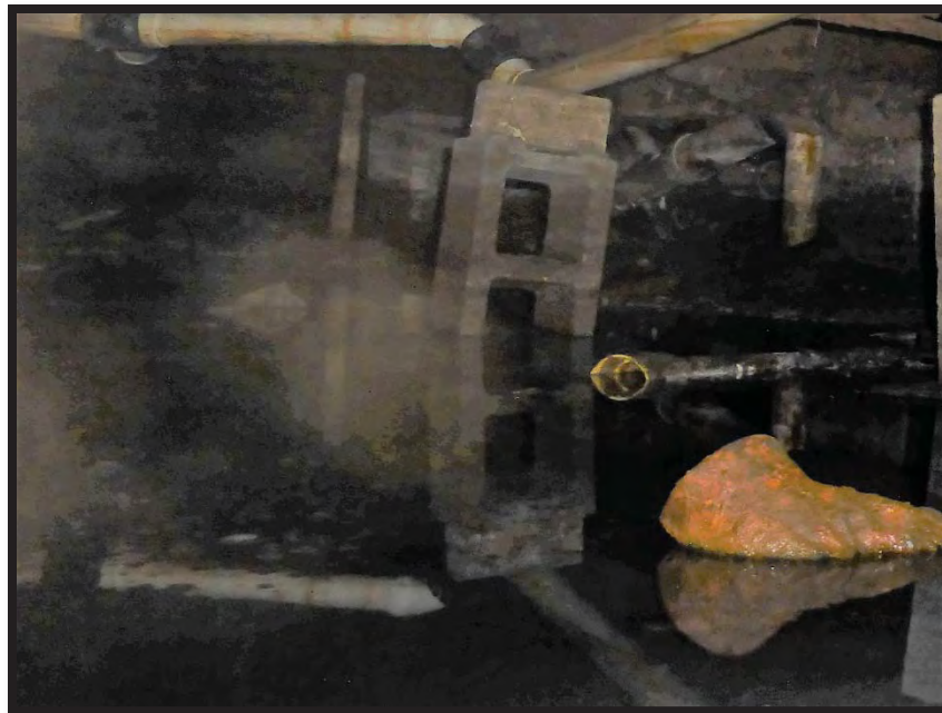
Photo 14: No Shoring Observed for Floor Decking
