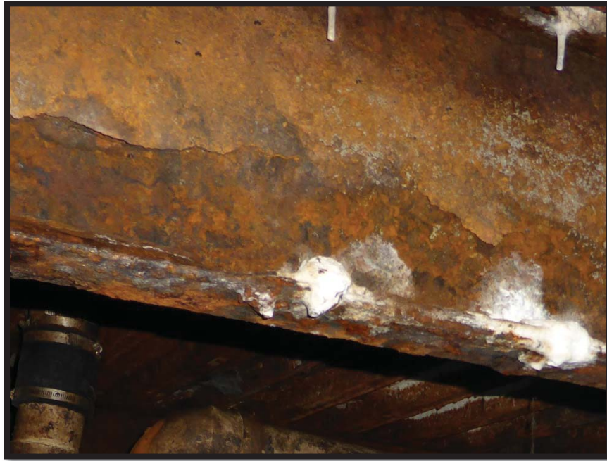
Photo 9: Severe Rust, Deterioration, and Delamination Observed on Joist Support Beam
