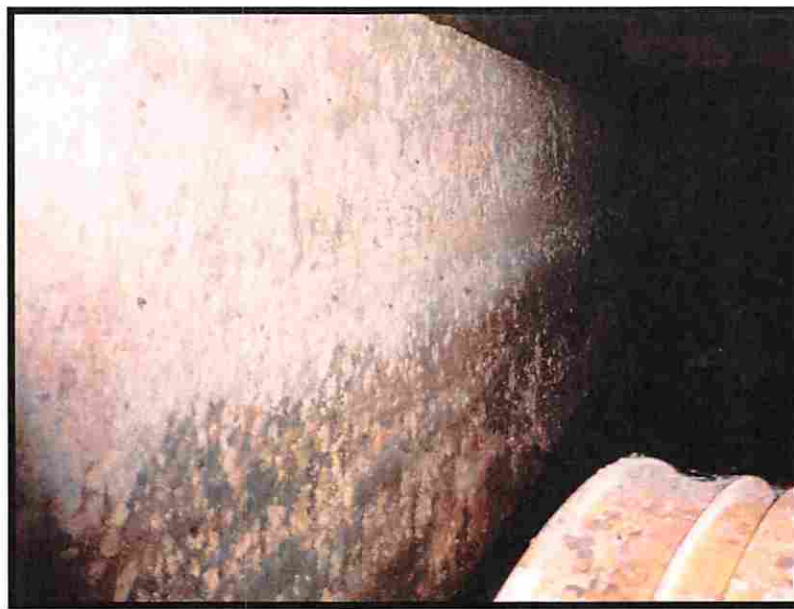
Photo 6: Evidence of Standing Water Observed on Perimeter Retaining Wall
