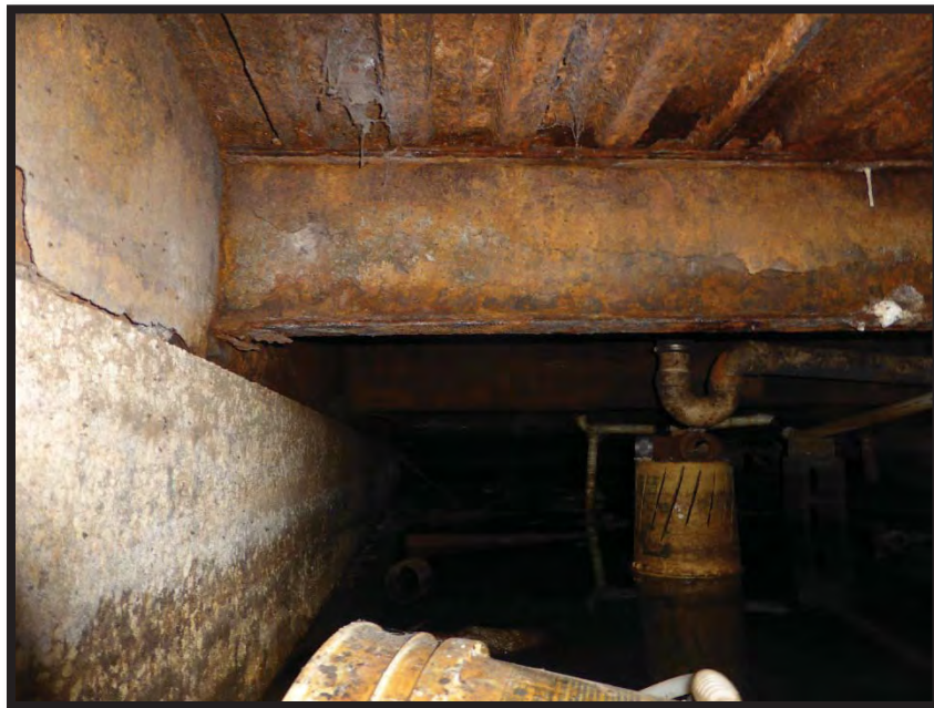
Photo 8: Severe Rust, Deterioration, and Delamination Observed on Joist Support Beams
