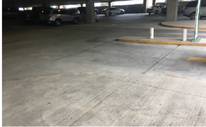
Condition on Date of Fall – September 26, 2017
