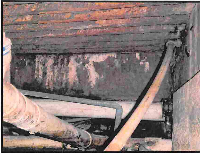
Photo 7: Rust, Deterioration, and Delamination Observed on Interior Girder Beam
