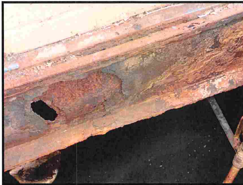
Photo 10: Severe Rust, Deterioration, and Delamination Observed on Perimeter Support Beam
