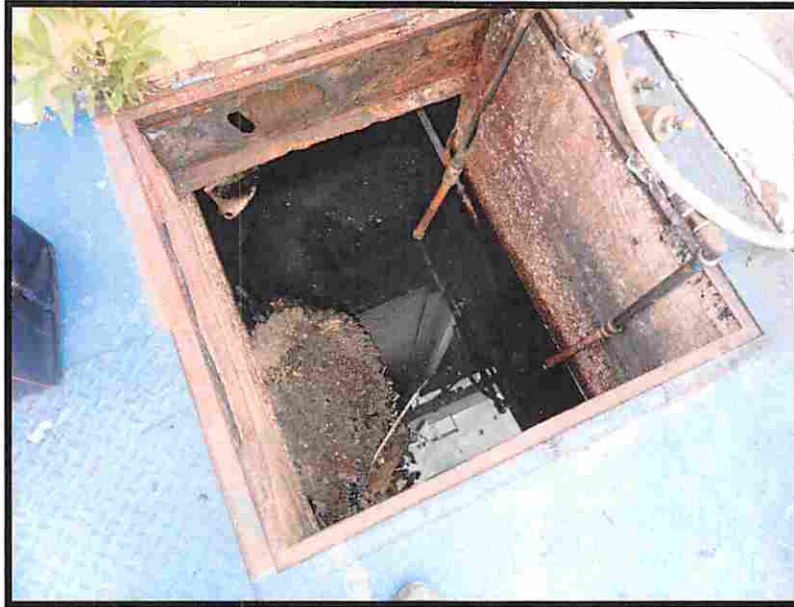
Photo 5: Standing Water at Entrance of Crawlspace
